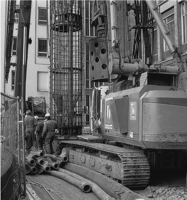
Figure 11.13 O-cell installation in 1500 mm test pile at Farringdon Station redevelopment, London. Maximum load mobilised was 80 MN. (Courtesy of Fugro Loadtest, Sunbury-upon-Thames, UK.)
