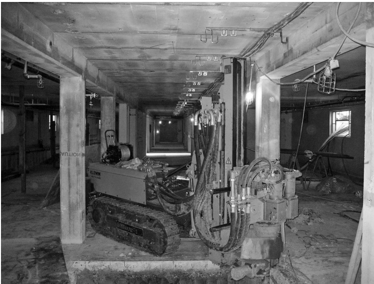
Figure 2.34 Klemm 702 restricted access drill with separate power pack installing bored piles. (Courtesy of Malcolm Drilling Company, San Francisco, CA.)
