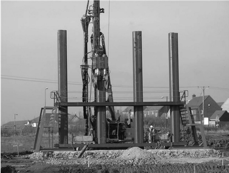
Figure 3.19 Push-pull piler installing box piles for bridge piers. (Courtesy of Dawson Construction Plant Ltd, Milton Keynes, UK.)
