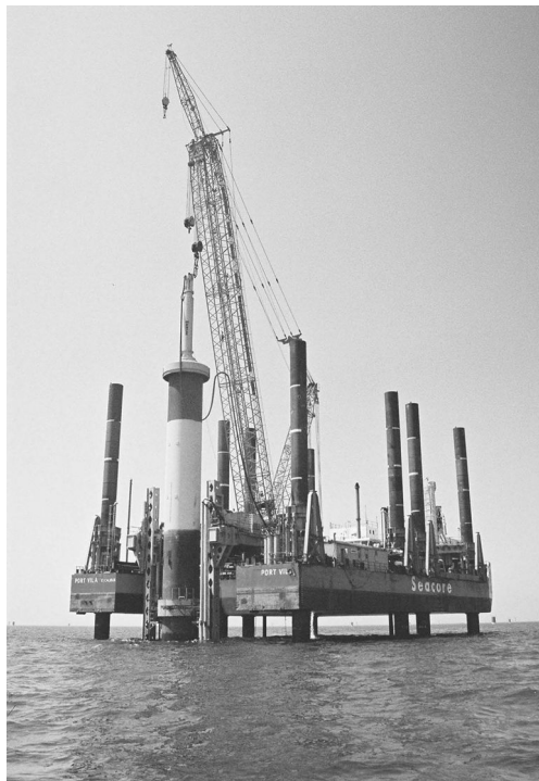
Figure 3.12 Driving a 4 m diameter monopile foundation for North Hoyle offshore wind farm using a MENCK MHU 500T hammer with large-diameter pile sleeve and anvil adapter. (Courtesy of Fugro Seacore Ltd, Falmouth, UK.)
