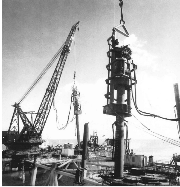
Figure 3.11 MRBS air/steam single-acting hammer with stabilising cage driving 54 in. diameter piles in legs of offshore jacket platform. (Courtesy of MENCK GmbH, Kaltenkirchen, Germany.)
