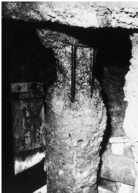
Figure 10.3 Disintegration of concrete in bored and cast-in-place pile due to attack by sulphuric acid leaking into fill from industrial processes.
