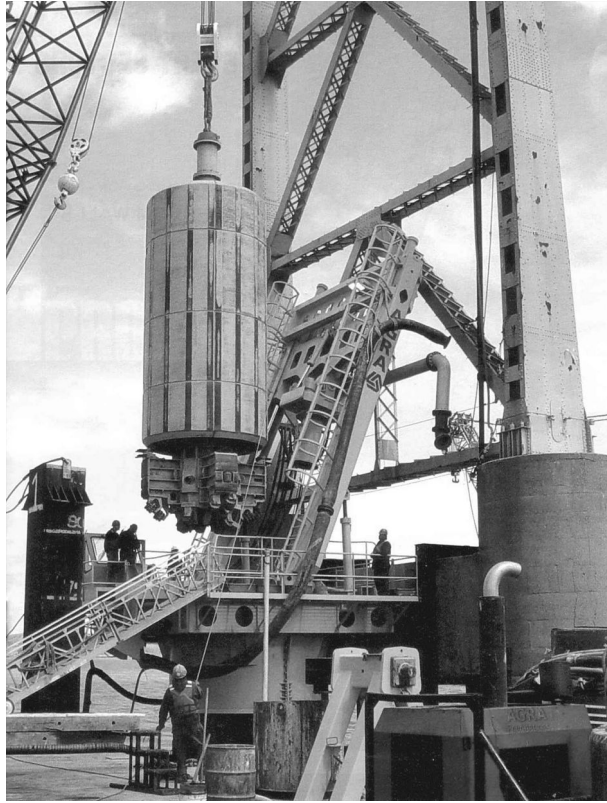
Figure 3.37 Pile-top rig drilling 3.8 m diameter piles for foundation strengthening to the Richmond-San Raphael Bridge, California. (Courtesy of Fugro Seacore Ltd, Falmouth, UK.)
