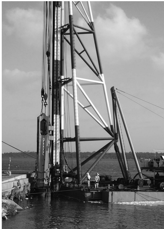
Figure 8.17 Shallow draft barge end-on to jetty driving 813 mm tubular piles in Mombasa with a CG240 hydraulic hammer. (Courtesy BSP International Foundations Ltd., Ipswich, England.)
