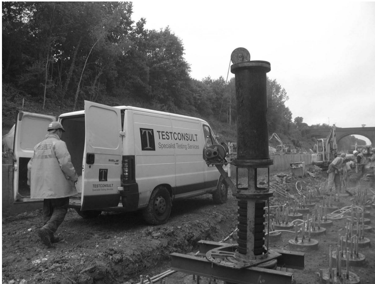
Figure 11.14 SIMBAT® test using a minirig for small-diameter dynamic tests. (Courtesy of Testconsult, Warrington, UK.)
