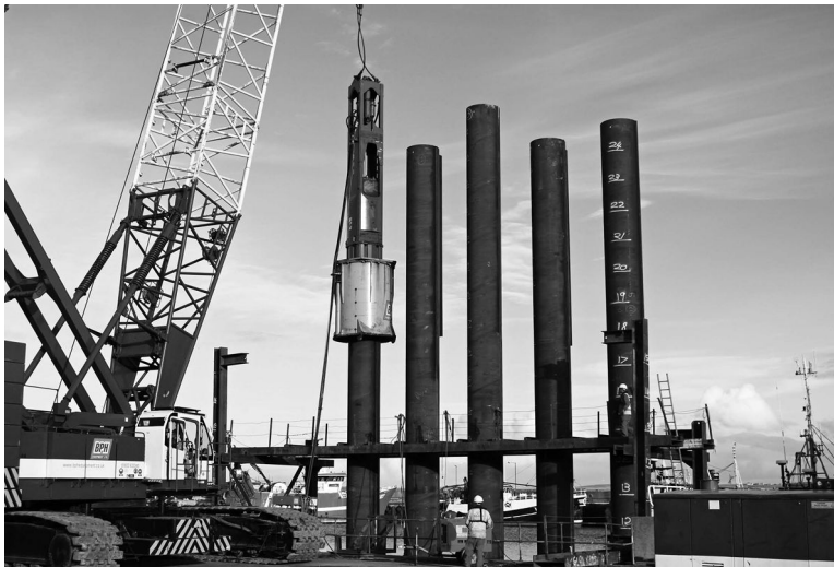
Figure 3.9 BSP CG300 hydraulic hammer suspended from a Kobelco CKEE2500 crane driving tubular piles in stages through trestle guides. (Courtesy of Steel Pile Installations Ltd, Bolton, UK.)
