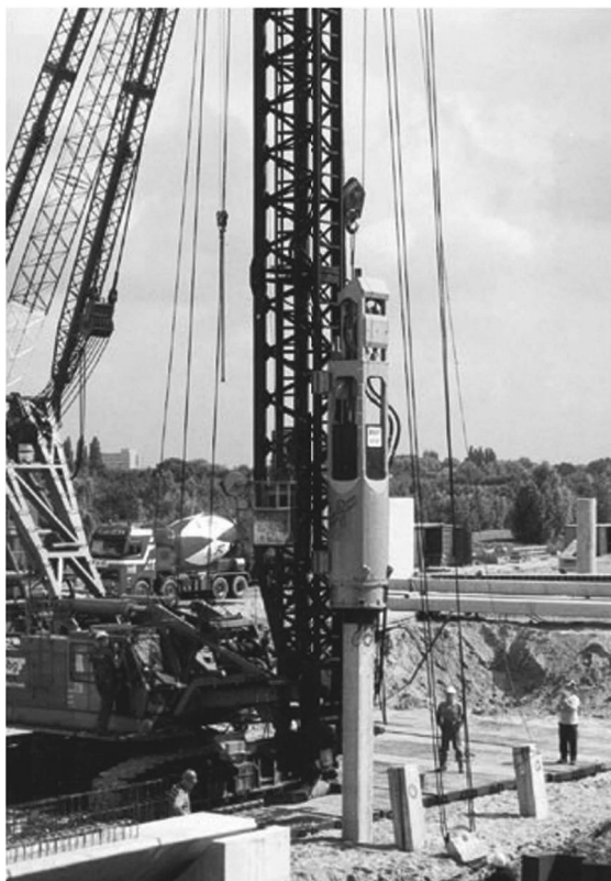
Figure 3.10 BSP CX110 hydraulic piling hammer on Hitachi crane-mounted leader. (Courtesy of BSP International Foundations Ltd, Ipswich, England.)
