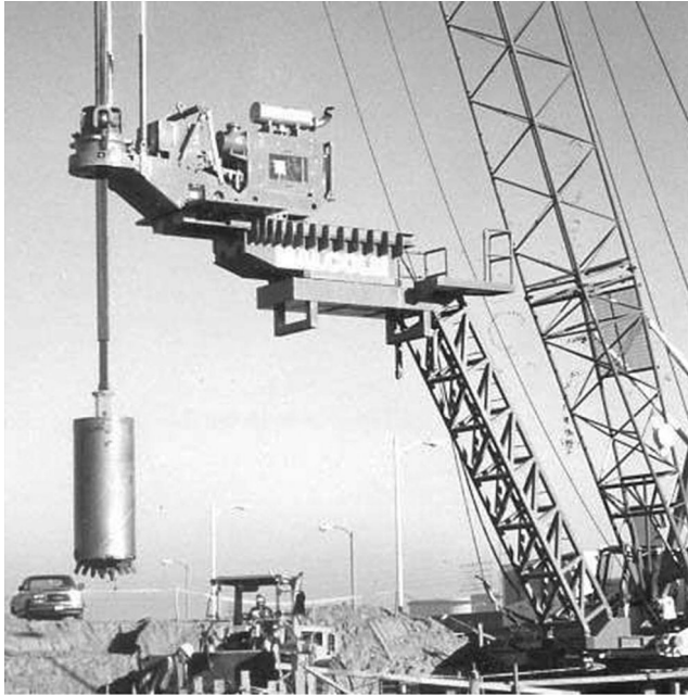
Figure 3.25 Watson 5000 crane attachment power auger on elevated platform on a 40 tonnes crane with 200 mm telescopic kelly for installing 2440 mm casings.
