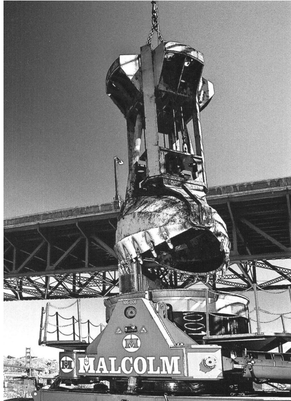
Figure 3.32 Leffer VRM 3800 casing oscillator and spherical grab installing 3.7 m diameter casings for the Doyle Drive Viaduct. (Courtesy of Malcolm Drilling Company, San Francisco, CA.)
