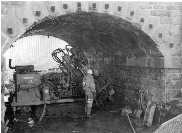
Figure 9.5 Keller piling rig installing Pali Radice piles to underpin the foundations to a rail underbridge. (Courtesy of Keller Geotechnique, Coventry, UK Tata Steel Projects. York, UK.)
