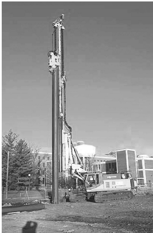
Figure 3.1 ABI Mobilram with telescopic leader fully extended driving tubular pile. (Courtesy of ABI GmbH, Niedernberg, Germany.)
