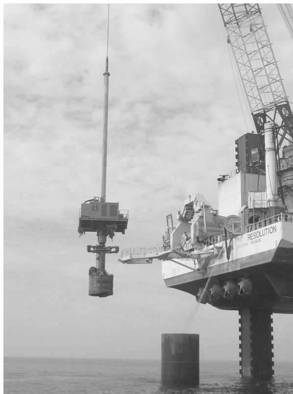
Figure 3.27 Flydrill 5500 with bucket auger removing spoil from 4.75 m diameter monopiles at the Barrow offshore wind farm site. (Courtesy of Bauer Maschinen GmbH, Schrobenhausen, Germany.)
