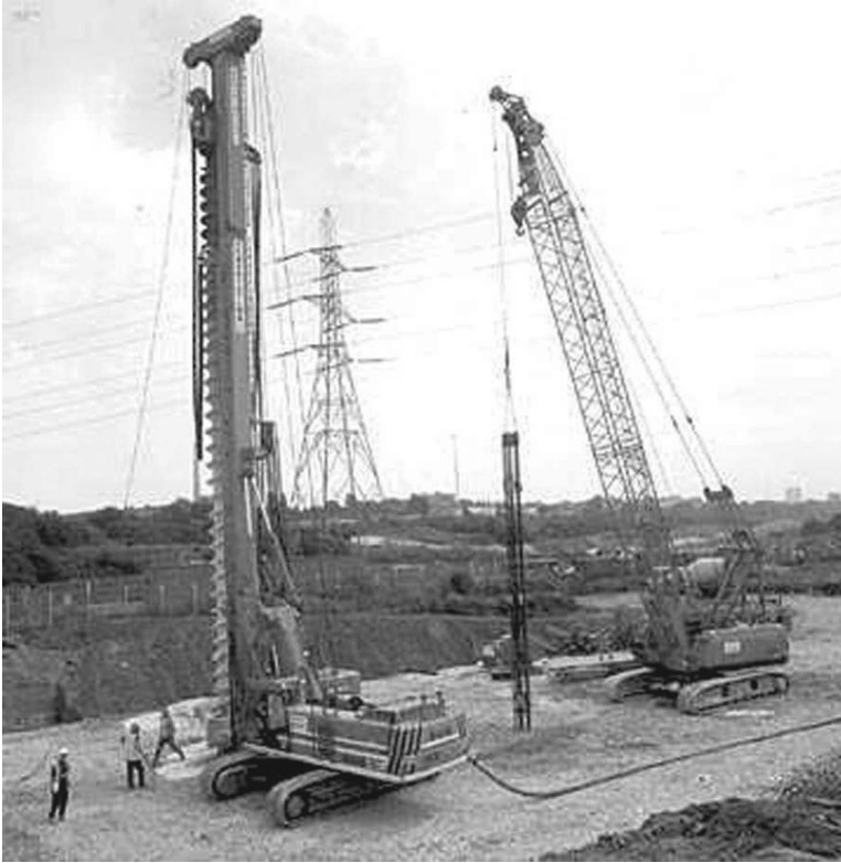
Figure 3.34 Installation of CFA piles in chalk with crane handling reinforcement cage. (Courtesy of Cementation Skanska, Rickmansworth, UK.)
