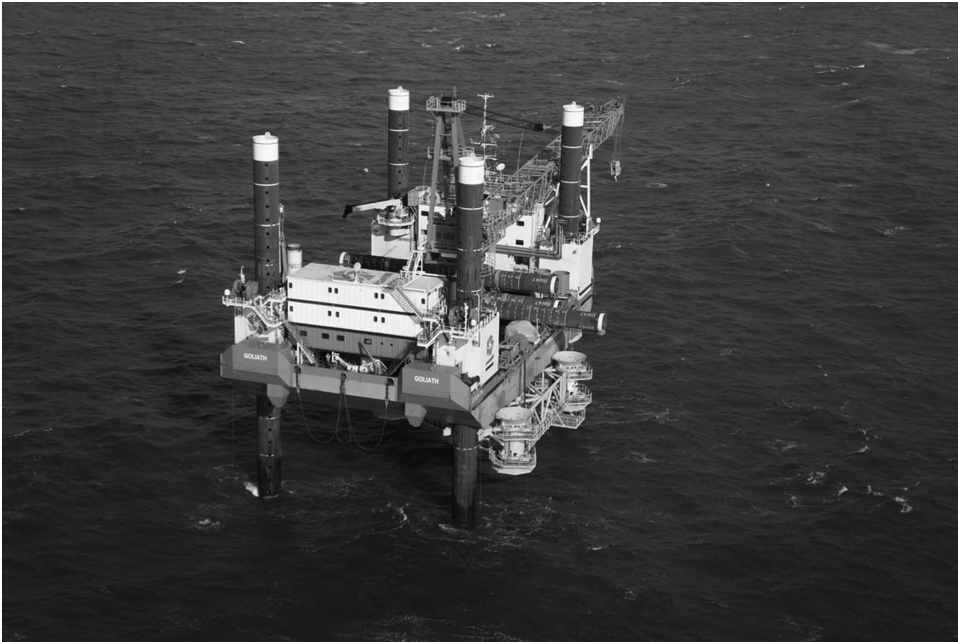
Figure 8.16 GeoSea's Goliath jack-up barge with a tripod seabed template slung ready for deployment at the Borkum wind farm in the North Sea. (Courtesy of GeoSea and DEME, Zwijndrecht, Belgium.)
