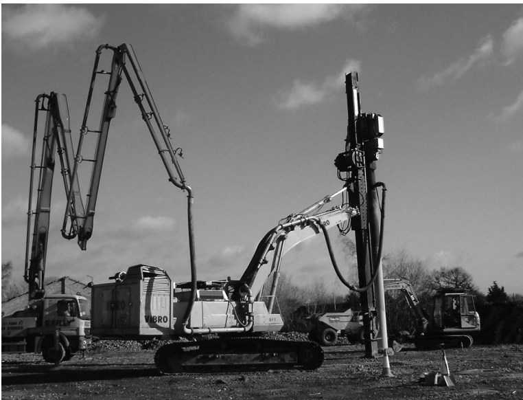
Figure 3.15 Installation of VCC showing concreting hose connected to vibrator. (Courtesy of Vibro Ménard, part of the Bachy Soletanche Group, Ormskirk, UK.)
