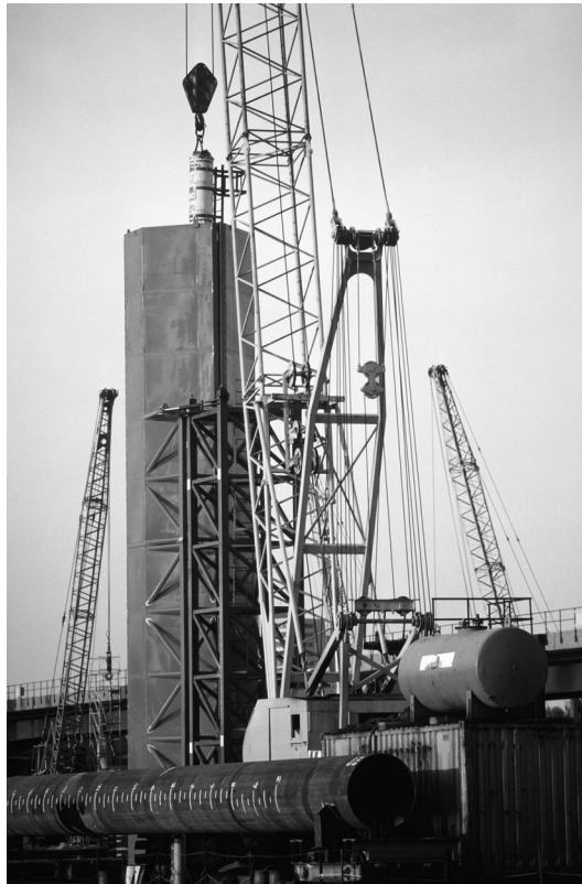
Figure 3.18 Noise suppression shroud around tubular steel pile driven by a hydraulic impact hammer.
