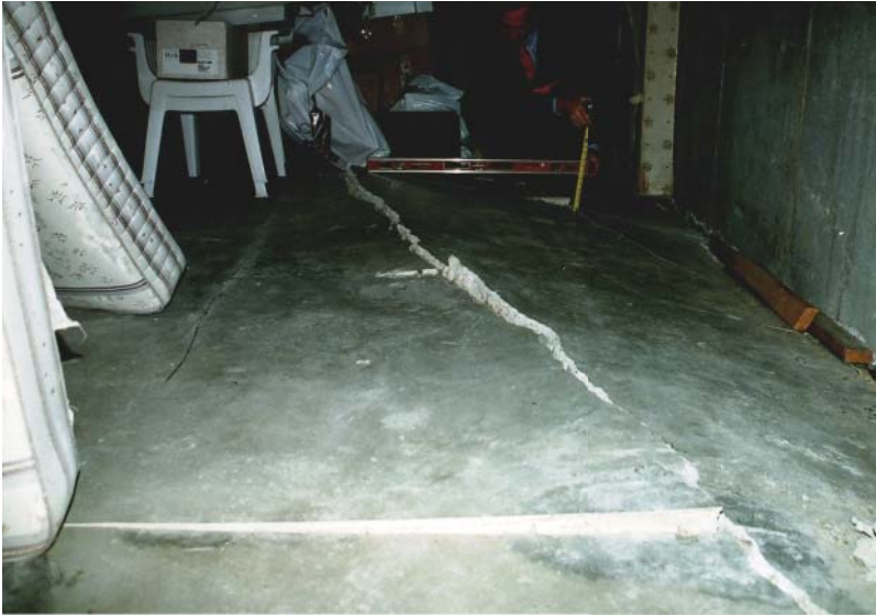
FIGURE 13.2. Slab-on-grade floor subjected to heave. Friction between the wall and the slab restricted slab movement.
