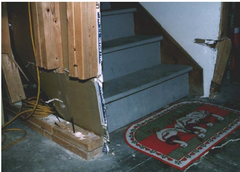
FIGURE 13.4. Closed gap of suspended non-load-bearing interior wall. Note the studs that were cut to prevent transmittal of forces to upper floors.
