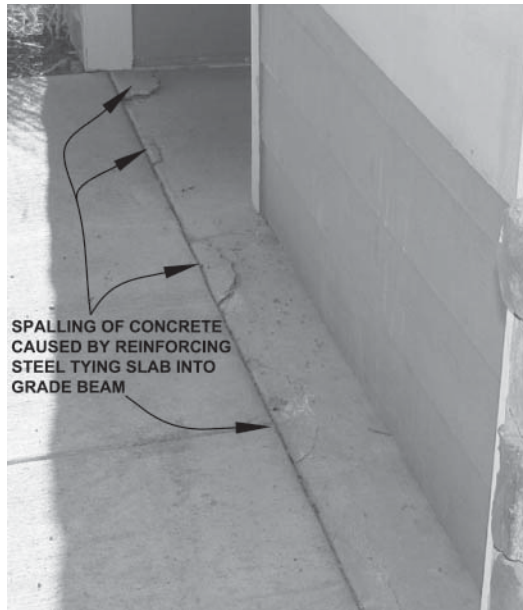
FIGURE 13.7. Damage caused by tying exterior slab into grade beam.
