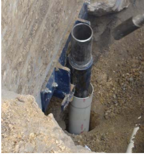
FIGURE 12.12. Micropile prior to grouting with annulus around the outside of casing (Schaut et al. 2011).
