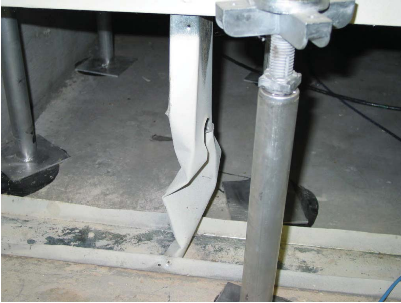
FIGURE 13.5. Steel stud buckled due to floor heave.
