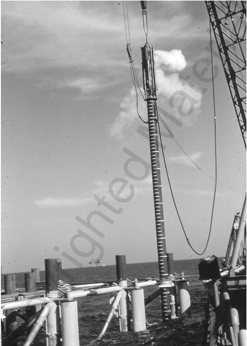
Figure 1.5 Vertical pile being driven at offshore site with a swinging steam hammer.
