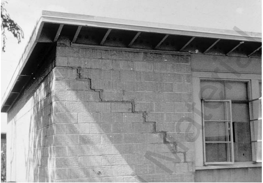
Figure 6.2 Damage to a masonry structure on expansive clay.
