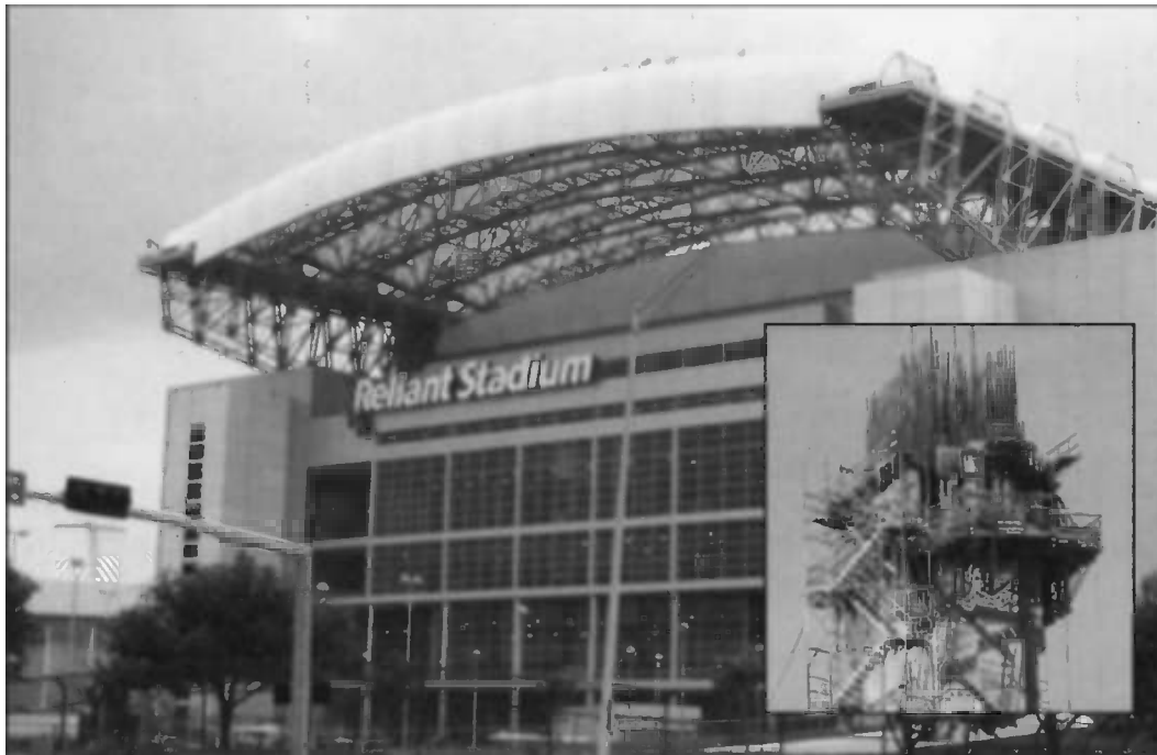
Fig. 20 —Reliant Stadium in Houston, home of the NFL Texans, utilized a high-performance ternary mixture of portland and slag cements and Class C fly ash in the four massive “super columns” that support the retractable roof (inset). The concrete met the requirements of high strength (13 000 psi), low heat (massive placement), and virtually self-consolidating consistency.
