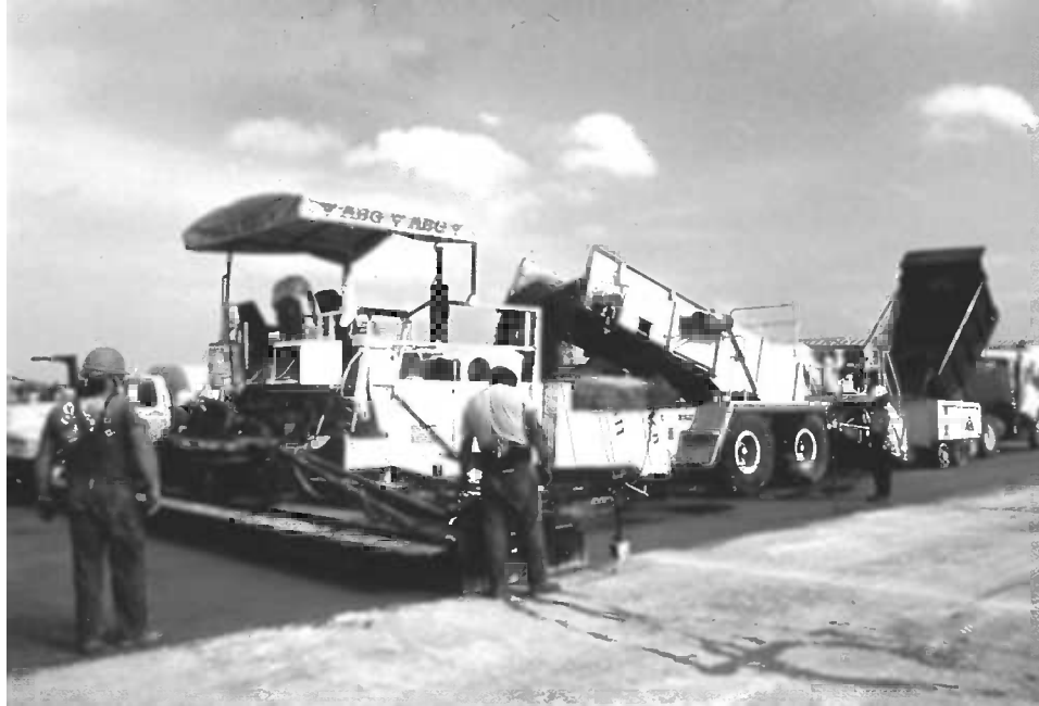
Fig. 2 —RCC being placed with heavy-duty paver. Intermediate transfer device used to maintain a constant flow of material to the paver.
