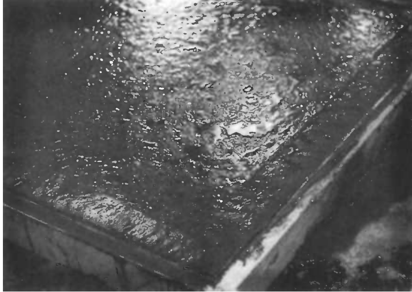
Fig. 1—Bleed water on the surface of a freshly placed concrete slab.
