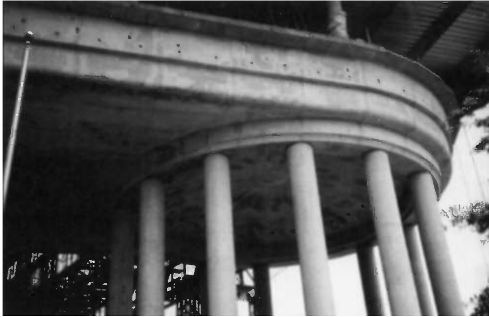
Fig. 19 —Greening is evident after forms were removed from the Canadian Embassy in Washington, DC. Greening disappeared after several weeks resulting in the desired light concrete appearance of slag cement concrete (see Fig. 17).
