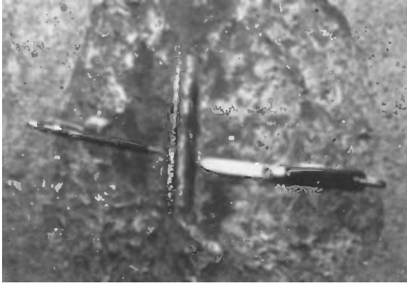
Fig. 3 —Concrete spall over a reinforcing bar in a parking garage floor.
