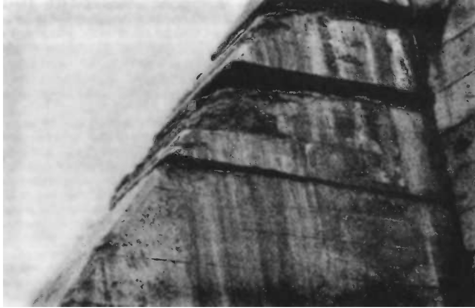
Fig. 16 —Deterioration at top of lifts in a dam from which the porous-nondurable concrete was not adequately removed prior to sequential lift placement. The poor quality concrete at the lift surface was caused by excessive bleeding and deteriorated due to frost action.
