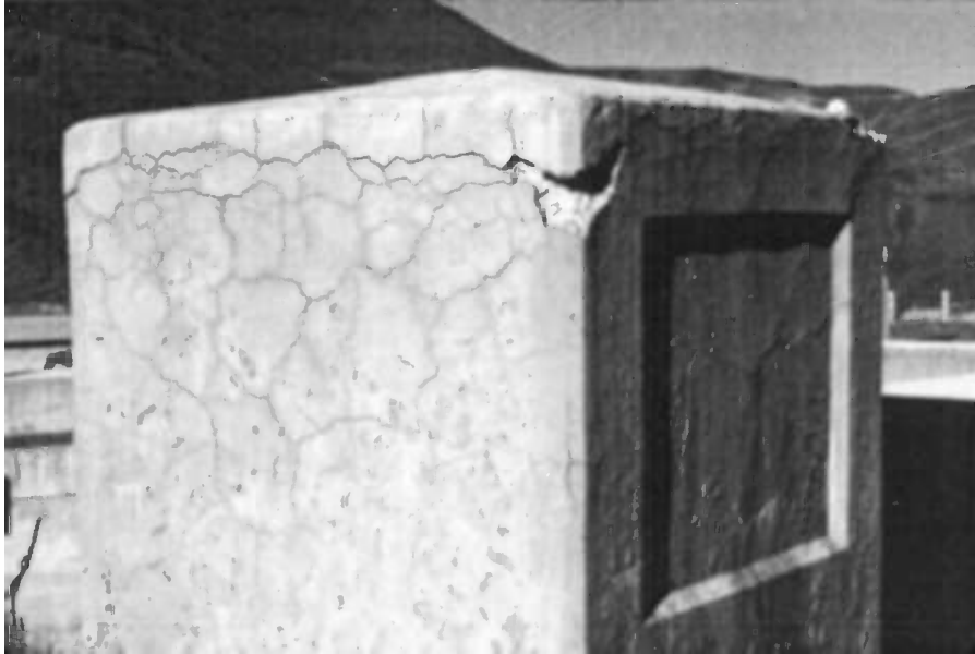
Fig. 1 —Fine pattern or random cracking initiated by ASR in a parapet wall of a dam. There is little, if any, cracking relating to differential restraint to expansion. It may be somewhat accentuated by drying shrinkage.
