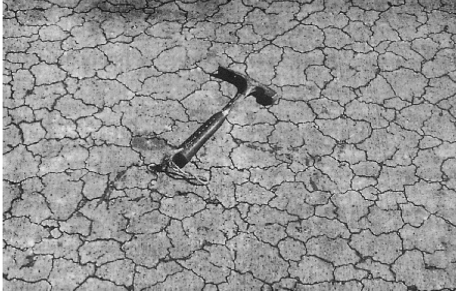
Fig. 1 —Typical cracking of concrete slab by alkali-carbonate reaction after three years, Ontario, Canada [7].
