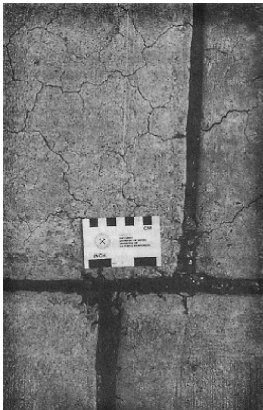
Fig. 2 —Concrete slab affected by alkali-carbonate reaction (upper portion of photo) that has moved 9 cm to the right relative to the concrete in the lower portion of the photo that has nonreactive aggregate. Expansion was measured at 1.2 % in three years, Ontario, Canada [48].
