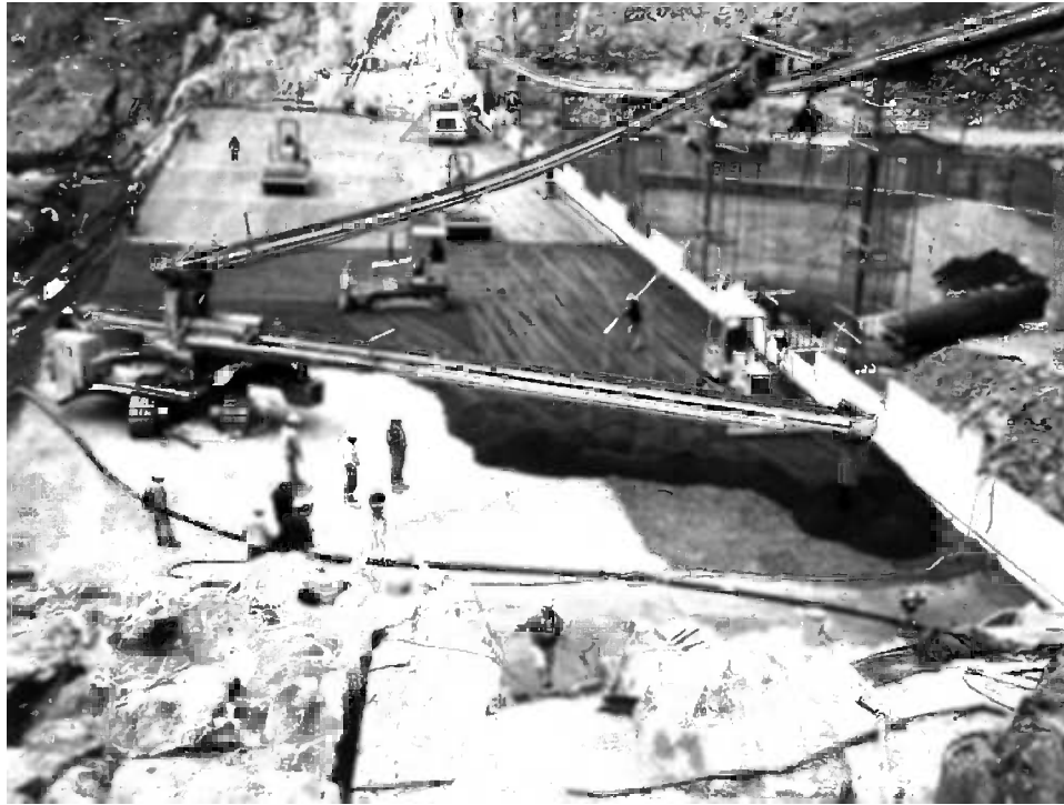
Fig. 1 —Construction of C. E. Siegrist Dam, PA. Note use of conveyors to place roller-compacted concrete (photo courtesy of Gannett Fleming).
