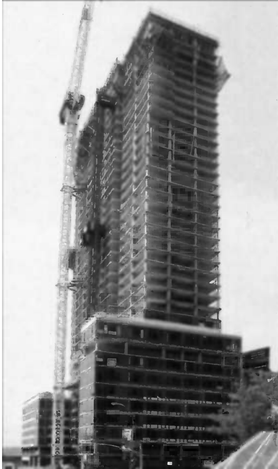
Fig. 21 —Forty-five percent slag cement concrete was used in the structural concrete in The Helena, in Manhattan, to help gain green building certification and a New York State tax incentive for green building construction. Two-day forming cycle was not affected by the use of slag cement, even though much of the construction occurred during the winter.
