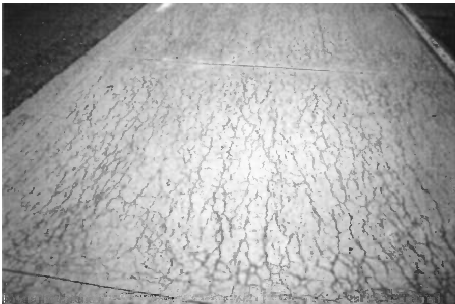
Fig. 2 —Longitudinal cracking initiated by ASR in a jointed, slab-on-grade pavement. A longitudinal crack pattern prevails in this pavement, together with minor random cracking, particularly near transverse joints.
