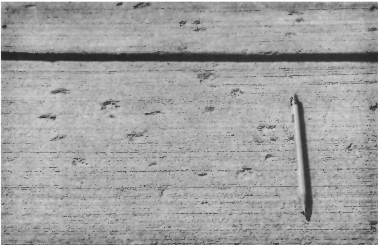
Fig. 19—Mortar flaking over coarse aggregate (photo courtesy of the Portland Cement Association).
