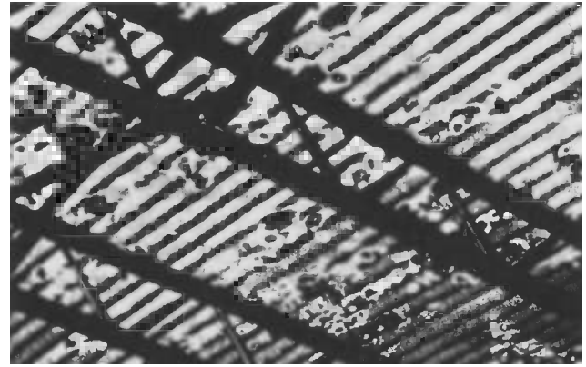
Fig. 3—Corrosion and perforation of galvanized steel from under concrete slab (from Ref 11).
