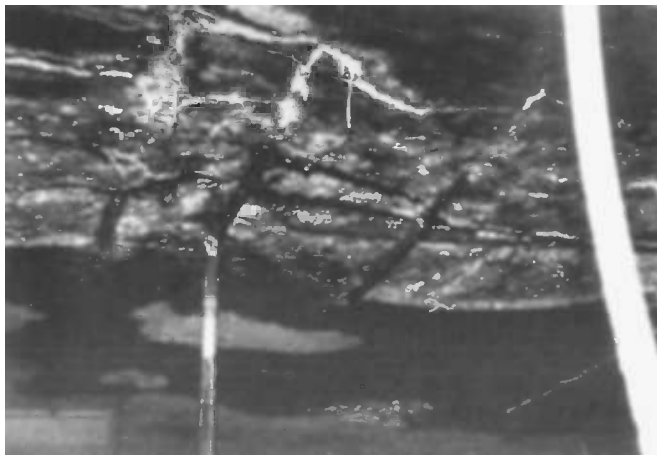
Fig. 4 —Severe corrosion of reinforcing steel and an embedded electrical conduit on the underside of a parking garage floor.
