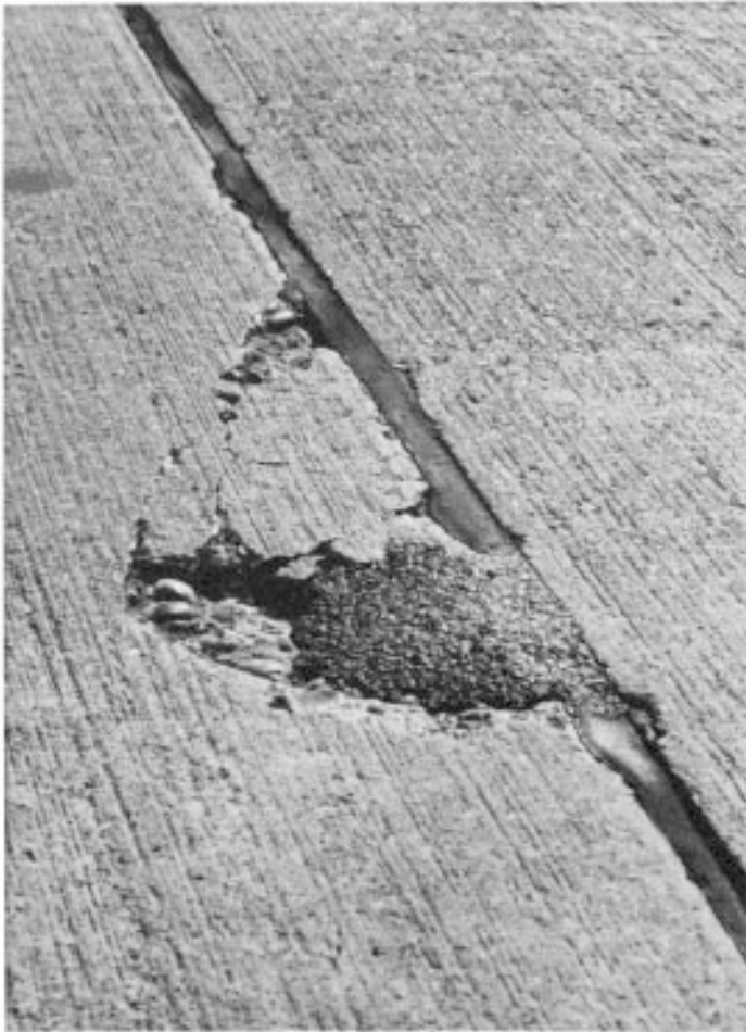
Figure 8.4 Defective joint in floor of multi-storey car park.
