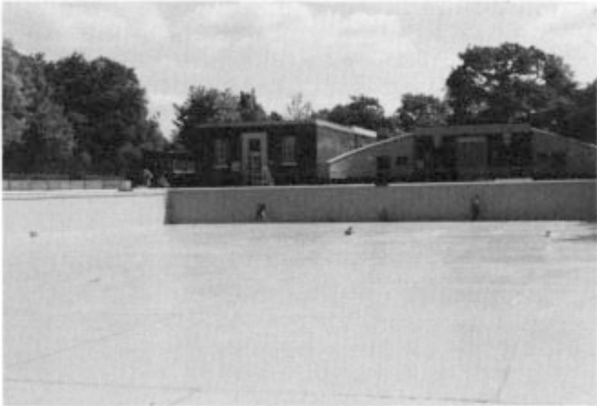
Figure 9.7 Open-air swimming pool being finished with chlorinated rubber coating after completion of repairs to joints, cracks and spalled concrete. Courtesy, Colebrand Ltd.
