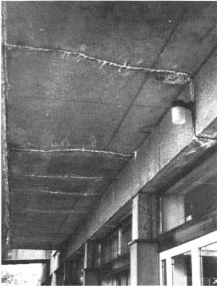
Figure 8.3 View of thermal contraction cracks in soffit of balcony slab. Courtesy, Prof. B.P.Hughes, Birmingham University.
