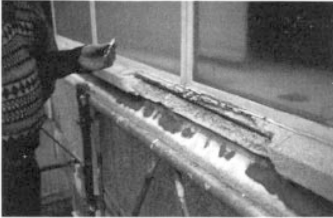
Figure 4.5 Damage to precast concrete sills caused by rebar corrosion.
