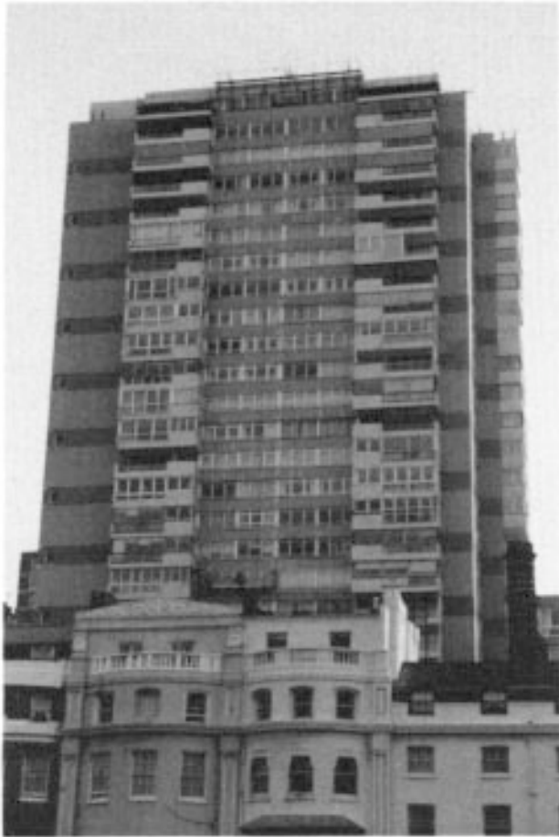
Figure 7.1 View of block of flats with defects in the concrete, and in the cement/sand rendering and in the mosaic finish. Courtesy, Gunac UK Ltd.
