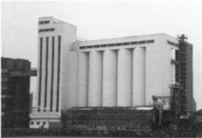
Figure 6.9 View of silos shown in Figures 6.7 and 6.8 after completion of repairs. Courtesy, Gunac UK Ltd.
