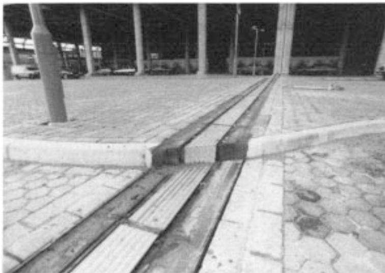
Figure 8.5 Sealed movement joint in floor of car park. Courtesy of Serviced Ltd.
