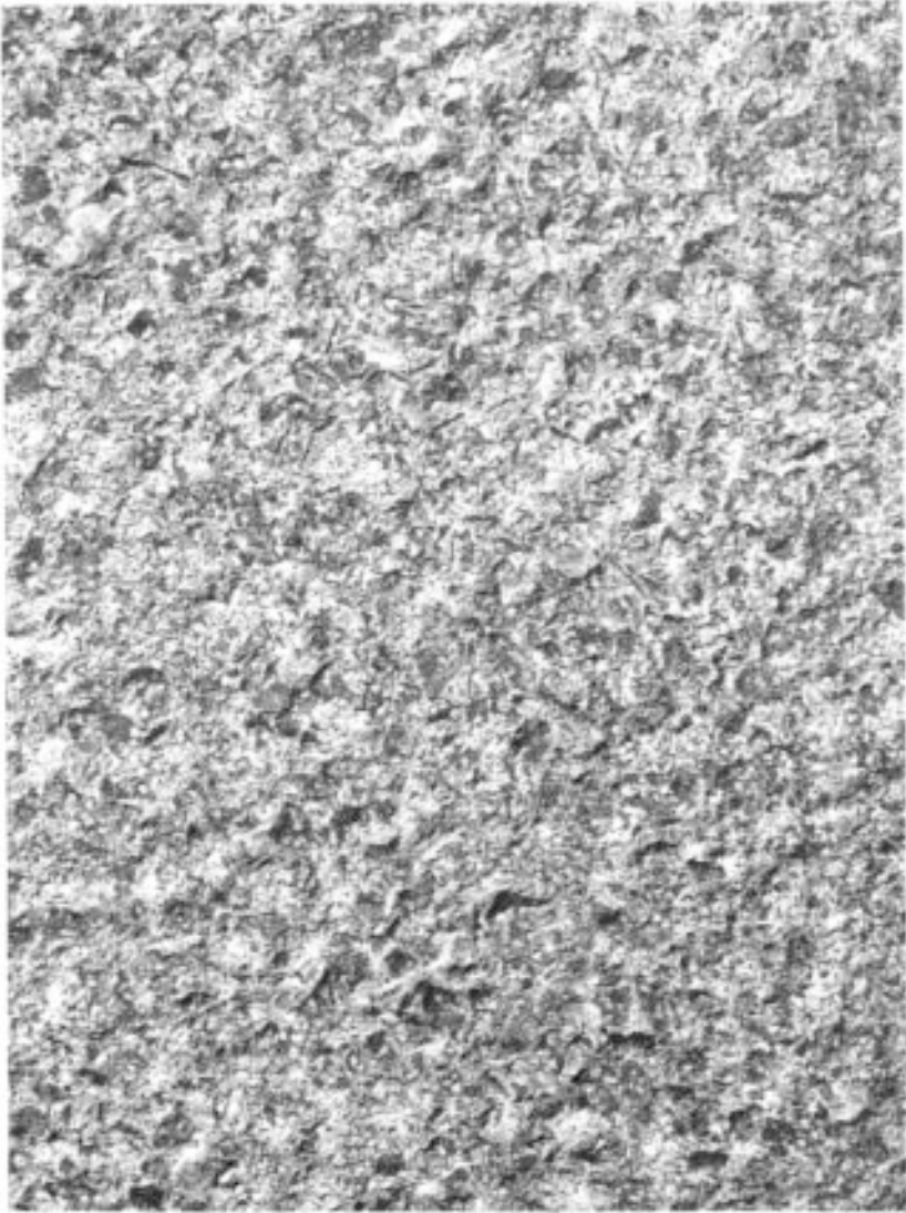
Figure 5.1 Close-up view of concrete surface prepared for application of repair mortar or concrete.
