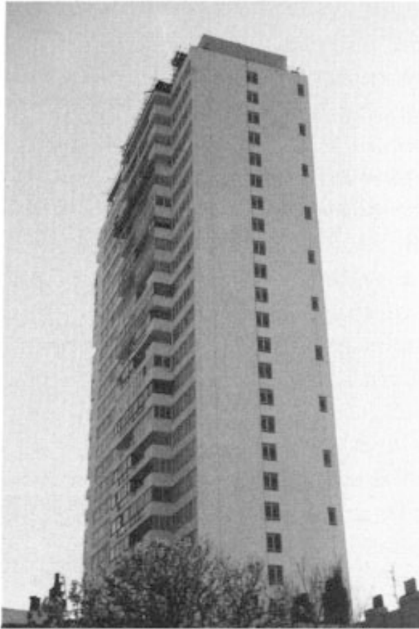
Figure 7.2 View of flats in Figure 7.1 after repair and finished with reinforced elastomeric coating. Courtesy, Gunac UK Ltd.
