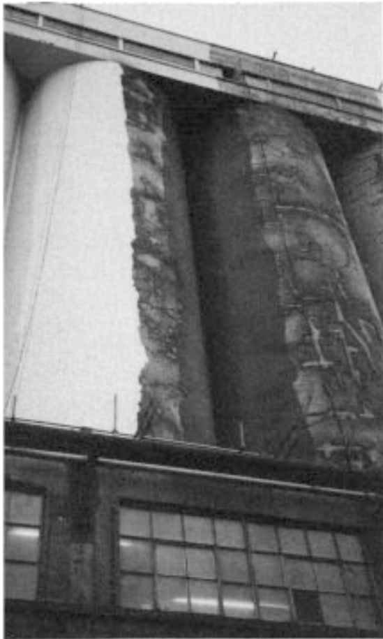
Figure 6.8 Silo in Figure 6.7 under repair showing part of final treatment with three-coat reinforced elastomeric coating. Courtesy, Gunac UK Ltd.
