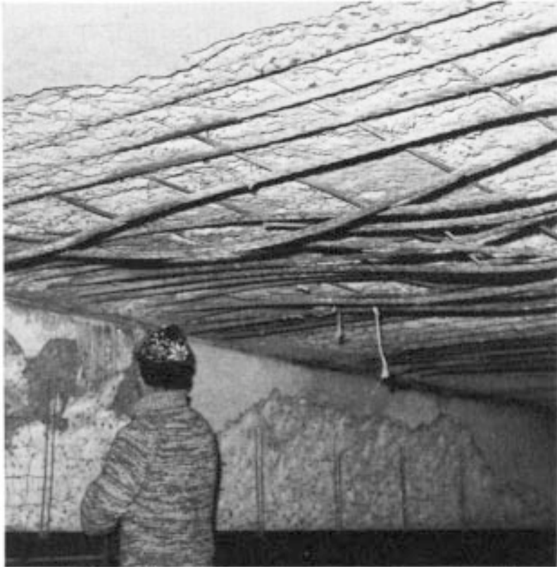
Figure 6.3 Fire damage to soffit of rc floor slab. Courtesy, Cement Gun Co. UK Ltd.
