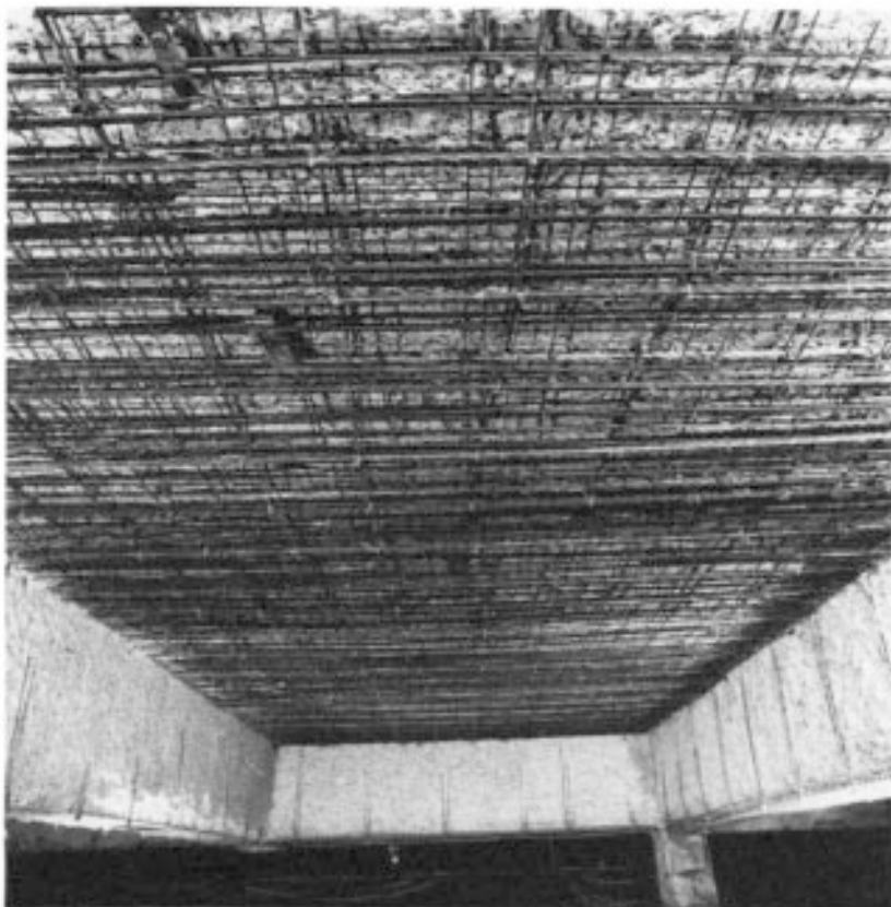
Figure 6.4 View of floor soffit in Figure 6.3 after fixing of new reinforcement prior to gunning. Courtesy, Cement Gun Co. UK Ltd.
