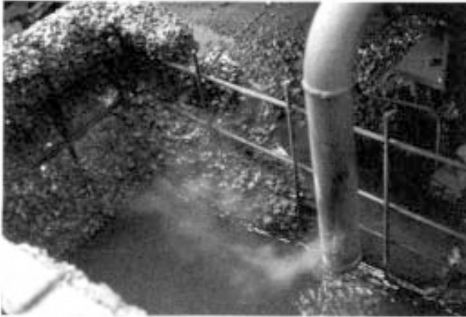
Figure 3.4 Damage to concrete by hot distilled water. Courtesy, Dr D.Higgins.
