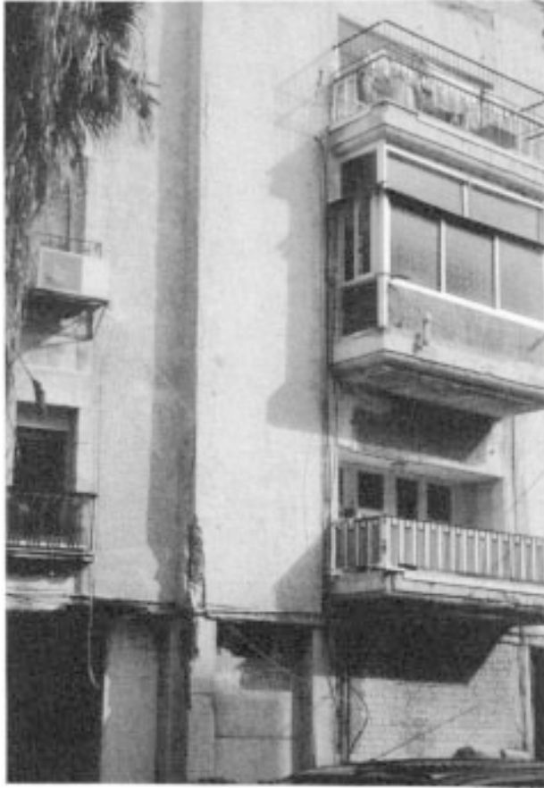
Figure 4.6 Cracking and spalling at arris initiated by careless removal of formwork.
