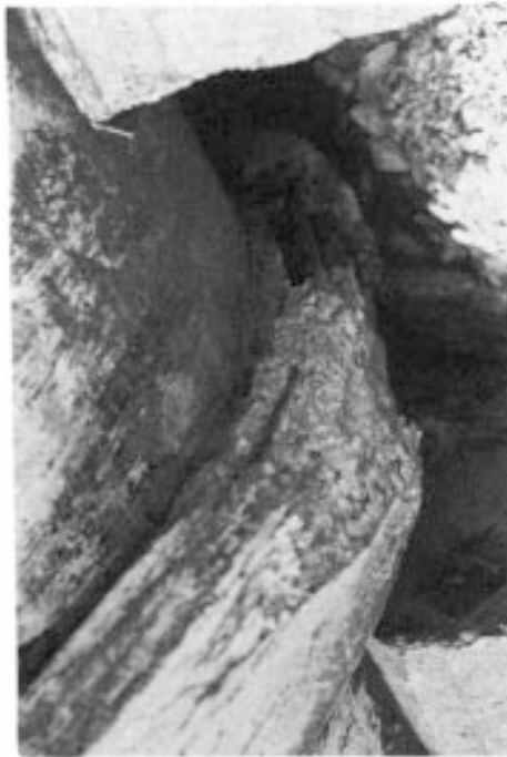
Figure 3.1 Frost damage to large-diameter concrete pipe laid above ground in the Scottish Highlands.
