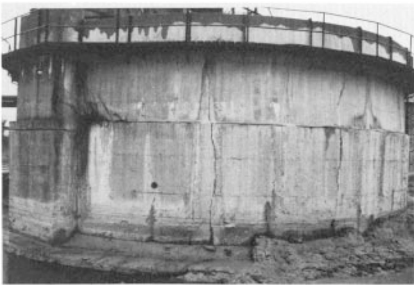
Figure 9.2 Deteriorated concrete slurry tank due to reinforcement corrosion. Courtesy, Cement Gun Co. UK Ltd.
