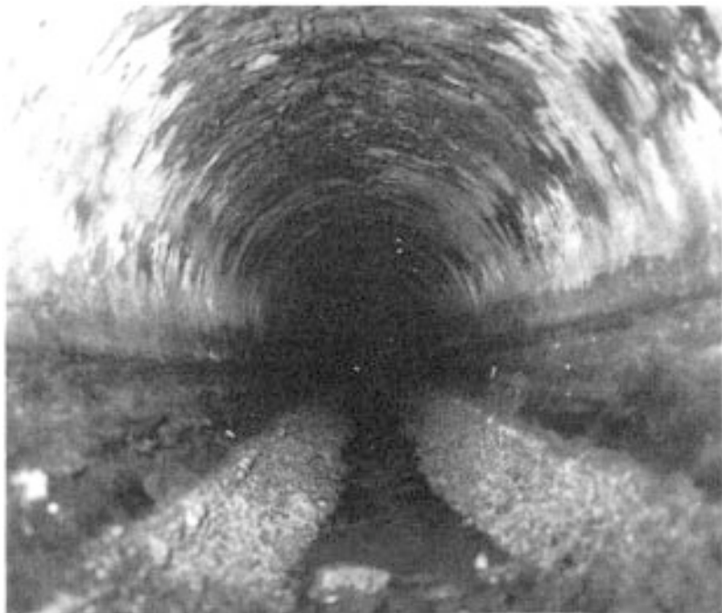
Figure 9.3 Serious attack by acidic trade effluent on concrete sewer.
