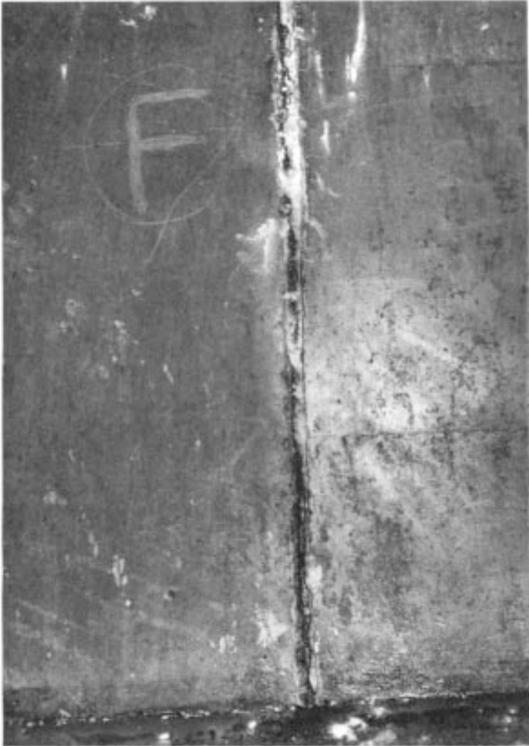
Figure 9.5 Deteriorated sealant in joint in wall of water reservoir. Courtesy, Colebrand Ltd and Thames Water Authority.
