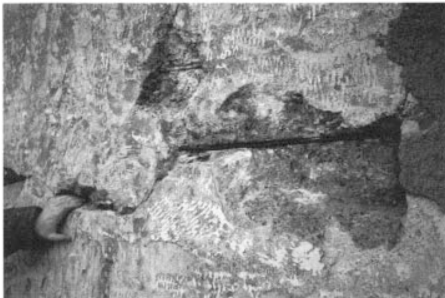
Figure 6.7 Close-up view of crack in wall of grain silo. Courtesy, Gunac UK Ltd.
