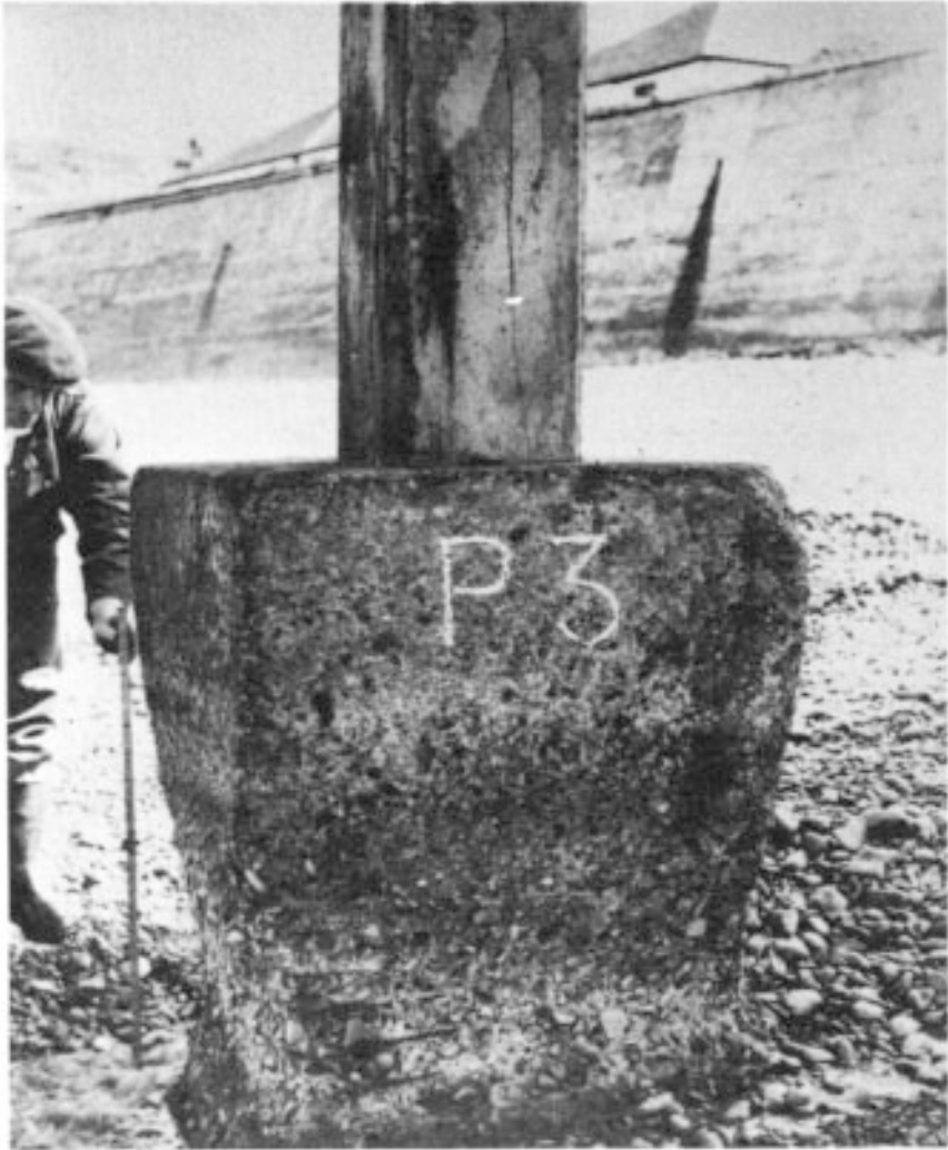
Figure 9.9 View of abrasion of concrete pier by shingle and sand.
