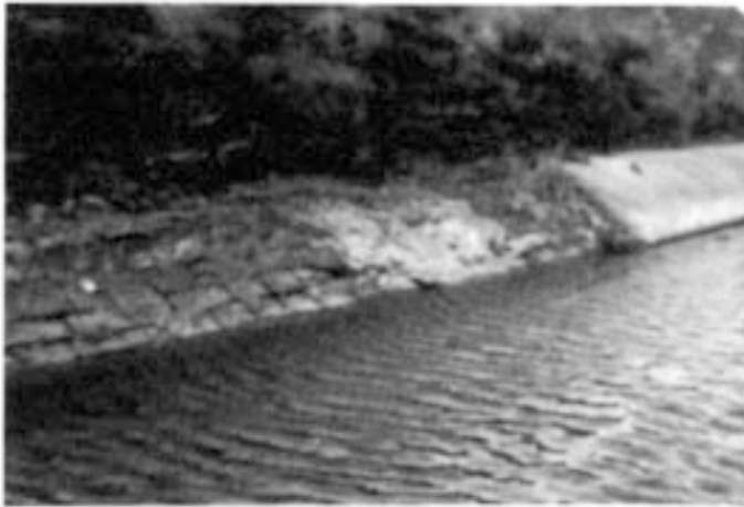
Figure 3.5 The effect of soft moorland water of low pH on concrete water channels.
