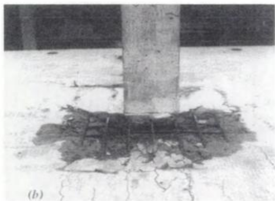
Figure 10.16 Reinforced concrete slab-column specimen transferring shear and unbalanced moment after loading 10.30 ; (a) general view; (b) failure region.
