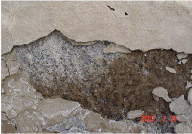
Figure 3.8 Deteriorated concrete because of sulfate attack [28].
