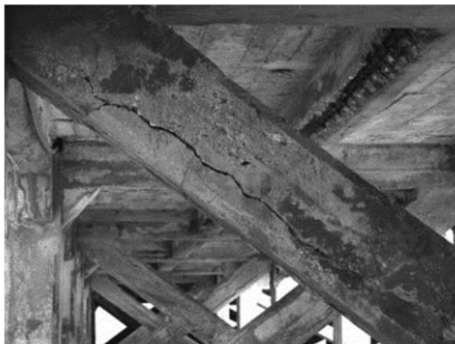
Figure 3.7 Cracking and spalling owing to corrosion in a marine environment [22].
