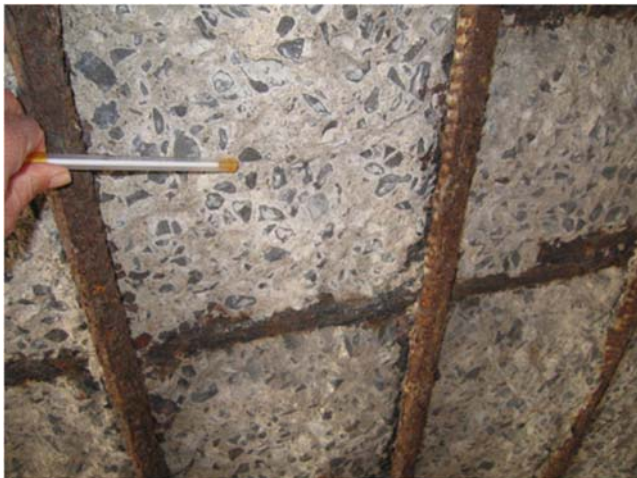
Figure 3.2 A picture of concrete damage as typical concrete durability problems from corrosion of steel bars and spalling of the concrete [4].
