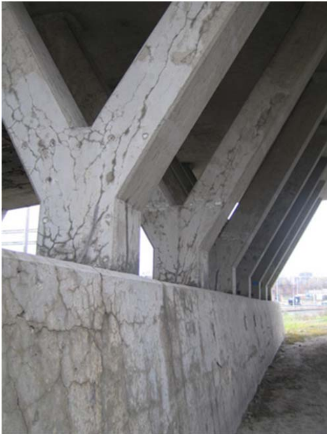
Figure 3.9 Concrete damage due alkali–aggregate reactions [4].
