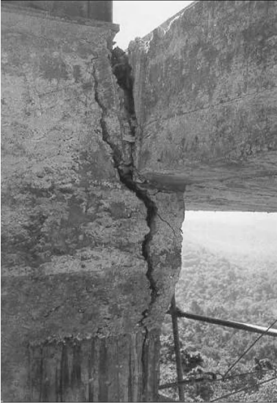
Figure 1.2 Edge beam starting to separate from column.
