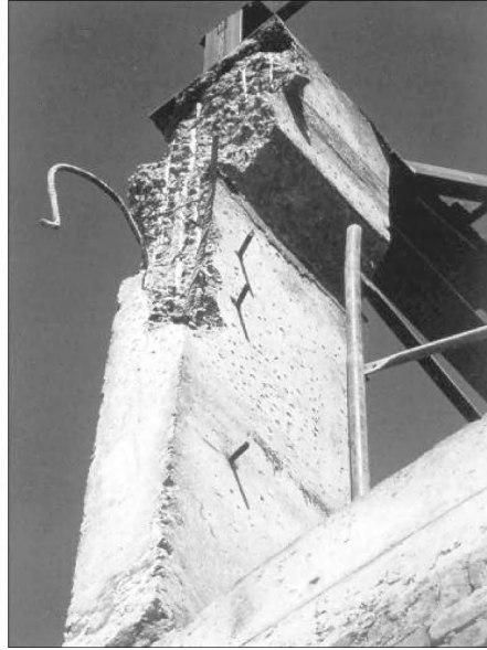
Figure 1.3 Column where edge beam has broken off.
