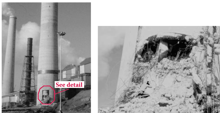
Detail: Close up of debris
