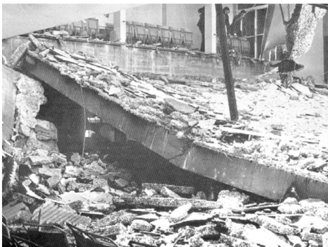
Figure 6.7 Collapsed roof lying on floor below. (From Scott, G.A., Building Disasters and Failures , Construction Press Ltd., Lancaster, 1976. With permission.)
