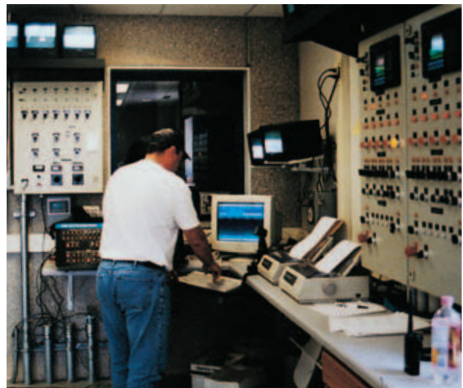
Fig. 10-1. Control room for batching equipment in a typical ready mixed concrete plant. (IMG12398)
