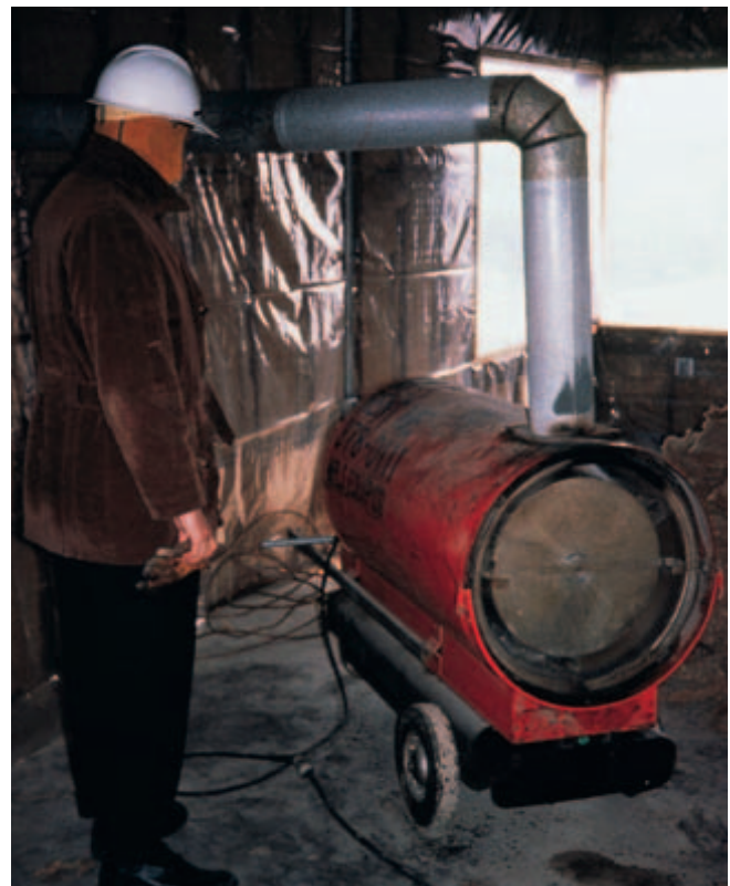
Fig. 14-23. An indirect-fired heater. Notice vent pipe that carries combustion gases outside the enclosure. (IMG12275)
