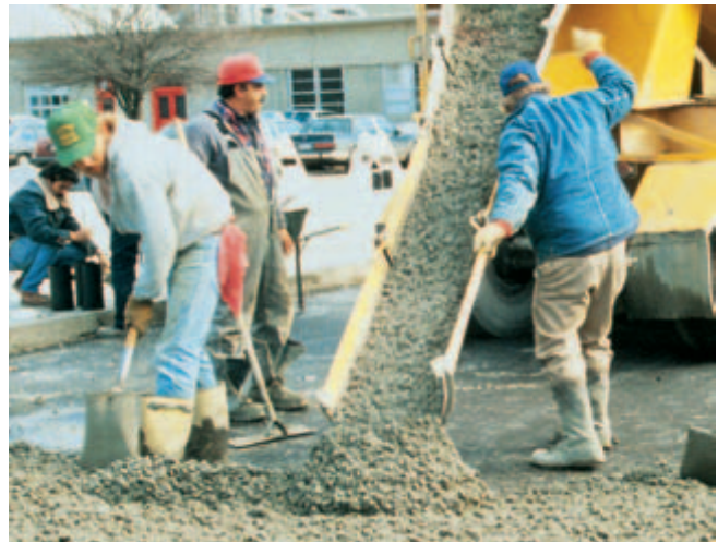
Fig. 10-10. Ready mixed concrete can often be placed in its final location by direct chute discharge from a truck mixer. (IMG12243)
