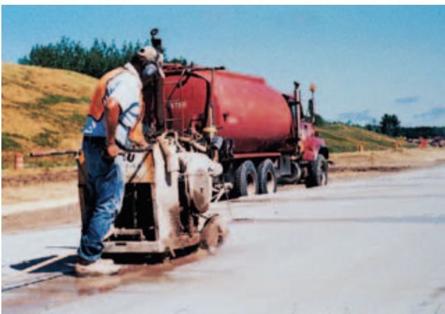
Fig. 11-28. Sawing a continuous cut in the top of a slab is one of the most economical methods for making a contraction joint. (IMG12373)
