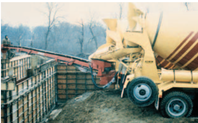
Fig. 10-14. A conveyor belt mounted on a truck mixer places concrete up to about 12 meters (40 feet) without the need for additional handling equipment. (IMG12244)
