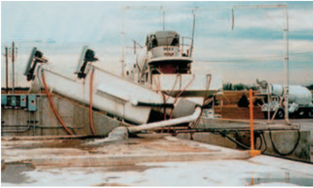
Fig. 4-4. Reclaiming system allows immediate reuse of wash water in batching. (IMG12425)
