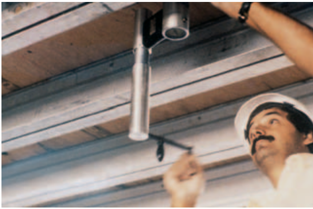
Fig. 16-23. Pullout test equipment being used to measure the in-place strength of concrete. (IMG12345)
