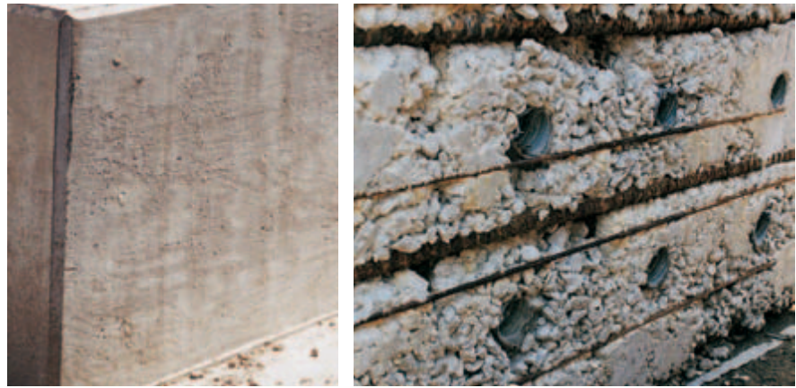
Fig. 1-8. Good consolidation (left) is needed to achieve a dense and durable concrete. Poor consolidation (right) can result in early corrosion of reinforcing steel and low compressive strength. (IMG12491, IMG12490)
