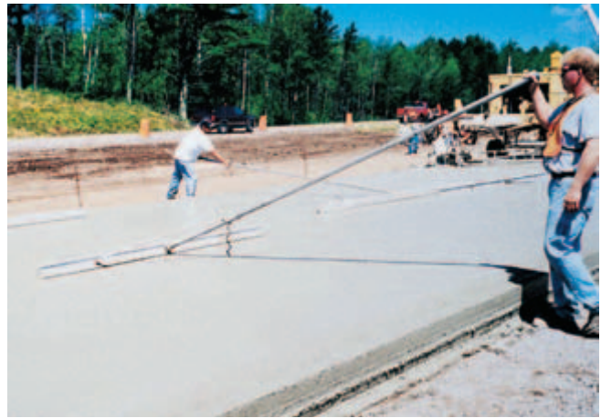
Fig. 11-17. Highway straightedges are used on highway pavement and floor construction where very flat surfaces are desired. (IMG12380)
