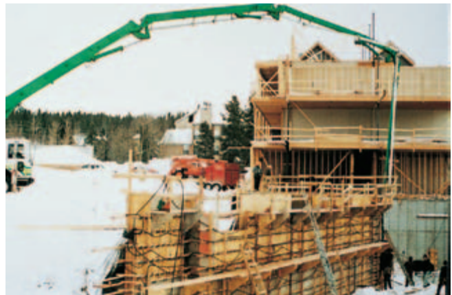
Fig. 14-25. Hydronic system showing hoses (top) laying on soil to defrost subgrade and (bottom) warming the forms while fresh concrete is pumped in. (IMG12349, IMG12348)
