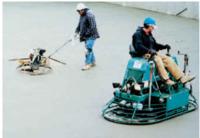
Fig. 11-18. Power floating using walk-behind and ride-on equipment. Footprints indicate proper timing. When the bleedwater sheen has evaporated and the concrete will sustain foot pressure with only slight indentation, the surface is ready for floating and final finishing operations. (IMG12379)
