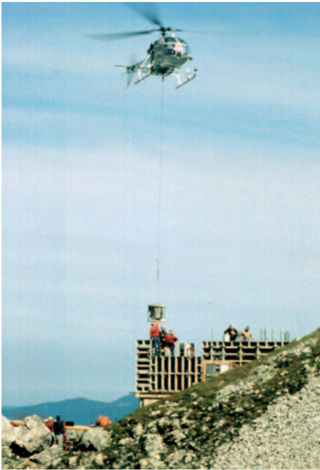
Fig. 10-17. For work aboveground or at inaccessible sites, a concrete bucket can be lifted by helicopter. (Source: Paschal)
