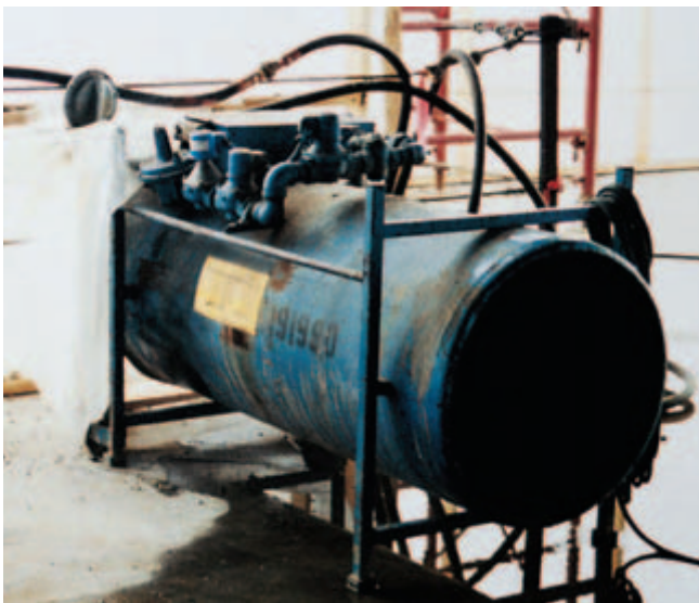
Fig. 14-24. A direct-fired heater installed through the enclosure, thus using a fresh air supply. (IMG12206)
