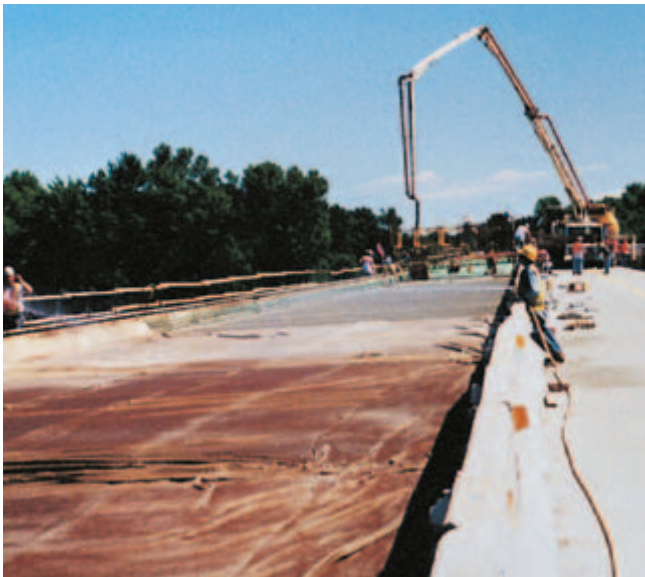
Fig. 12-1. Curing should begin as soon as the concrete stiffens enough to prevent marring or erosion of the surface. Burlap sprayed with water is an effective method for moist curing. (IMG12363)
