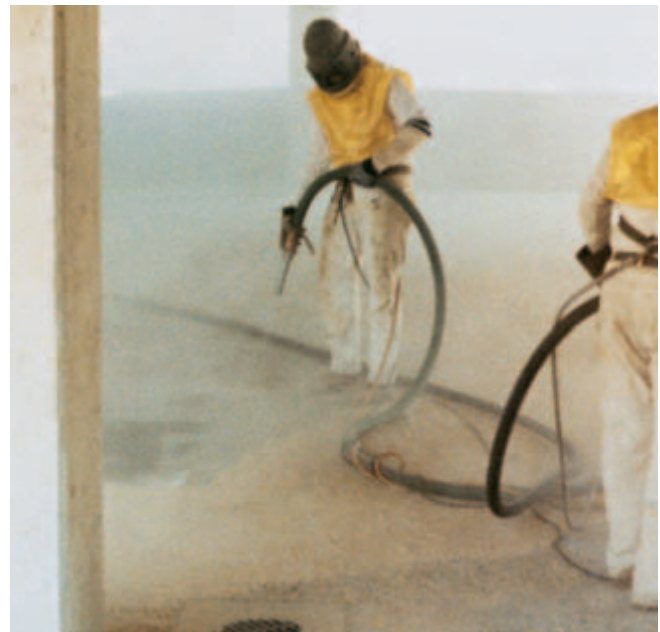
Fig. 11-23. Sandblasting can clean any size or shape surface – horizontal, vertical or overhead. Consult local environmental regulations regarding sandblasting. (IMG12252)
