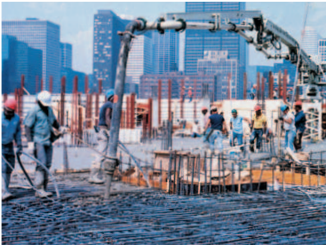
Fig. 10-18. A pump boom mounted on a mast and located near the center of a structure can frequently reach all points of placement. It is especially applicable to tall buildings where tower cranes cannot be tied up with placing concrete. Concrete is supplied to the boom through a pipeline from a ground-level pump. Concrete can be pumped hundreds of meters (feet) vertically with these pumping methods. (IMG12245)
