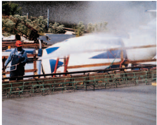
Fig. 12-4. Fogging minimizes moisture loss during and after placing and finishing of concrete. (IMG12362)
