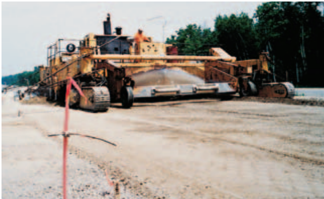
Fig. 11-1. A base course foundation for concrete pavement is shaped by an auto-trimmer to design grades, cross section and alignment by automatic sensors that follow string lines. (IMG12388)
