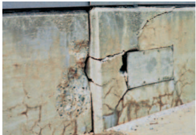
Fig. 1-27. Cracking, joint closing, spalling, and lateral offset are caused by severe alkali-silica reactivity in this parapet wall. ( IMG12295)
