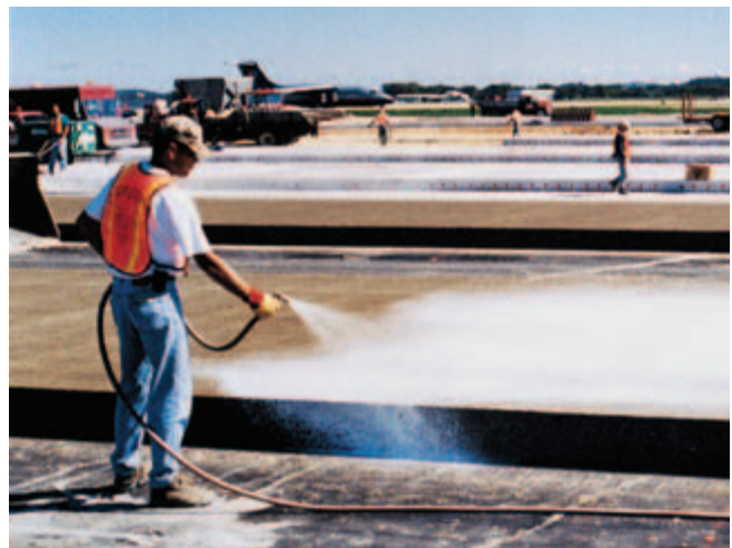
Fig. 12-8. Liquid membrane-forming curing compounds should be applied with uniform and adequate coverage over the entire surface and edges for effective, extended curing of concrete. (IMG12359)
