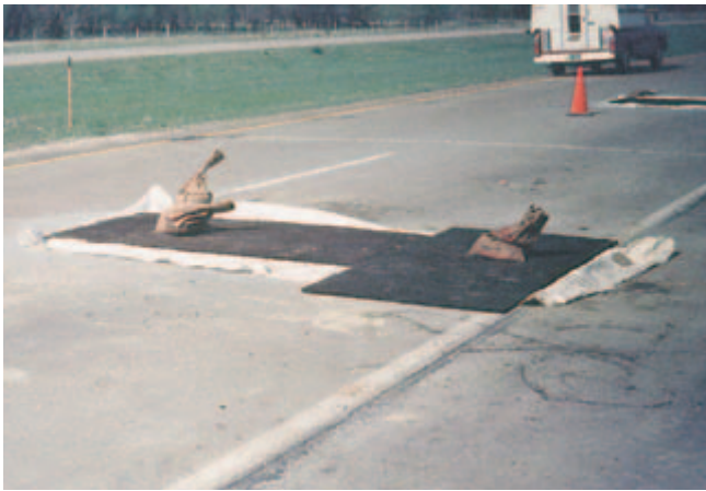
Fig. 11-34. Good curing is essential to successful patching. This patch is covered with polyethylene sheeting plus rigid insulation to retain moisture and heat for rapid hydration and strength gain. (IMG12253)
