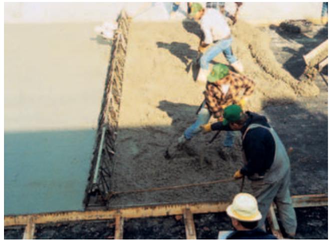
Fig. 11-12. Vibratory screeds such as this truss-type unit reduce the work of strikeoff while consolidating the concrete. (IMG12251)
