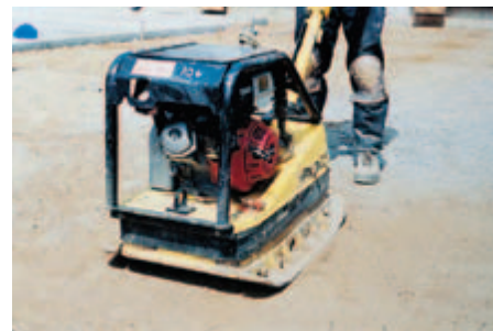
Fig. 11-3. (top) Adequate compaction of a base course foundation for concrete pavement can be achieved by using a vibratory roller. (bottom) Vibratory plate compactors are also used to prepare subgrades under slabs. (IMG12370, IMG12369)
