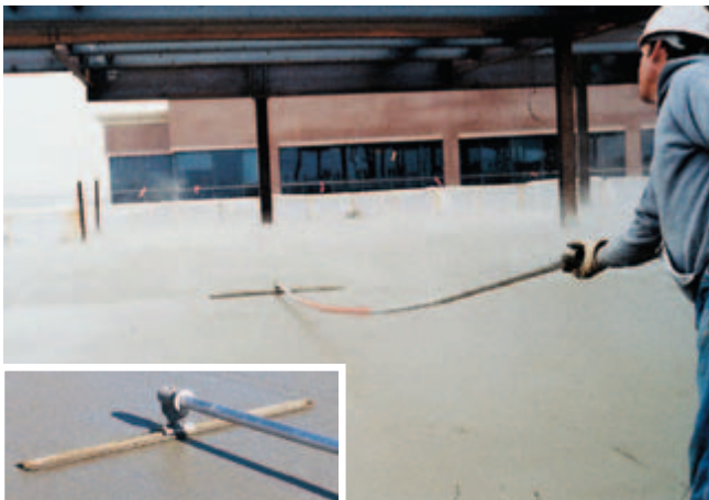
Fig. 11-16. (top) Darbying brings the surface to the specified level and is done in tight places where a bullfloat cannot reach. (bottom) Bullfloating must be completed before any bleed water accumulates on the surface. (IMG12383, IMG12382, IMG12381)
