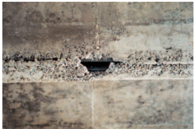
Fig. 11-9. Honeycomb and rock pockets are the results of inadequate consolidation. (IMG12262)
