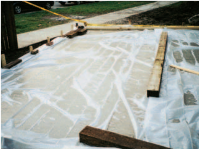
Fig. 12-7. Polyethylene film is an effective moisture barrier for curing concrete and easily applied to complex as well as simple shapes. To minimize discoloration, the film should be kept as flat as possible on the concrete surface. (IMG12360)
