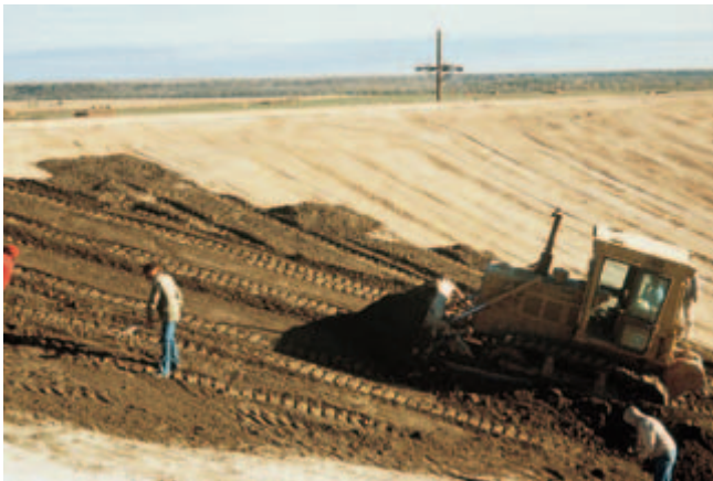
Fig. 18-12. A dozer places a plant-mixed soil-cement on a slope for construction of a wastewater lagoon. (IMG12286)
