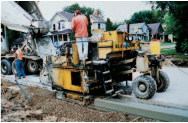
Fig. 11-7. Curb machines continuously extrude low-slump concrete into a shape that immediately stands without support of formwork. (IMG12365)
