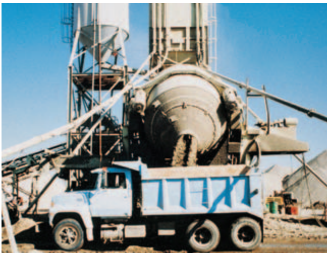
Fig. 10-2. Concrete can be mixed at the jobsite in a stationary mixer. (IMG12246)
