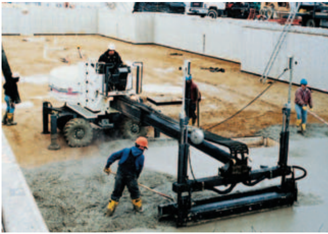
Fig. 11-14. A laser level stimulating the sensors on this screed guides the operator as he strikes off the concrete. Screed poles and chairs are not needed and fewer workers are required to place concrete. Laser screeds interfaced with total station surveying equipment can also strike off sloped concrete surfaces. (IMG12385)
