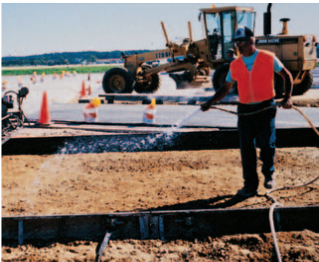
Fig. 13-9. Dampening the subgrade, yet keeping it free of standing water will lessen drying of the concrete and reduce problems from hot weather conditions. (IMG12356)
