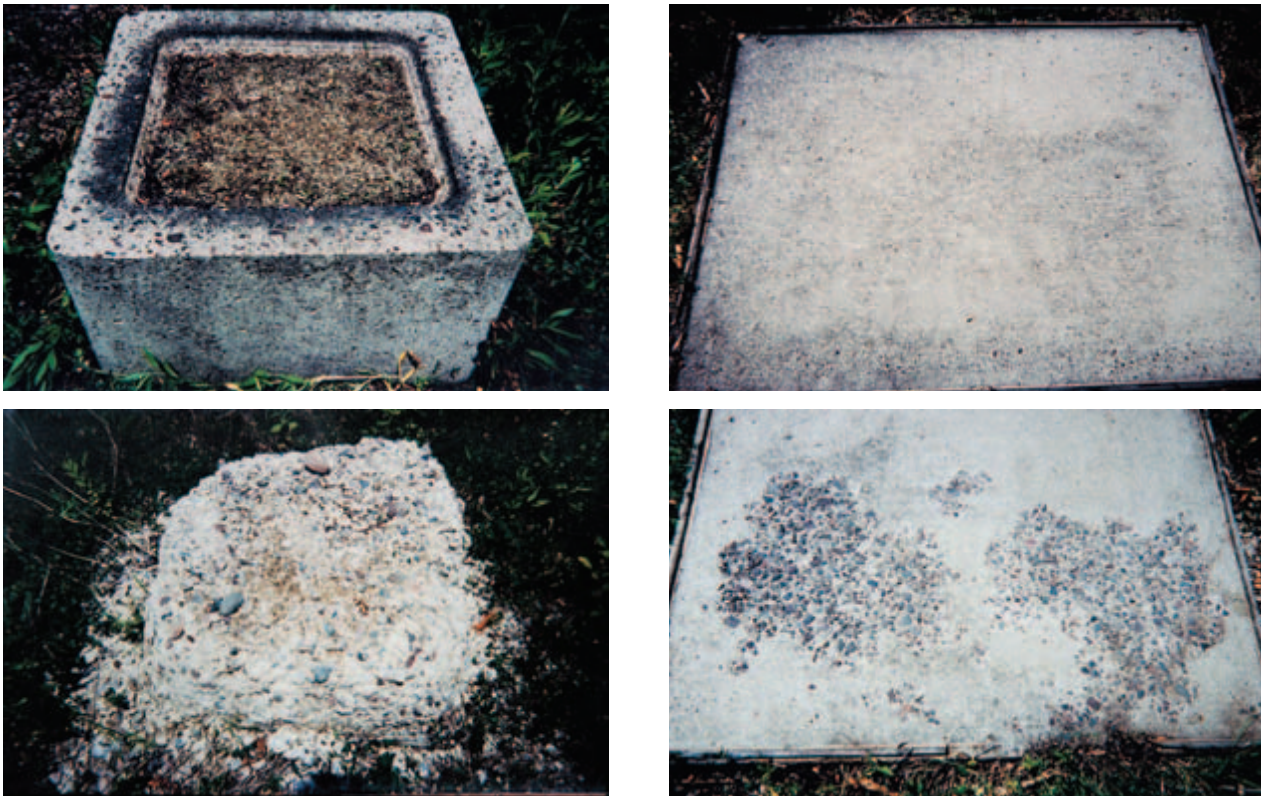
Fig. 8-3. Effect of weathering on boxes and slabs on ground at the Long-Time Study outdoor test plot, Project 10, PCA, Skokie, Illinois. Specimens at top are air-entrained, specimens at bottom exhibiting severe crumbling and scaling are non-air-entrained. All concretes were made with 335 kg (564 lb) of Type I portland cement per cubic meter (cubic yard). Periodically, calcium chloride deicer was applied to the slabs. Specimens were 40 years old when photographed (see Klieger 1963 for concrete mixture information). (IMG12408, IMG12406, IMG12407, IMG12405)
