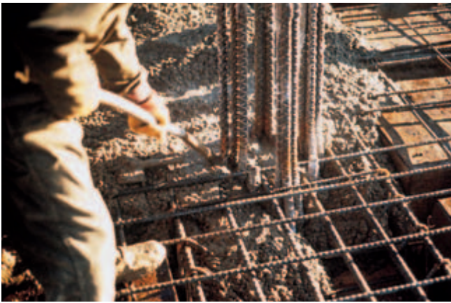
Fig. 11-10. Proper vibration makes possible the placement of stiff concrete mixtures, even in heavily-reinforced concrete members. (IMG12250)
