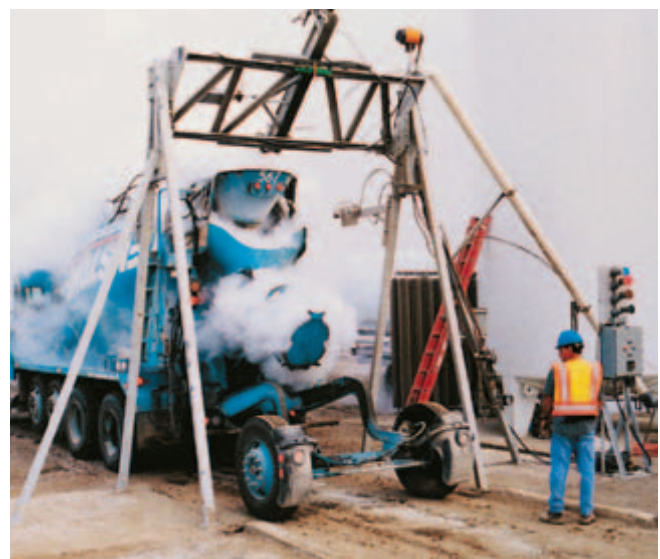
Fig. 13-1. Liquid nitrogen added directly into a truck mixer at the ready mix plant is an effective method of reducing concrete temperature for mass concrete placements or during hot-weather concreting. (IMG12357)
