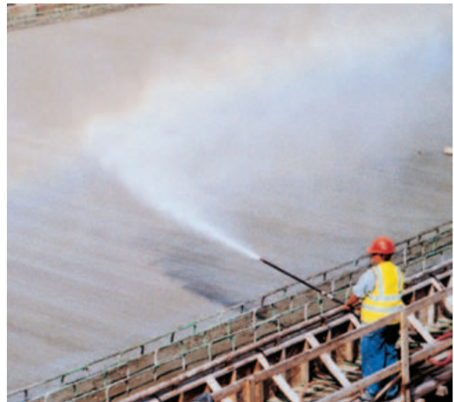
Fig. 13-11. Fogging cools the air and raises the relative humidity above flatwork to lessen rapid evaporation from the concrete surface, thus reducing cracking and improving surface durability. (IMG12355)
