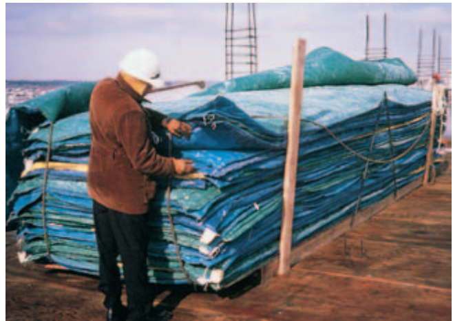
Fig. 14-19. Stack of insulating blankets. These blankets trap heat and moisture in the concrete, providing beneficial curing. (IMG12270)
