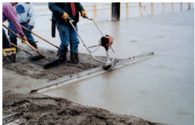
Fig. 11-13. Where floor tolerances are not critical, an experienced operator using this vibratory screed does not need screed poles supported by chairs to guide the screed. Instead, he visually matches elevations to forms or previous passes. The process is called wet screeding. (IMG12386)
