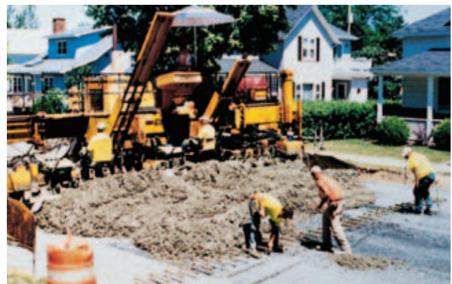
Fig. 11-6. Dump trucks deposit concrete ahead of a slip-form paver that places the entire width of a street in one pass. Epoxy coated dowels on metal chairs are positioned at a joint and spiked down to the base course just ahead of the paver. (IMG12366)
