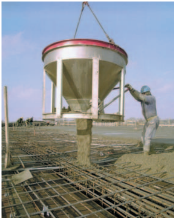
Fig. 10-9. Concrete is easily lifted to its final location by bucket and crane. (IMG12230)
