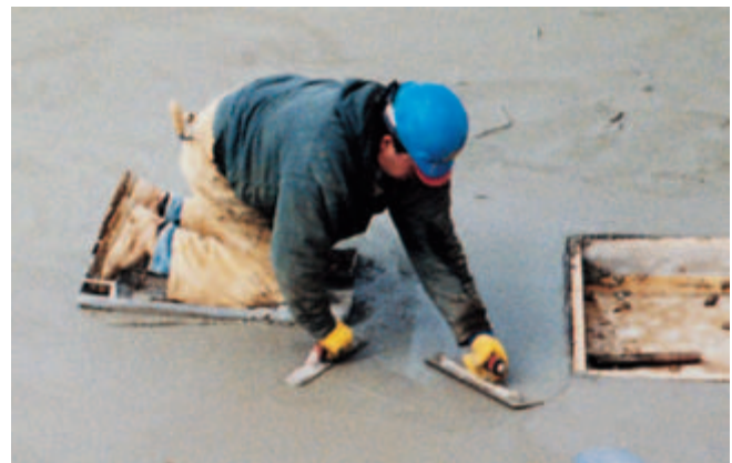
Fig. 11-19. Hand floating (right hand) the surface with a hand float held flat on the concrete surface and moved in a sweeping arc with a slight sawing motion. Troweling (left hand) with blade tilted is performed before moving the kneeboards. (IMG12378)
