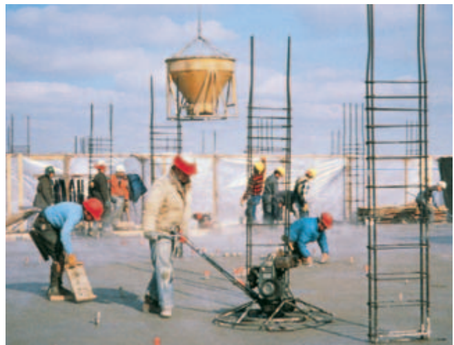
Fig. 14-9. Finishing this concrete flatwork can proceed because a windbreak has been provided, there is adequate heat under the slab, and the concrete has low slump. (IMG12278)
