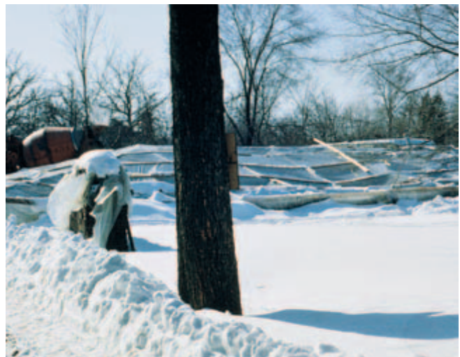
Fig. 14-17. Even in the winter, an outdoor swimming pool can be constructed if a heated enclosure is used. (IMG12269)
