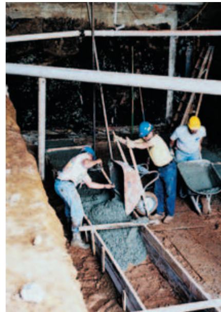
Fig. 11-4. Wheelbarrows are used to place concrete in areas that are not easily accessed by other placement methods. (IMG12368)
