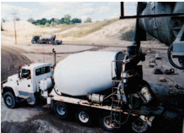
Fig. 10-3. Central mixing in a stationary mixer of the tilting drum type with delivery by a truck mixer operating at agitating speed. (IMG12391)
