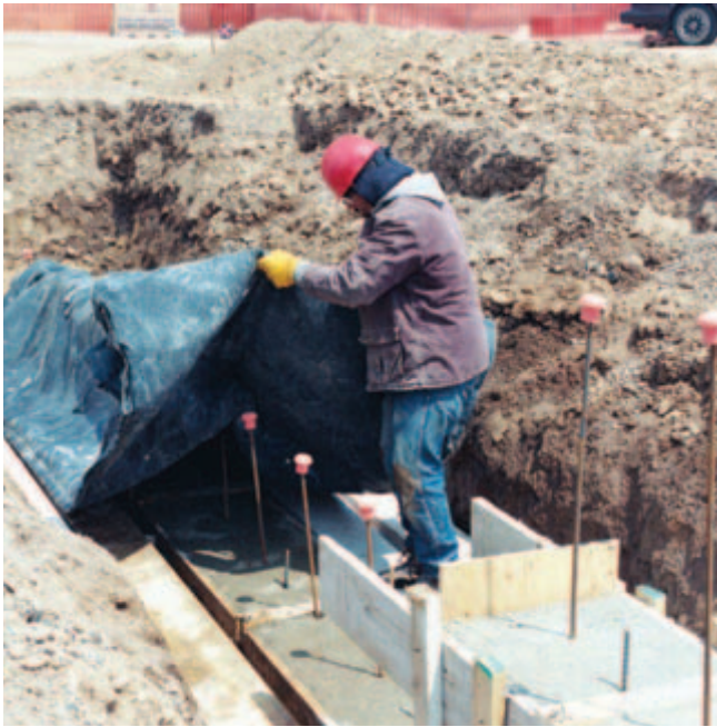
Fig. 14-8. Concrete footing pedestal being covered with a tarpaulin to retain the heat of hydration. (IMG15125)
