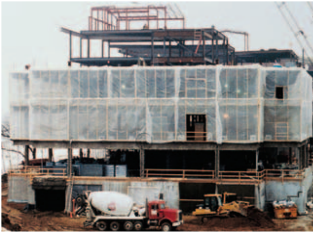
Fig. 14-18. (top) Tarpaulin heated enclosure maintains an adequate temperature for proper curing and protection during severe and prolonged winter weather. (bottom) Polyethylene plastic sheets admitting daylight are used to fully enclose a building frame. The temperature inside is maintained at 10°C (50°F) with space heaters. (IMG12205, IMG12204)
