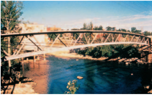
Fig. 17-9. The Sherbrooke footbridge in Quebec, built in 1997, is North America's first reactive-powder concrete structure. (IMG12342)
