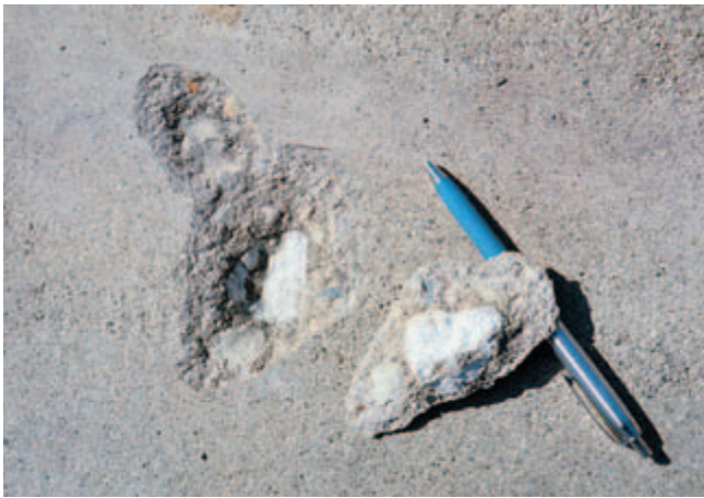
Fig. 5-18. A popout is the breaking away of a small fragment of concrete surface due to internal pressure that leaves a shallow, typically conical depression. (IMG12316)
