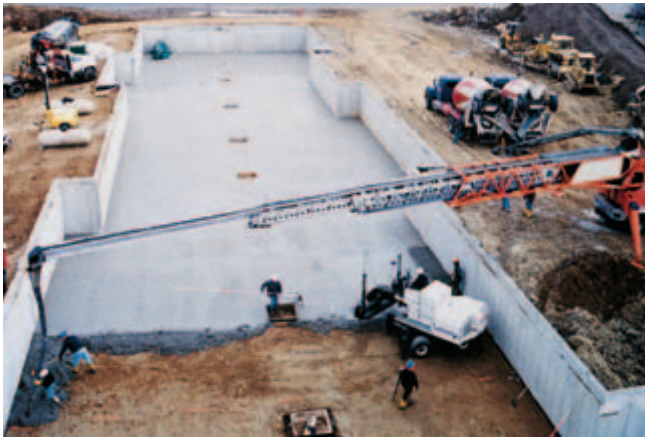
Fig. 10-13. The conveyor belt is an efficient, portable method of handling concrete. A dropchute prevents concrete from segregating as it leaves the belt; a scraper prevents loss of mortar. Conveyor belts can be operated in series and on extendable booms of hydraulic cranes. (IMG12395)
