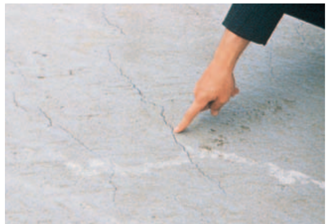
Fig. 13-7. Typical plastic shrinkage cracks. (IMG12267)
