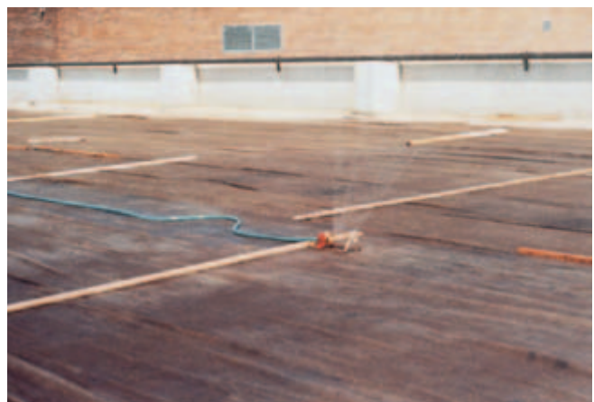
Fig. 12-5. Lawn sprinklers saturating burlap with water keep the concrete continuously moist. Intermittent sprinkling is acceptable if no drying of the concrete surface occurs. (IMG12263)
