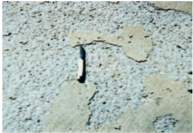
Fig. 6-3. Scaled concrete surface resulting from lack of air entrainment, use of deicers, and poor finishing and curing practices. (IMG12414)
