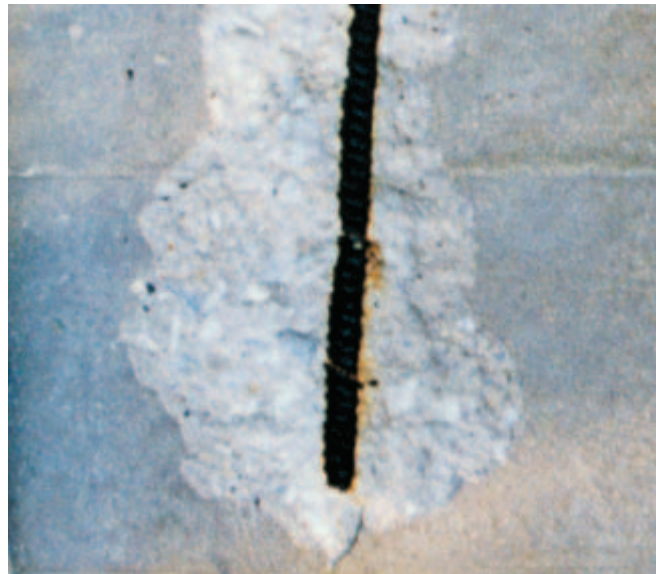
Fig. 1-29. Carbonation destroys concrete's ability to protect embedded steel from corrosion. All concrete carbonates to a small depth, but reinforcing steel must have adequate concrete cover to prevent carbonation from reaching the steel. This reinforcing bar in a wall had less than 10 mm (0.4 in.) of concrete cover; the ACI building code requires a minimum of 38 mm (1½ in.). After years of outdoor exposure, the concrete carbonated to the depth of the bar, allowing the steel to rust and spall the concrete surface. (IMG12499)
