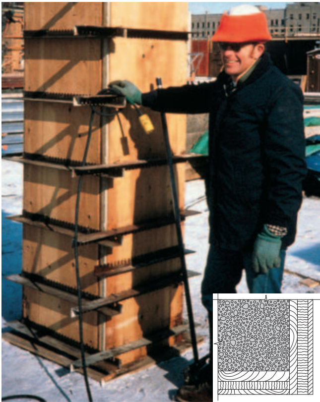
Fig. 14-21. With air temperatures down to -23^{\circ}\text{C} ( -10^{\circ}\text{F} ), concrete was cast in this insulated column form made of 19-mm ( \frac{3}{4} -in.) high-density plywood inside, 25-mm (1-in.) rigid polystyrene in the middle, and 13-mm ( \frac{1}{2} -in.) rough plywood outside. R value: 1.0\text{ m}^2 \cdot ^{\circ}\text{C}/\text{W} ( 5.6\text{ [}^{\circ}\text{F} \cdot \text{hr} \cdot \text{ft}^2\text{]}/\text{Btu} ). (IMG12274)
