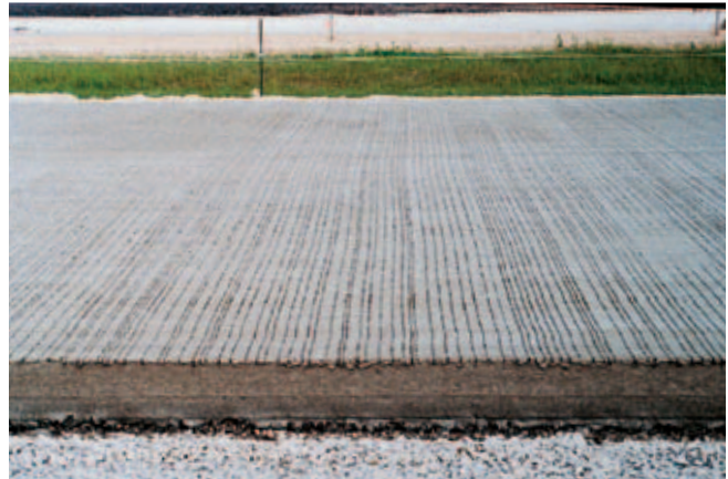
Fig. 11-21. (top) This machine is tining the surface of fresh concrete. (bottom) Tining of pavements improves tire traction and reduces hydroplaning. (IMG12376, IMG12375)
