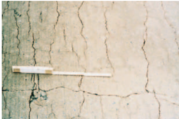
Fig. 5-20 (top and bottom). Cracking of concrete from alkali-silica reactivity. (IMG12421, IMG13049)
