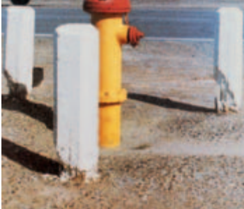
Fig. 1-31. Sulfate attack is often the most severe at the location of the most wetting and drying, which is usually near the soil line. Here concrete posts have been attacked by sulfates near the soil line. Also see the inset in Fig. 1-32. The concrete is in better condition deep within the soil where it is moist. (IMG12497)
