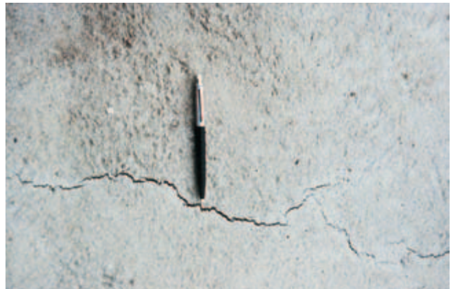
Fig. 15-6. Plastic shrinkage cracks resemble tears in fresh concrete. (IMG12283)
