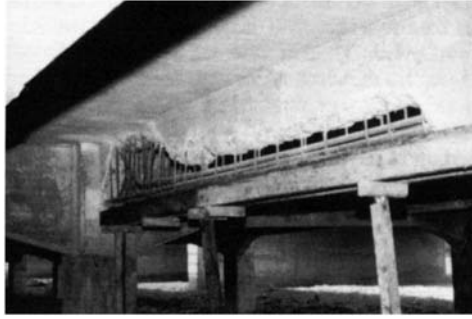
Fig. 9. Medium sized repair suitable for the use of “flowing concrete” type material prior to the fixing of the side shutters and the letter box placement openings
