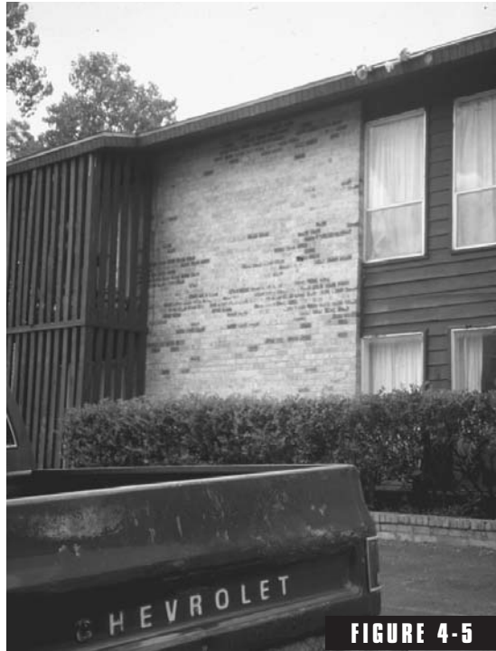
Uneven color distribution. (from Beall, Christine, Masonry Design and Detailing, 4th edition, McGraw-Hill, New York ).
