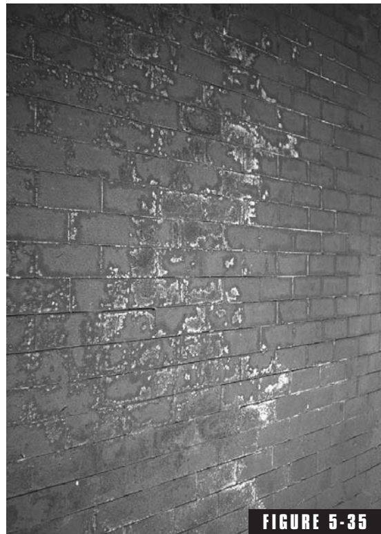
FIGURE 5-35 Masonry efflorescence. (from Beall, Christine, Masonry Design and Detailing , 4th edition, McGraw-Hill, New York).
