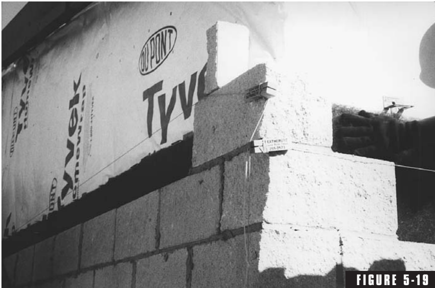
A masonry line block holds the string in place so units can be laid to the line.
