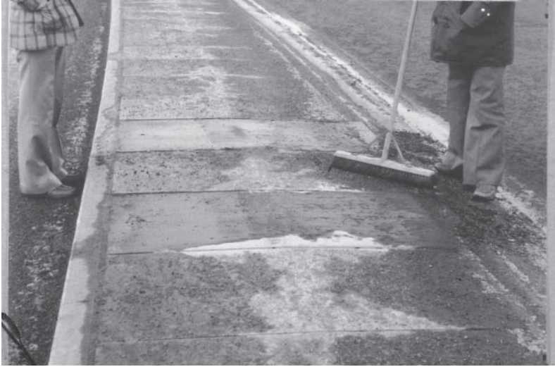
Figure 5.19 Scaling of a concrete surface owing to freeze–thaw, exacerbated by de-icing salts.
