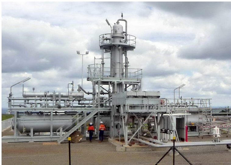
Fig. 6.13 Cougar Energy gas treatment plant at Kingaroy site.
