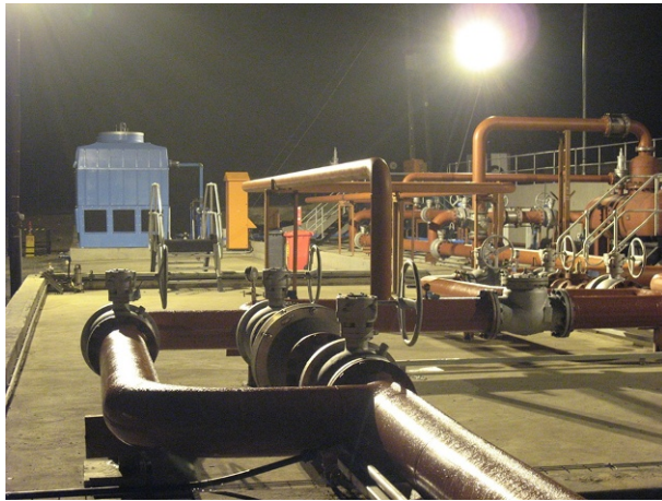
Fig. 14.19 15,000 Nm 3 /h gas treatment plant.
