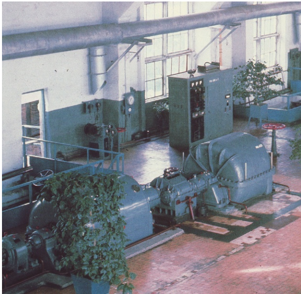
Picture 3.4 Engine room of the compressor plant.
