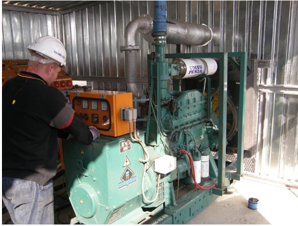
Fig. 14.14 Modified diesel generator operating on \epsilon UCG gas.
