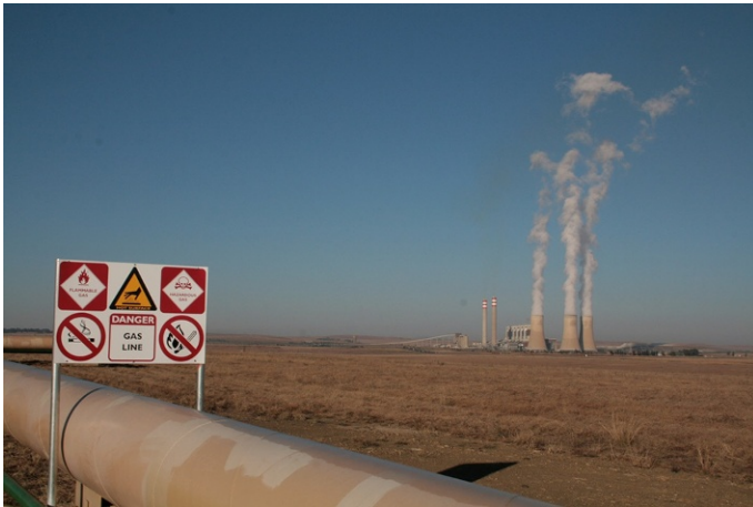
Fig. 14.15 UCG gas pipeline to Majuba Power Station.
