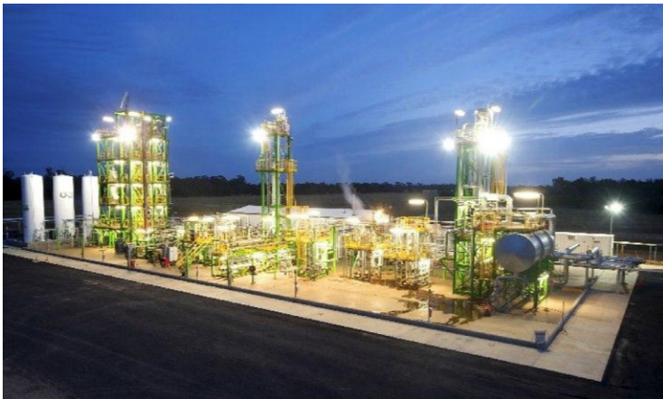
Fig. 6.6 Linc Energy GTL plant at Chinchilla.
