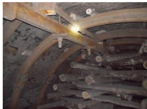
Figure 2. The condition of the hauling roadway of the 4 th longwall, h_9 seam, Tsentrosoyuz mine, in the area of the roadway junction with the breakage face.
