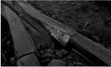
Figure 3. Wear of inner surface of the rail on a bend of a switch.
