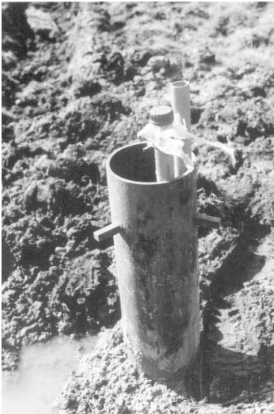
Figure 9.4 Piezometer group measuring water levels in two formations in an opencast working. (Photograph by LPT.)
