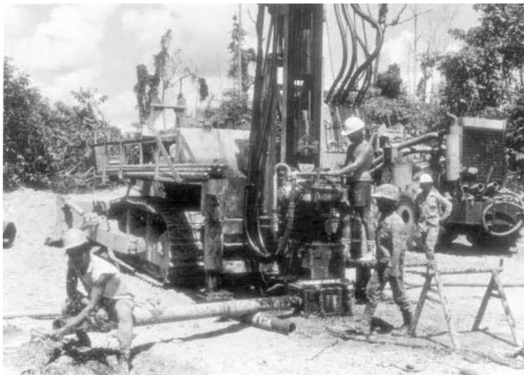
Figure 6.14 Dando dual air–mud flush rig mounted on a bulldozer for use in difficult tropical terrain. (Photograph by M. C. Coultas.)
