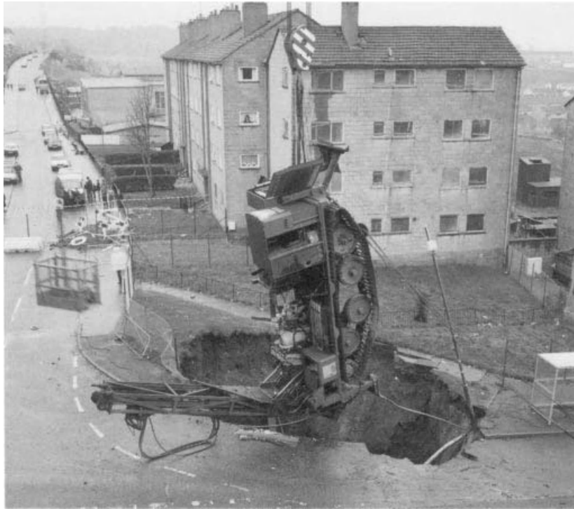
Figure 12.11 Collapse of capping material over an old concealed shaft in a modern urban area, United Kingdom. (Photograph by courtesy of IPR/25-36c British Geological Survey. © NERC. All rights reserved.)
