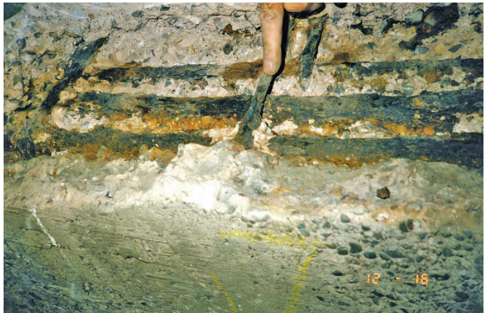
Figure 10.2 – Severe main bar corrosion
