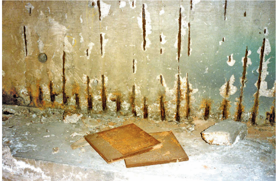
Figure 3.2 – Concrete spalling due to corrosion of panel wall reinforcement
