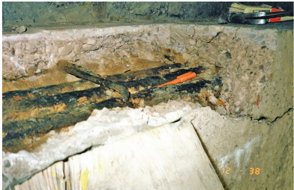
Figure 10.1 – Torsion bar corroded right through
