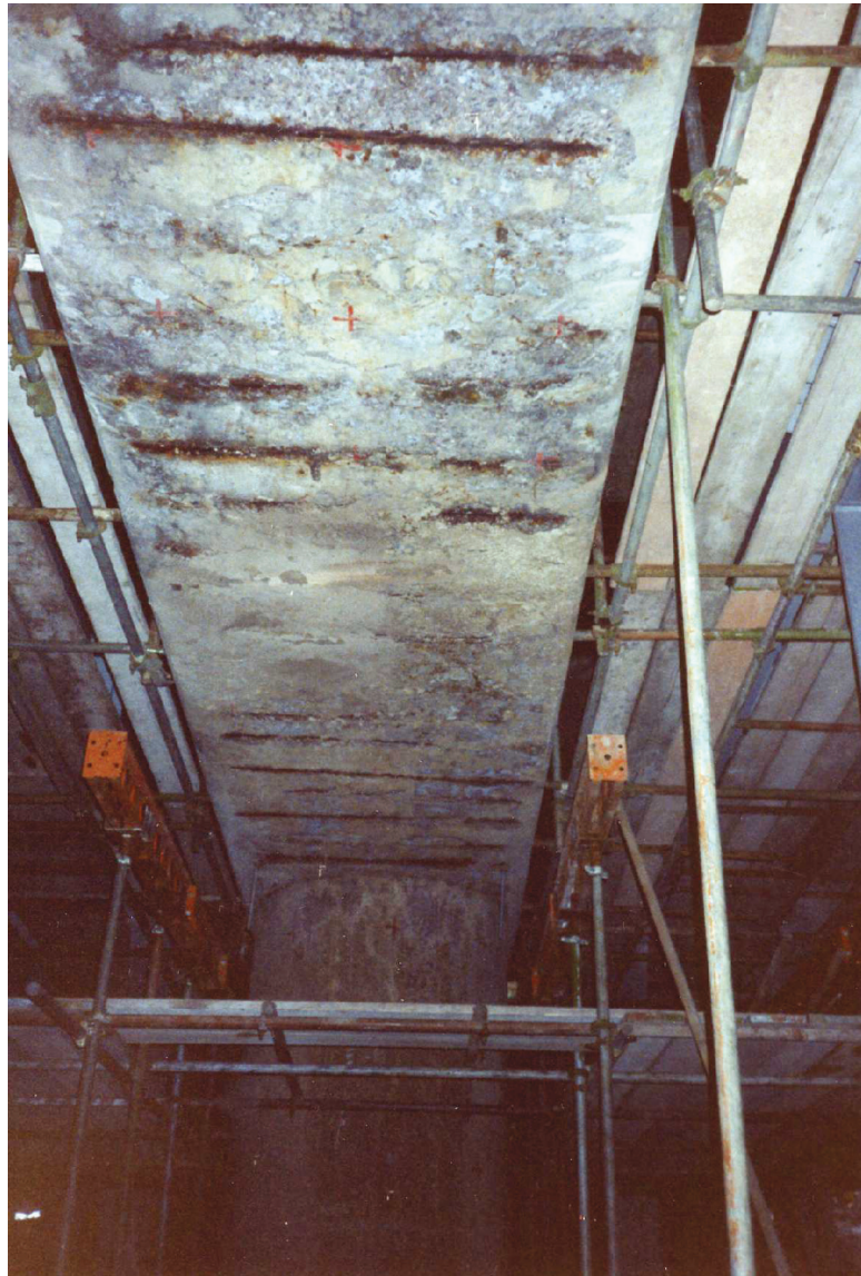
Figure 2.1 – Deteriorated crossbeam soffit
