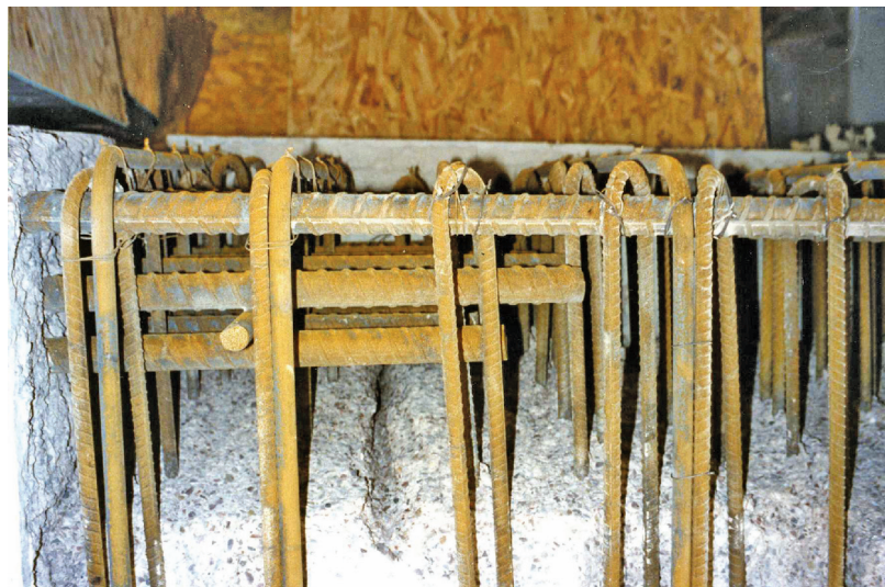
Figure 1.6 – Top of crossbeam broken out to enable insertion of anchor bars for strengthening nibs
