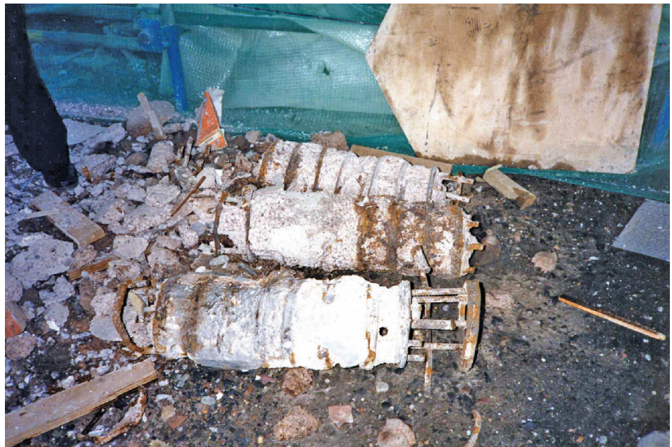
Figure 15.7 – Discarded deteriorated stub columns
