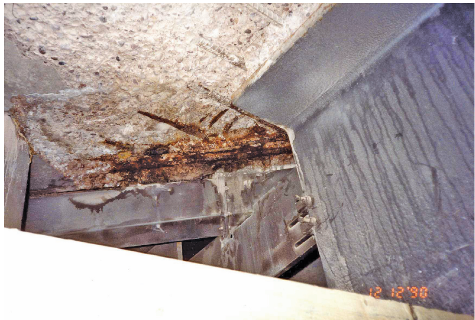
Figure 19.1 – Deck soffit corrosion
