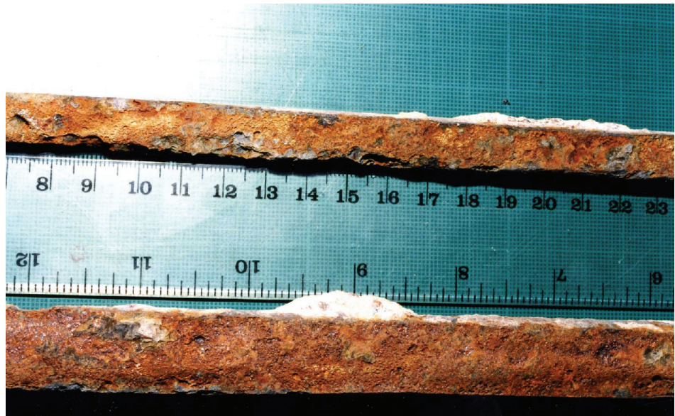
Figure 16.1 – Deck rebar pitting corrosion
