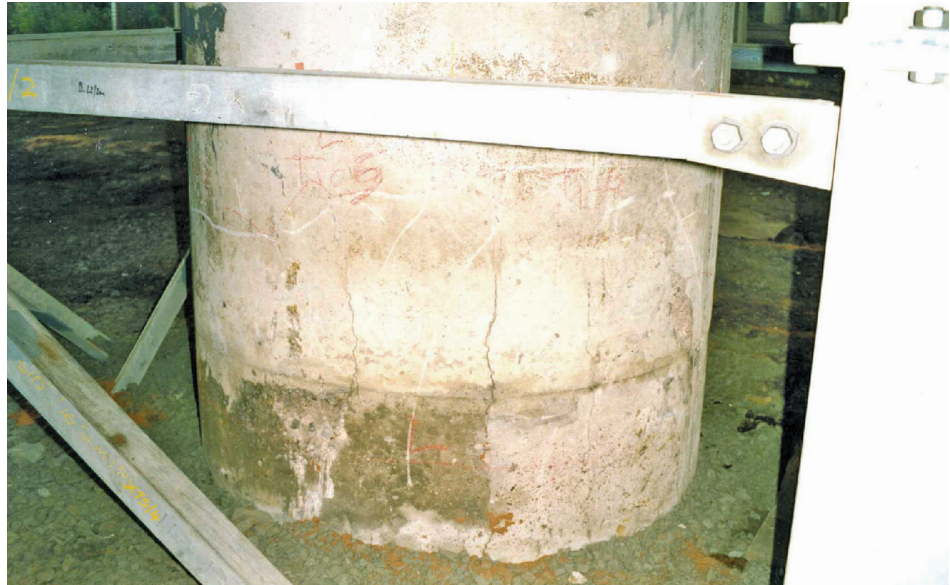
Figure 8.1 – Cracks indicating column delamination
