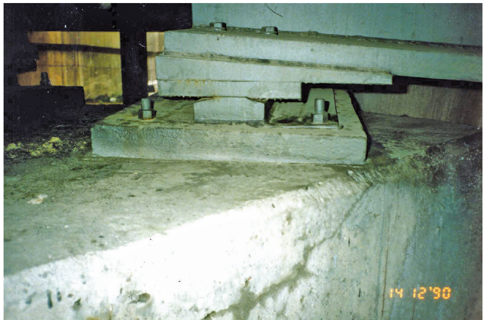
Figure 15.5 – Steel rocker bearing. No bearing stiffeners
