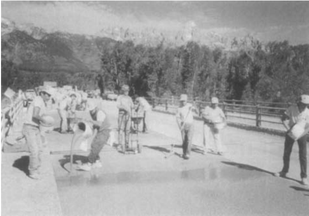
Fig. 5.3. Overlay of 3/8 in. polymer concrete installed in Grand Teton National Park helps protect bridge deck (Photo courtesy Transpo Industries).
