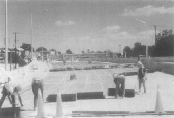
Fig. 5.4. Reinforcing steel in this bridge deck is protected against corrosion by cathodic protection offered by titanium anode mesh (Courtesy Corpro Companies Inc.).
