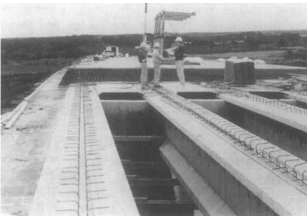
Fig. 5.2. Traditional reinforced concrete deck is finished by worker standing on bridge attached to rolling screed. Concrete containing calcium nitrate plasticizer is pumped onto removable plywood formwork (Photo courtesy W. R. Grace).
