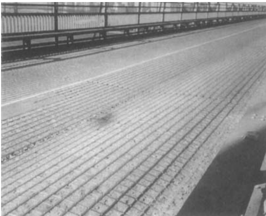
Fig. 4.2. Concrete-filled steel grid deck exhibits deterioration known as "growth" phenomenon on the Williamsburg Bridge in New York City.
