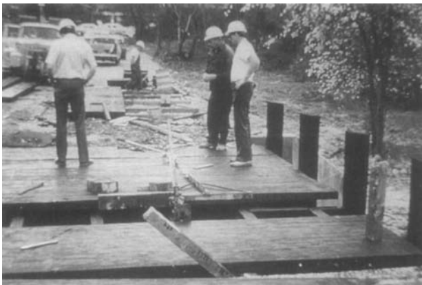
Fig. 6.5. Doweled glulam panels were field assembled to construct deck of all-timber bridge.
