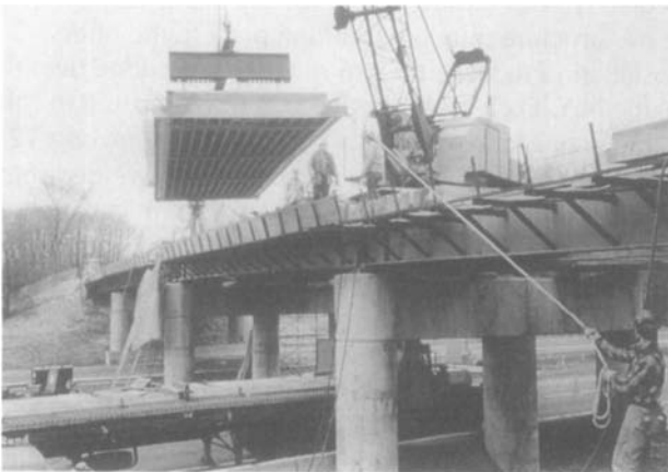
Fig. 6.2. Precast exodermic modules form the deck of bridge over New York State Thruway near Albany.
