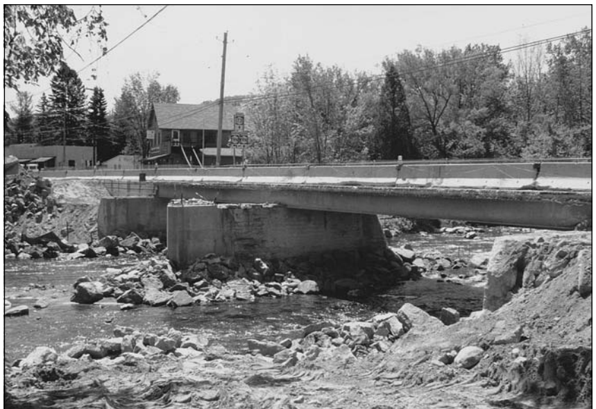
Figure 4.11 It's time for this solid wall pier, located in a stream crossing, to be replaced.
