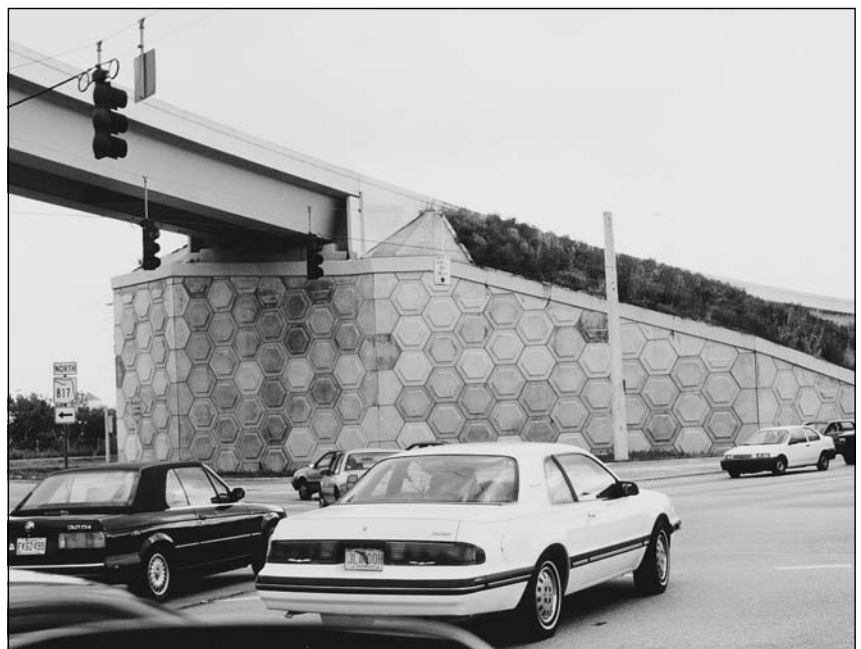
Figure 4.2 A reinforced earth abutment is used to support this composite steel bridge.
