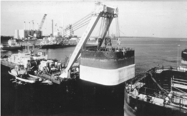
FIGURE 3.30 Setting prefabricated box caisson on which is mounted a temporary cofferdam, Great Belt Eastern Bridge, Denmark.
