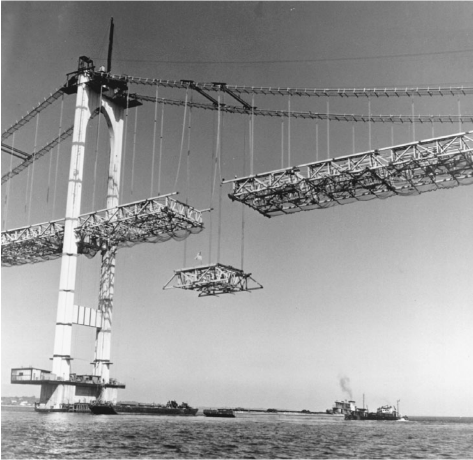
FIGURE 1.40 Suspended deck steelwork erection, Newport Bridge suspension spans, Narragansett Bay, R.I., 1968. Closing mainspan deck section is being raised into position by two cable travelers, each made up of a pair of 36 in. (0.91 m) wide-flange rolled beams that ride cables on wooden wheels. Closing section is 40-1/2 ft (12 m) long at top-chord level, 66 ft (20 m) wide and 16 ft (5 m) deep, and weighs about 140 tons. (Courtesy of Bethlehem Steel Corporation.)
