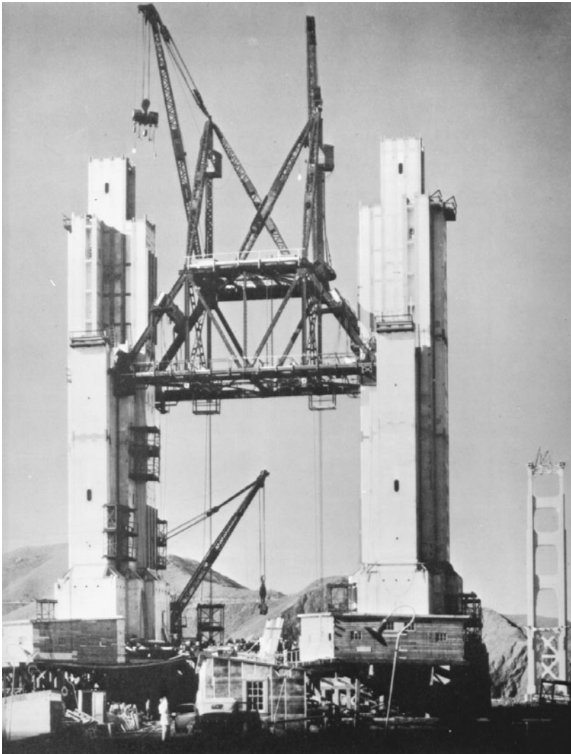
FIGURE 1.22 Erecting south tower of Golden Gate Bridge, San Francisco, 1935. A creeper traveler with two 90 ft (27 m) booms erects a tier of tower cells for each leg, then is jumped to the top of that tier and proceeds to erect the next tier. The tower legs are 90 ft (27 m) center-to-center and 690 ft (210 m) high. When the traveler completed the north tower (in background) it erected a Chicago boom on the west tower leg, which dismantled the creeper, erected tower-top bracing, and erected two small derricks (one shown) to service cable erection. Each tower contains 22,200 tons of steelwork.
