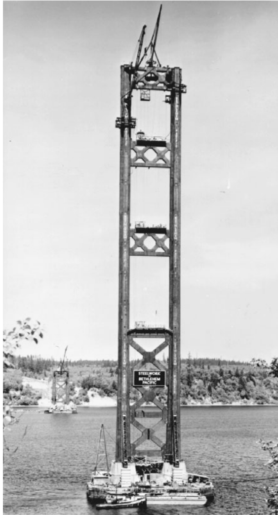
FIGURE 1.24 Tower erection, second Tacoma Narrows Bridge, Washington, 1949. This bridge replaced first Tacoma Narrows bridge, which blew down in a 40 mph (18 m/sec) wind in 1940. Tower legs are 60 ft (18 m) on centers and 462 ft (141 m) high. Creeper traveler is shown erecting west tower, in background. On east tower, creeper erected a Chicago boom at top of south leg; this boom dismantled creeper, then erected tower-top bracing and a stiffleg derrick, which proceeded to dismantle Chicago boom. Tower manhoist can be seen at second-from-topmost landing platform. Riveting cages are approaching top of tower. Note tower-base erection kneebraces, required to ensure tower stability in free-standing condition (see Figure 1.27 ).
