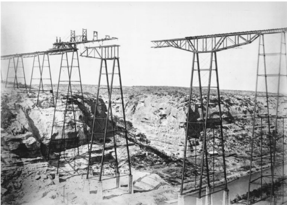
FIGURE 1.19 Pecos River railway viaduct, Texas, 1892. Erection by massive steam-powered wood traveler having many sets of falls and very long reach. Cantilever-truss main span has 185 ft (56 m) clear opening.
