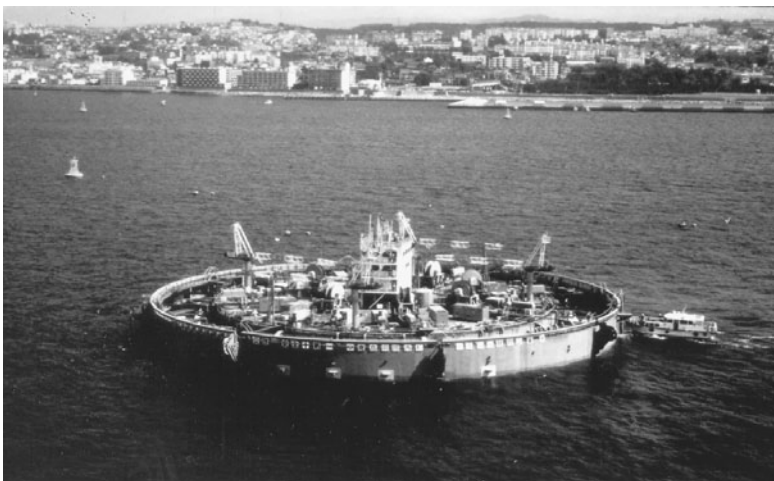
FIGURE 3.20 Akashi Strait Suspension Bridge is founded on steel box caissons filled with tremie concrete.
