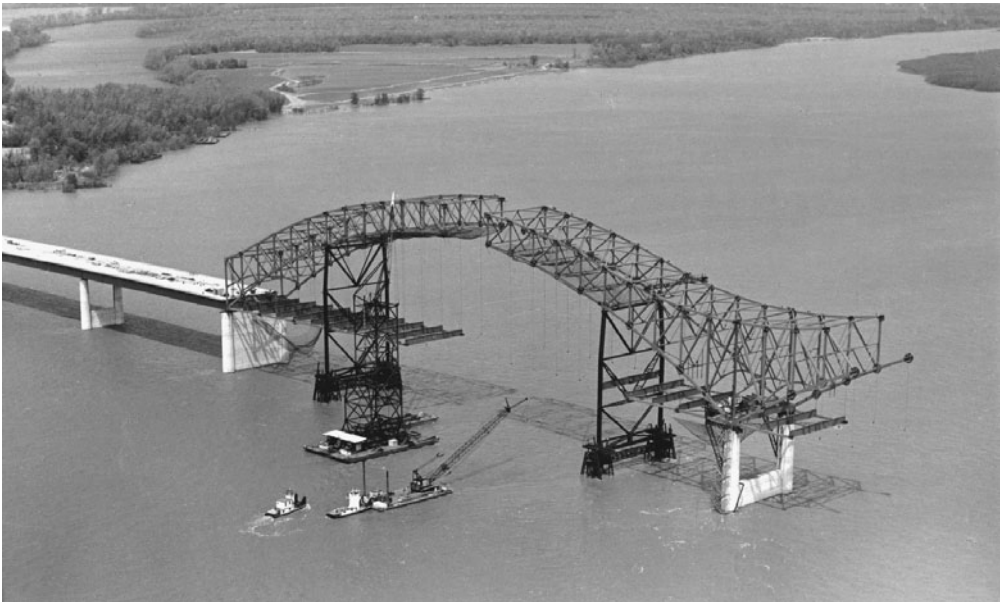
FIGURE 1.43 Erection of west arch span of twin-arch Hernando de Soto Bridge, Memphis, Tenn., 1972. The two 900 ft (274 m) continuous-truss tied-arch spans were erected by a high-tower derrick boat incorporating a pair of barges. West-arch steelwork (shown) was cantilevered to midspan over two pile-supported falsework bents. Projecting east-arch steelwork (at right) was then cantilevered to midspan (without falsework) and closed with falsework-supported other half-arch. (Courtesy of Bethlehem Steel Corporation.)
