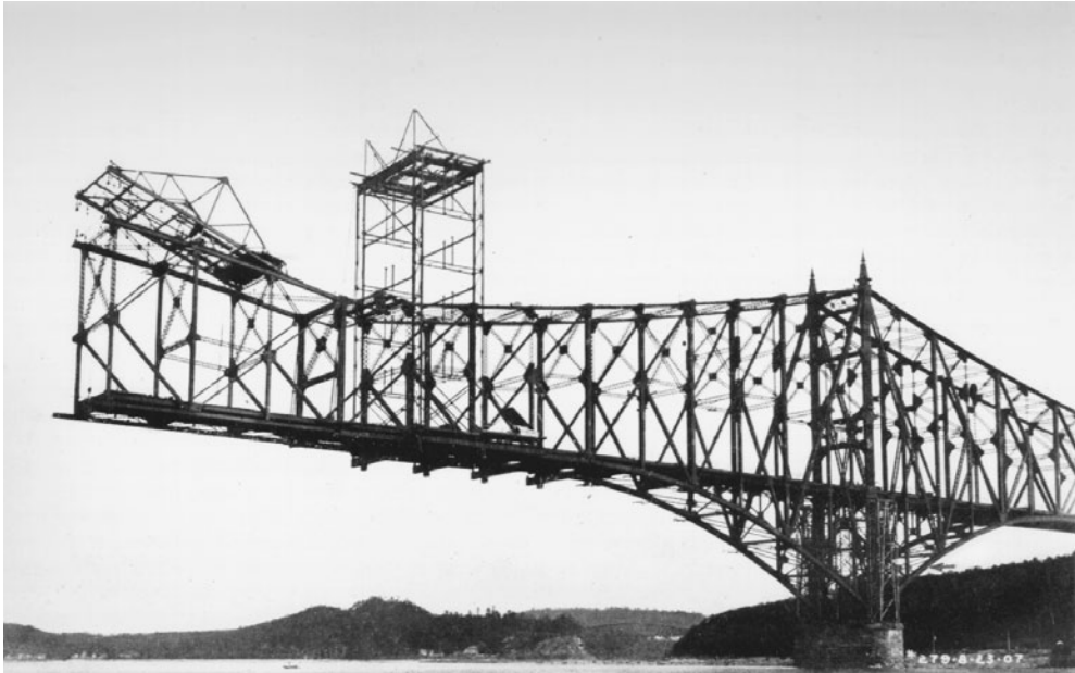
FIGURE 1.11 First Quebec railway cantilever bridge, 23 August 1907. Cantilever erection of south main span is shown six days before collapse. The tower traveler erected the anchor span (on falsework) and then the cantilever arm; then erected the top-chord traveler, which is shown erecting suspended span at end of cantilever arm. The main span of 1800 ft (549 m) was the world's longest of any type. The sidespan bottom chords second from pier (arrow) failed in compression because laticing connecting chord corner angles was deficient under secondary bending conditions.
