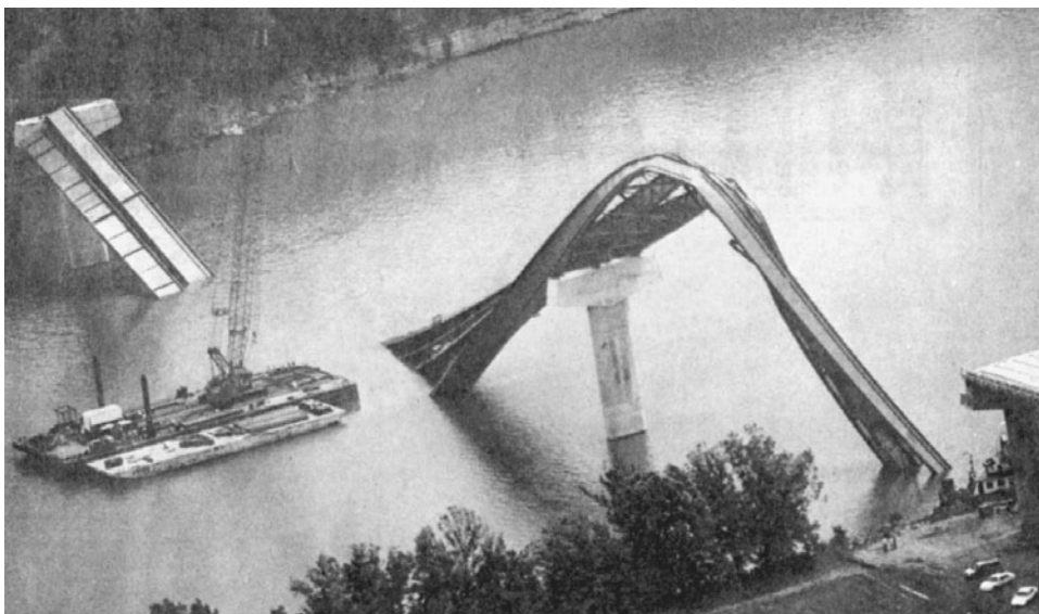
FIGURE 1.1 Failure of a steel girder bridge during erection, 1995. Steel bridge failures such as this one invite suspicion that the construction engineering aspects were not properly attended to.
