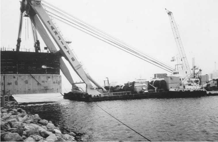
FIGURE 3.29 Lifting box caisson from quay wall on which it was prefabricated and transporting it to site while suspended from crane barge.
