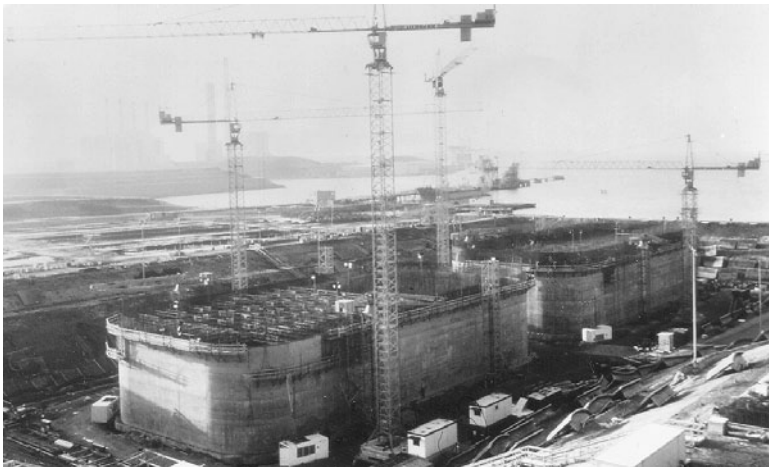
FIGURE 3.23 Large concrete box caissons fabricated in construction basin for subsequent deployment to site by self-flotation, Great Belt Eastern Bridge, Denmark.
