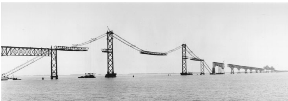
FIGURE 1.6 Suspension spans of first Chesapeake Bay Bridge, Maryland, 1952. Deck steelwork is under erection and is about 50% complete. A typical four-panel through-truss deck section, weighing about 100 tons, is being picked in west side span, and also in east side span in distance. Main span is 1600 ft (488 m) and side spans are 661 ft (201 m); towers are 324 ft (99 m) high. Cables are 14 in. (356 mm) in diameter and are made up of 61 helical bridge strands each (see Figure 1.8 ).
