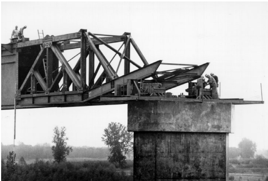
FIGURE 1.41B Launching nose rides up onto pier 5 skidway units, removing girder-train leading-end sag.
