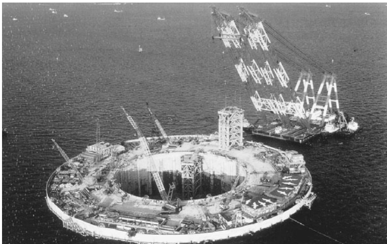
FIGURE 3.10 Slurry wall cofferdam for Kawasaki Island ventilation shaft, Trans-Tokyo Bay tunnels and bridge.
