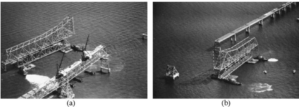
FIGURE 1.30 Floating-in erection of a truss span, first Chesapeake Bay Bridge, Maryland, 1951. Erected 300 ft (91 m) deck-truss spans form erection dock, providing a work platform for two derrick travelers. A permanent deck-truss span serves as a falsework truss supported on barges and is shown carrying the 470 ft (143 m) anchor arm of the through-cantilever truss. This span is floated to its permanent position, then landed onto its piers by ballasting the barges. (a) Float leaves erection dock, and (b) float arrives at permanent position. (Courtesy of Bethlehem Steel Corporation.)
