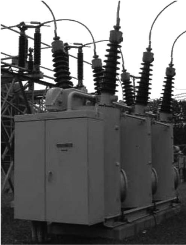
FIGURE 10.13 HV oil circuit breaker in outdoor substation yard.
