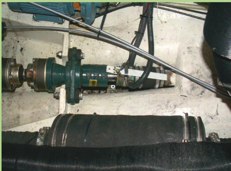
A proper grounded system should have all parts connected and a plate on the outside of the hull.
