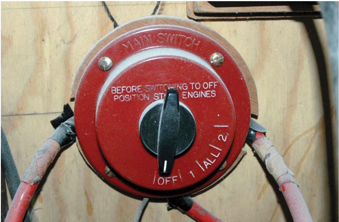
The old battery isolator had some oxidised surfaces, and needed replacement as well.
