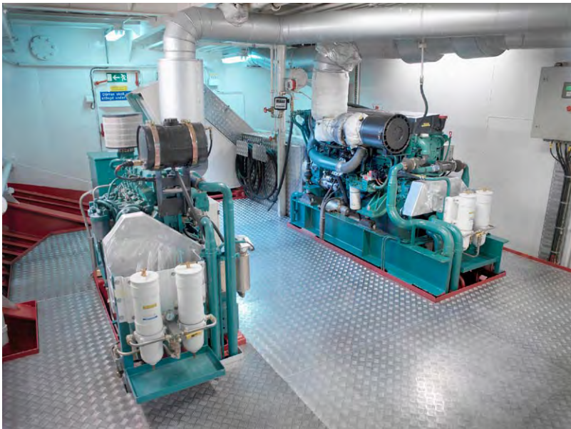
FIGURE 30.45 Two Volvo Penta D16 MH engines arranged to power a double-ended road ferry
