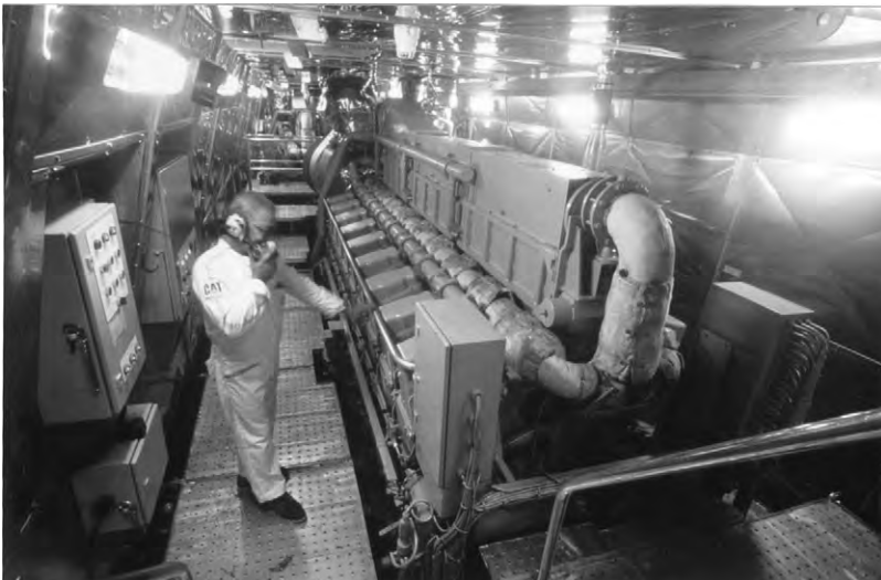
FIGURE 19.3 One of four 7200 kW Caterpillar 3618 engines installed in a fast catamaran ferry
