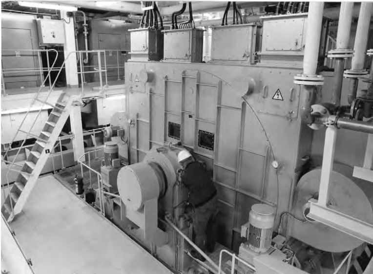
FIGURE 6.5 One of two 15 000 kW STN Atlas propulsion motors installed on the cruise liner Costa Victoria
