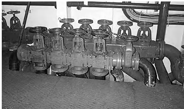
Figure 5.3 A ballast system valve chest
