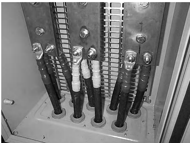
Figure 6.6 Part of a distribution panel with cable attachments
