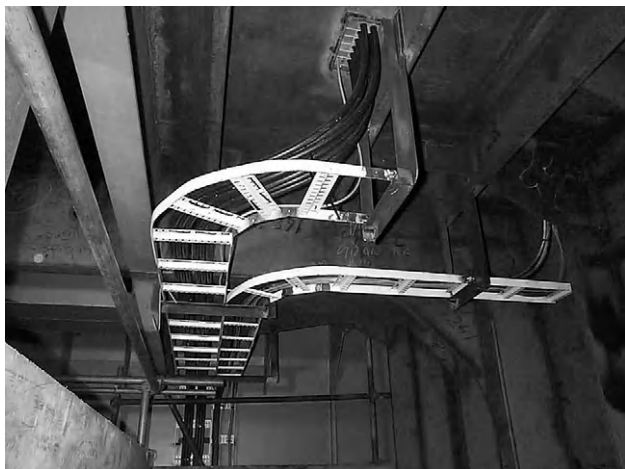
Figure 6.5 Grouping of electric cables on a cable tray
