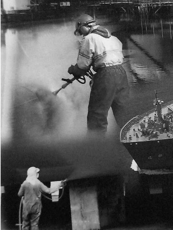
Figure 2.3 Hull preparation by water blasting (top) and hull painting by airless spray (bottom)
