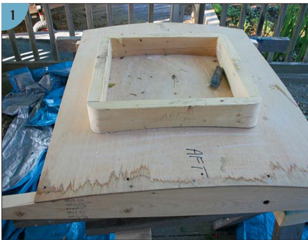
(1) The plywood mold for the new deck section sits on 2 x 8s that replicate the deck camber. The wooden frame standing on a square of plywood in the center of the mold marks the outside perimeter of the opening for the new Lewmar 60 hatch. The foam core for the new hatch boss will butt up against the outside of this wooden frame. (2) Here we're laminating the new deck section over the mold. We placed a sheet of plastic over the plywood mold to stop the resin from sticking to it, then laid down the \frac{3}{8} -inch (9 mm)
