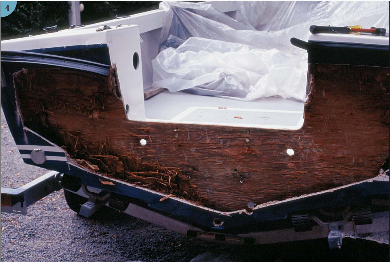
(4) This is what remained of the transom after I removed the rotted core.
