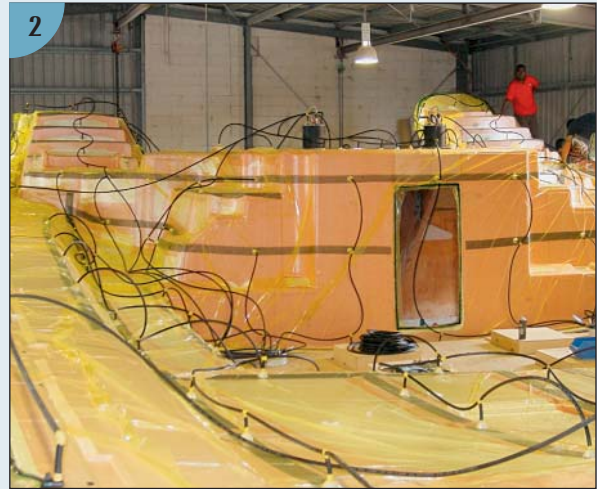
The infusion lines are in place, and as soon as the vacuuming is completed, the valves will be opened and resin will pass through the larger-diameter lines into the laminate. (Courtesy Perry Catamarans, Queensland Composites, and High Modulus)
