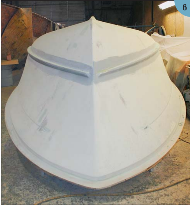
(6) When the hull plug is completely smooth, the spray rail, quarter rails, and a cove stripe are added. The flange at the bottom of the image (i.e., what will be the hull's sheerline) is for the deck mold to be fitted to the boat. The joint will be covered with a rubrail when the boat is built.
