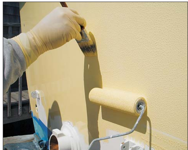
This topcoat application is proceeding toward the camera. The paint is rolled on with a foam roller, then tipped with a good-quality brush. (Courtesy Interlux)
