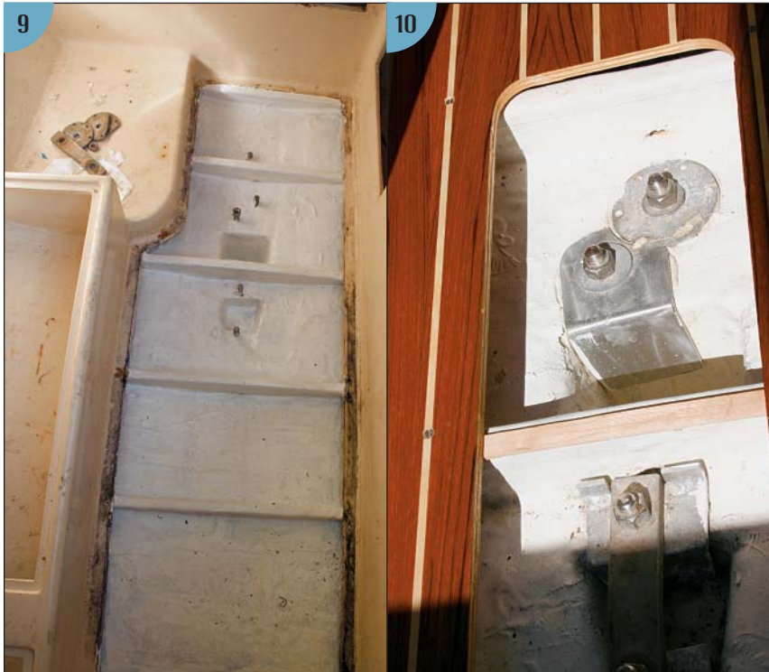
(9) We glassed the floors in place and painted out the entire area with Interlux Epoxy Primekote. The keel bolts fashioned for the lifting sling well are visible here. (10) A flange on the keel bolt washer is intended to protect the glasswork in the lifting sling area.
