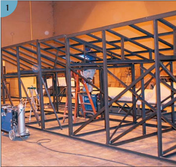
(1) The steel armature for a portion of a large yacht's upperworks is welded together.
