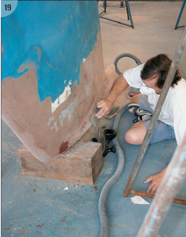
(18, 19) Then they sanded the fairing using a longboard with progressively finer grits. While the hull repair was curing, they turned to the keel, first straightening its tip and then using fairing compound to smooth out the imperfections.
