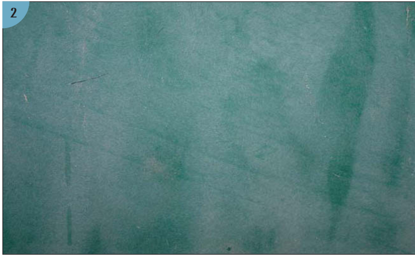
(2) This oxidized gelcoat could have been restored with aggressive compounding, but the hull had sustained other damage and the owner decided to paint the boat. (This is the hull of the J/24 owned by my son; other repairs to this boat are described in Chapters 5 and 7.)
