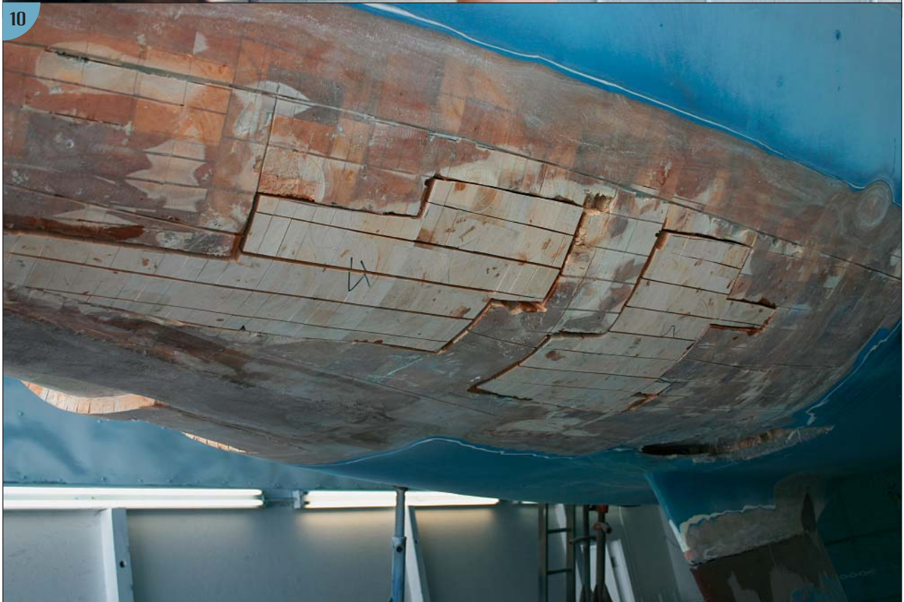
(9) Then they pressed the new core into place and clamped it until the resin hardened. (10) The finished core patch.
