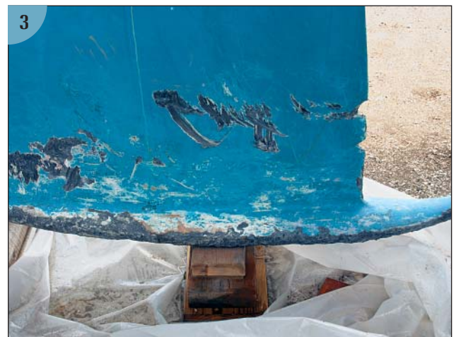
(3) The keel has also received its share of damage. Note the upturned tip on the keel bulb.
