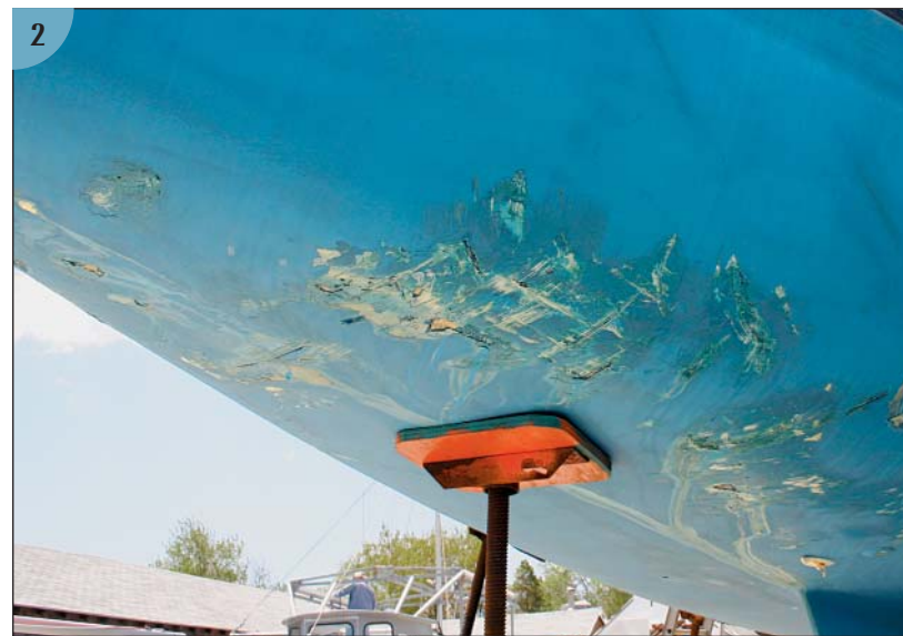
(2) A view of the damage a little farther aft. The rocks punched into the hull in several places, fracturing the outer laminate.
