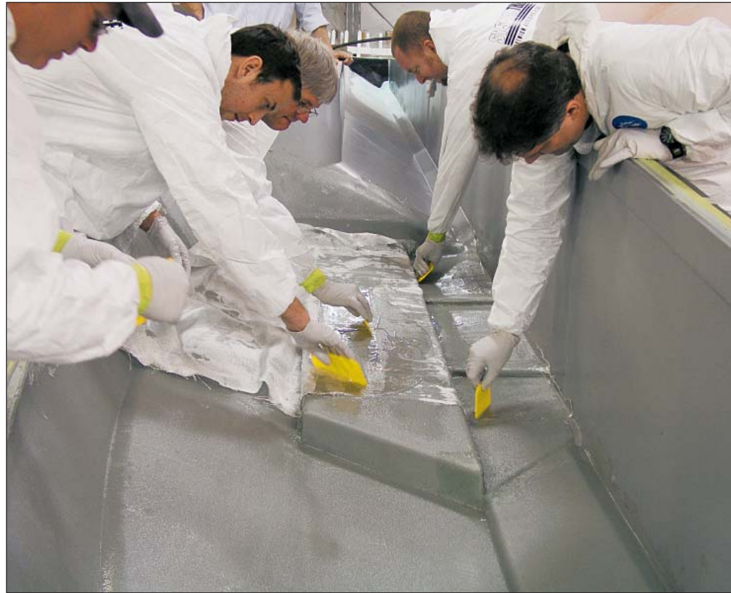
After coating the repair surface with well-mixed resin, lay your fiberglass in the wet resin. Add a little more resin on top of the fiberglass and roll it out to ensure that the entire surface is wet. Work from the center toward the edges to eliminate air bubbles. (Courtesy System Three)
