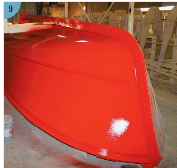
(9) The plug has been sprayed with red tooling gelcoat. This layer will be coated with mold release wax to allow the mold to peel away easily from the plug. The coats of resin and wax are thin enough not to change the shape of the plug. The plug will then be ready for constructing the hull mold.
