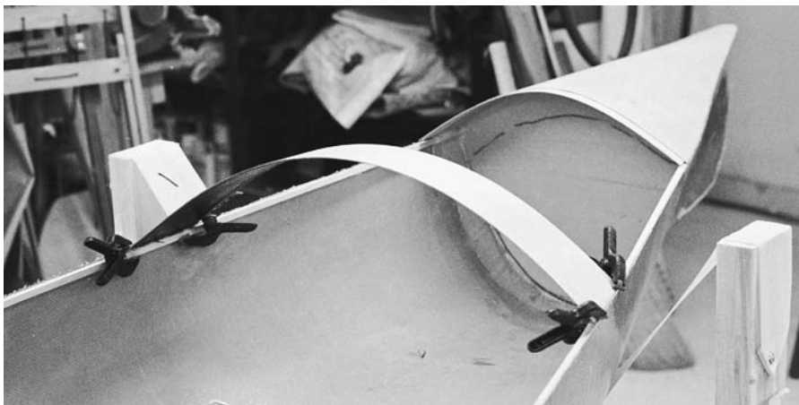
FIGURE 12.6. A plywood arch strip is clamped in place for trimming and test-fitting.
