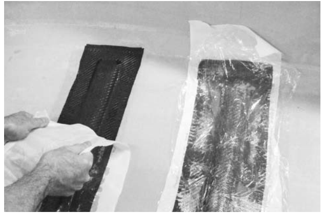
FIGURE 11.25. When the epoxy has set and the peel ply is removed, the ribs will blend smoothly into the hull.
