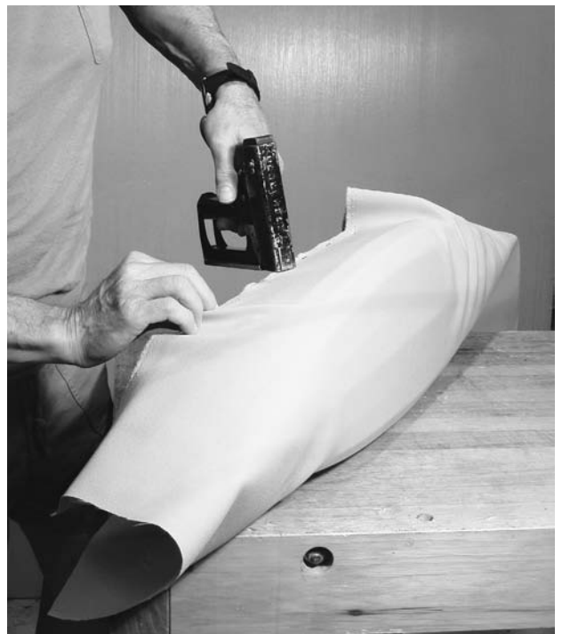
FIGURE 10.11. The fabric is stretched over the form and stapled to the mounting board.
