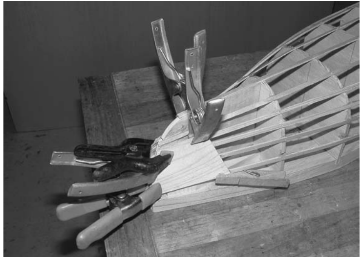
FIGURE 10.7. After all stringers are attached, optional 1-millimeter-thick cheek plates are glued and clamped in place with small spring clamps.
