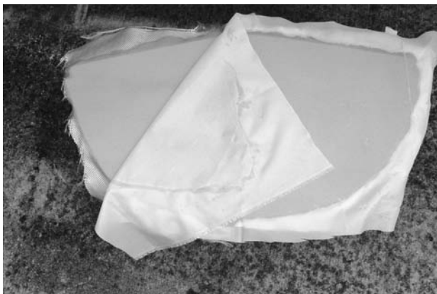
FIGURE 11.9. When the epoxy has cured, peel off the polyester layer. You will have a nicely textured surface ready for structural bonding of the bulkhead. Trim off excess Kevlar.
