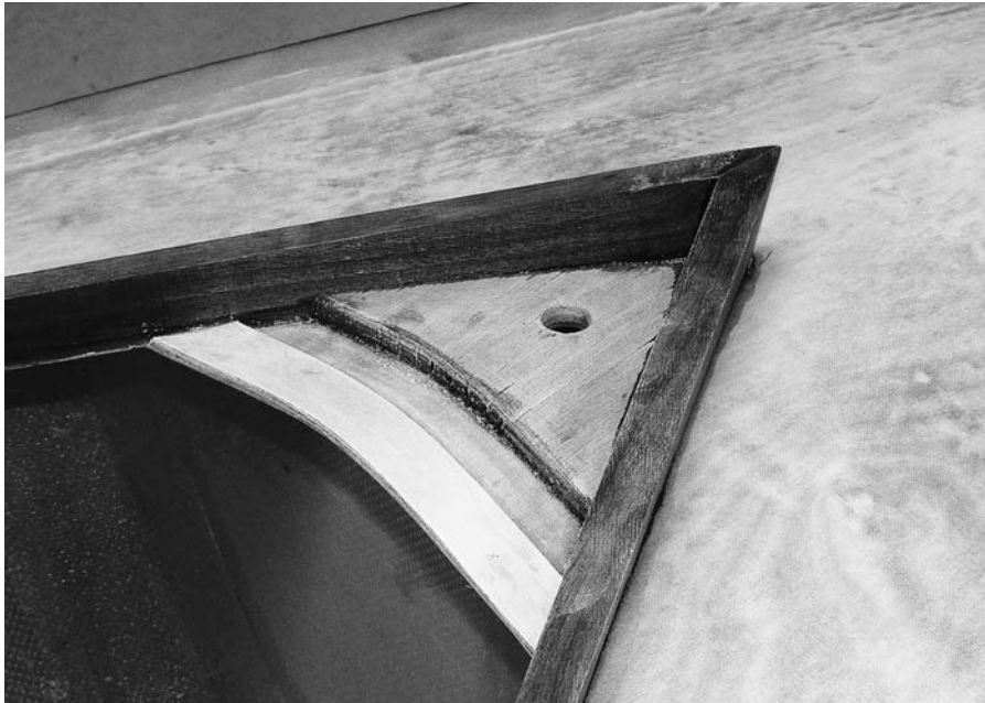
FIGURE 11.19. A drain hole is required in the deck of each end flotation chamber.
