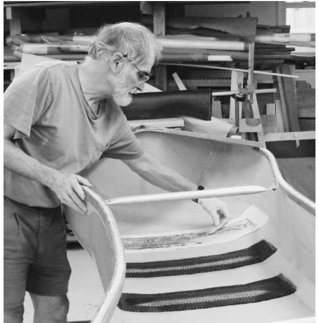
FIGURE 11.23. After wetting out carbon fiber, a layer of polyester fabric peel ply is applied.
