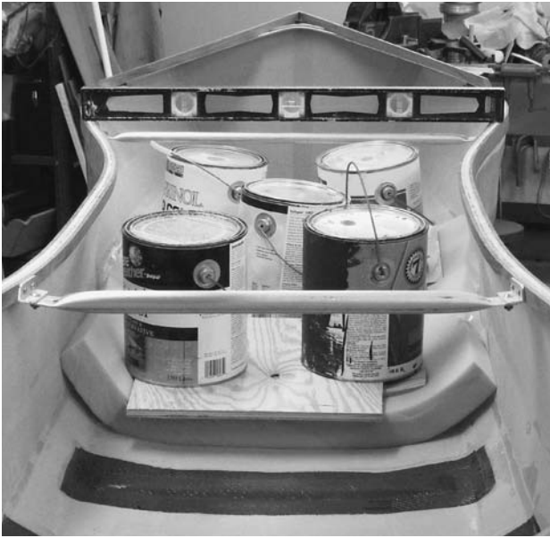
FIGURE 11.24. Soft foam 2 inches or thicker is placed on top of the ribs after the peel ply and plastic wrap. Scraps of plywood are weighted down—in this instance with paint cans—to compress the soft foam and apply pressure to the ribs as uniformly as possible. The plywood under the weights helps to distribute the load and prevents the hull from sagging down in the middle. It is best to position a third sling stand to support the hull under the rib being weighted. That will help to keep the hull from deforming from the designed shape.
