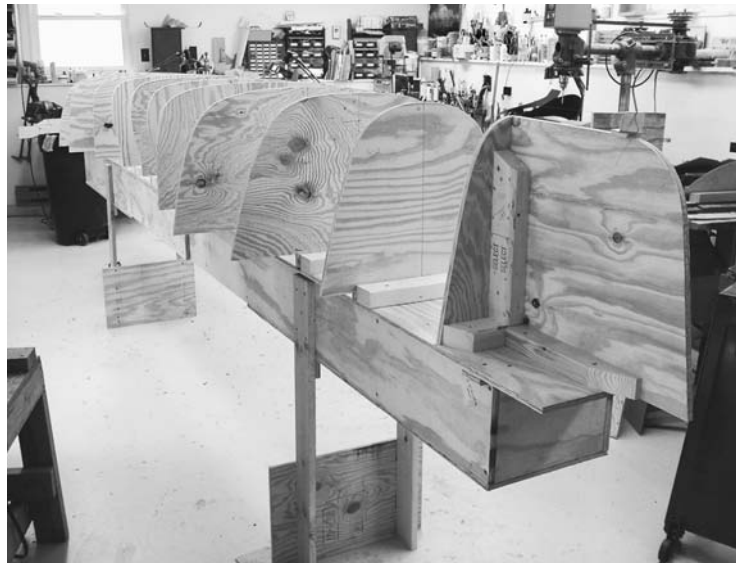
FIGURE 6.4. Pieces of 2 \times 4 are screwed to the strongback, and the stations are screwed to those 2 \times 4 s. Note the arrangement of 2 \times 4 s used to attach the end forms.
