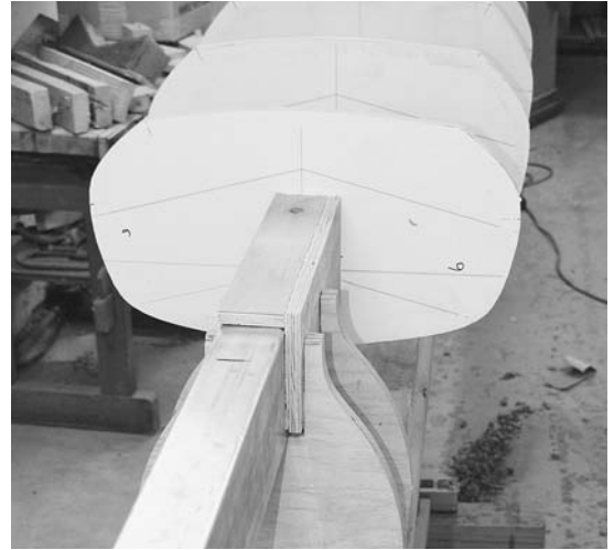
Figure 5-23. With this aluminum strongback, I use L-shaped spacers to hold the forms in place. The end forms are screwed in place, and wedges between the middle forms hold everything tight.
