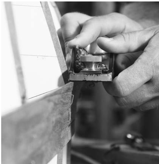
Figure 12-16. Clean up the edge with a rabbet plane. Try for a smooth, fair curve with a consistent angle on the bevel.
