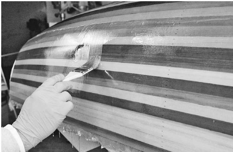
Figure 11-20. The fill coat fills up the fabric texture (right) to create a smooth finish (left). Brush on the epoxy using the same crisscross technique you will eventually use to apply varnish.
