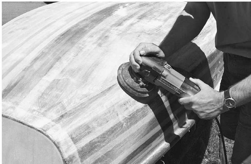
Figure 11-38. The fill coat should leave a quite smooth surface, but a good finish often requires some serious sanding. Start with 60-grit sandpaper on your random orbit sander. On the boat shown there were some rough spots along the edge where the fiberglass doubled up. The goal is to feather in these edges and level any irregularities in the surface so there are no shiny spots left on the surface. Along the edges of additional layers you will need to sand into the glass a little bit. However, if you start seeing signs of the fiberglass showing up elsewhere in the surface immediately adjacent to shiny spots, stop sanding that area. You will need to add another fill coat.
