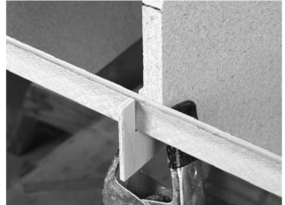
Figure 6-9. Getting the first strip aligned on the forms to create a smooth, fair curve may require a little finagling. Use some U-shaped jigs to temporarily hold the strip in place while checking the alignment. When you have it right, secure the strip in place with a staple or other fastener.
