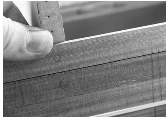
Figure 6-15. With most boats the sides are relatively flat, so very little beveling is required. Most small boats, however, will have some places where gaps will open up if you are using square-edged strips. These gaps may be eliminated by planing a rolling bevel as described earlier. Notice the double lines on the strips near the right side of the photo. These help align the grain while installing strips cut consecutively from the board.
