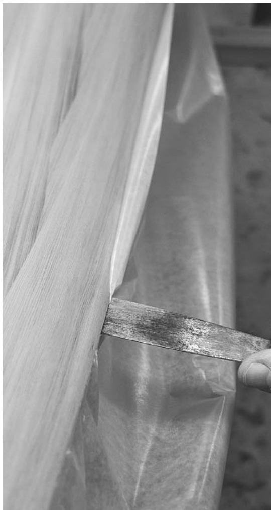
Figure 13-43. Slide a sheet of waxed paper in between the deck and hull to protect the other half as you stain and epoxy. The seam may be quite tight—I find that a putty knife helps coax the paper into the sheer seam.
