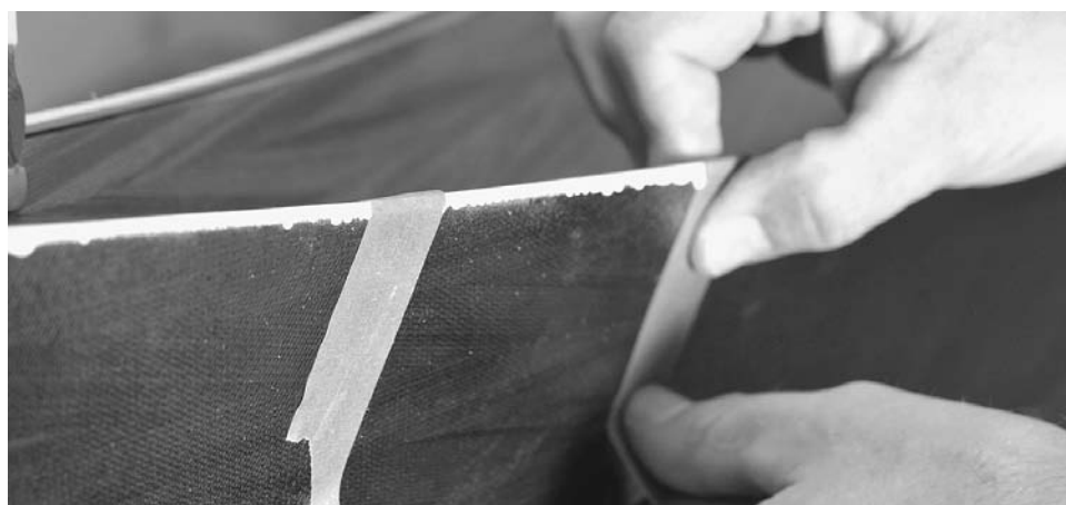
Figure 13-48. I installed a feature strip of light-colored contrasting wood along the top edge of the hull after the rest of the outside had been stained and fiberglassed. I glued it down and secured it with tape. After installation you can glass the inside. The outside will be reinforced when the deck is attached and the seam is glassed.
