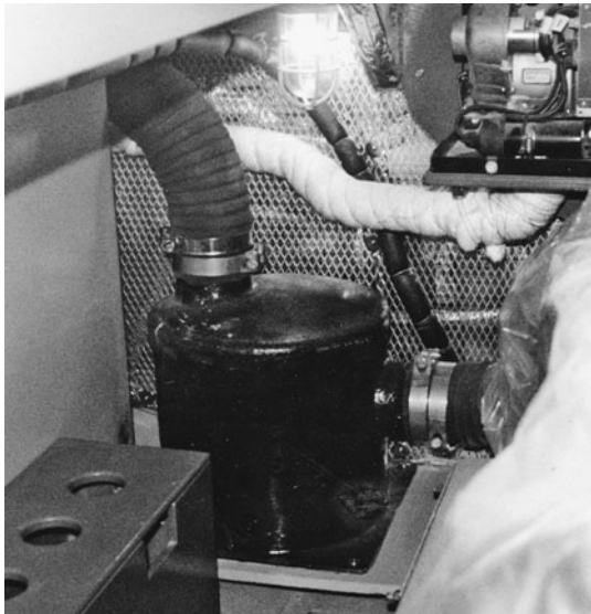
Figure 7-11. Waterlift muffler installed
