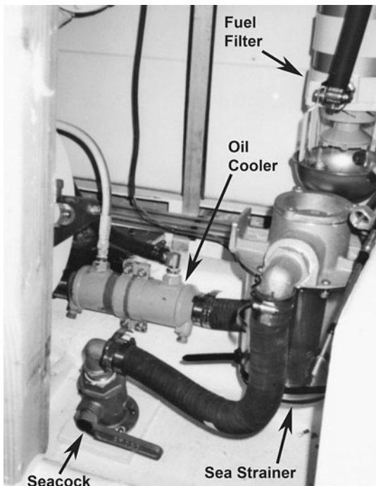
Figure 4-10. Return oil cooler
