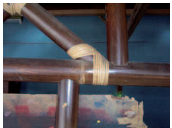
Figure 3-7: Eccentricity of force transfer and the effort placing the joints near to the node
