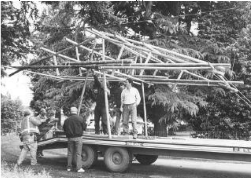
This structure was built under the direction of Simon Velez by unskilled Americans in a day
