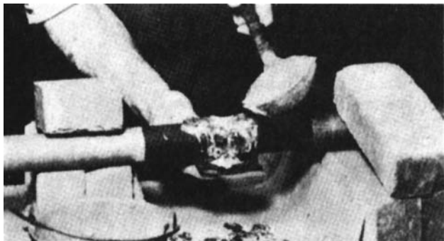
Fig. 10-4 Solder has just been poured on the joint and that caught in the cloth is being pressed against the bottom to get up heat.
