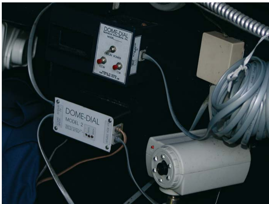
Figure 2.14. Dome-Dial display unit and relay box, mounted on observatory wall. Black-and-white security camera is also shown. (Used with permission, Technical Innovations, Inc.)
