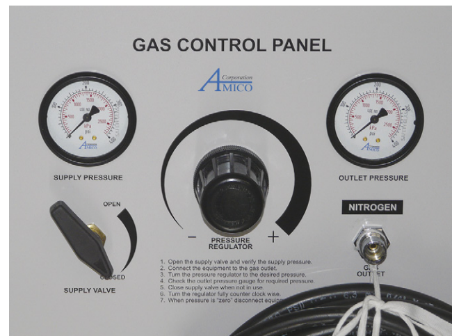
FIGURE 1-20 ■ An operating room control panel for nitrogen. The outlet pressure of nitrogen can be controlled by the variable pressure regulator. In this manner, the exact pressure can be set to meet the demands of the piece of equipment being powered.
