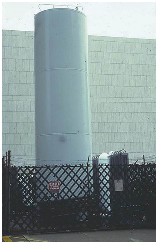
FIGURE 1-13 ■ A typical bulk-storage vessel for liquid oxygen.
