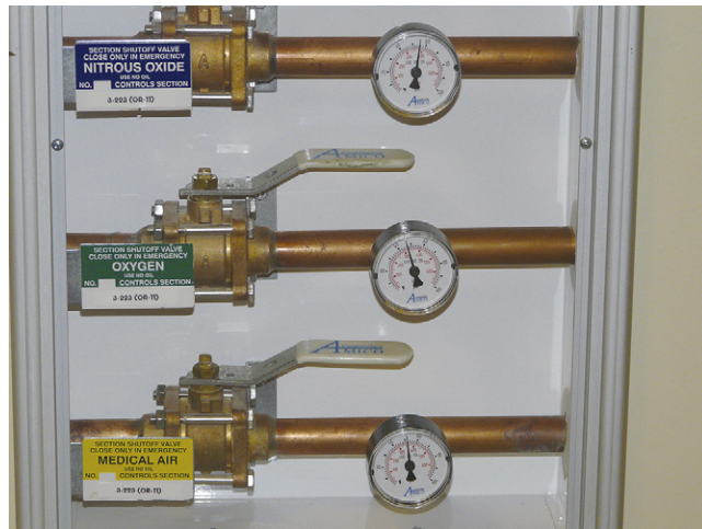
FIGURE 1-22 ■ Typical shut-off valves for the gases supplied in operating rooms (ORs). Each gas must have its own shut-off valve, and a separate set of valves must be present for each OR.
