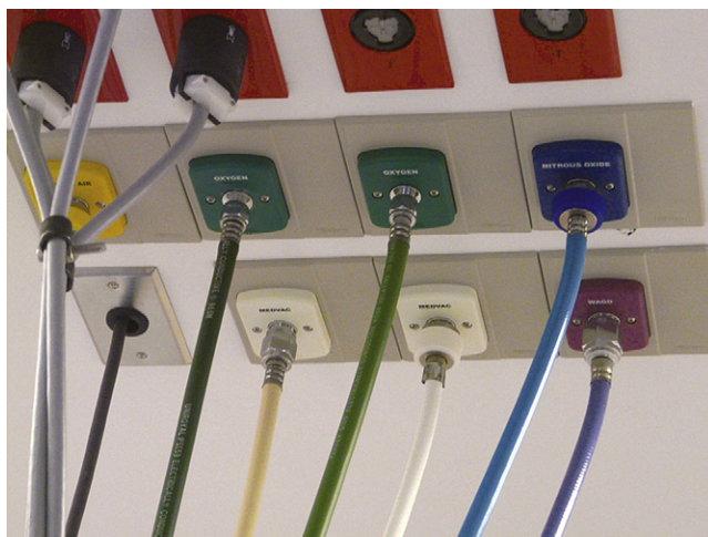
FIGURE 1-26 ■ Freestanding ceiling hose drops in an operating room. Note the proximal ends of the hoses (nearest to the ceiling) have diameter index safety system connections. The distal ends (nearest to the anesthesia machine) have quick-coupler connections (see Fig. 1-23).
