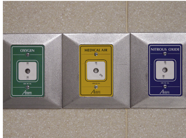
FIGURE 1-24 ■ Wall connections for oxygen, air, and nitrous oxide in a safety-keyed quick-connect system. The GE Healthcare (Waukesha, WI) quick-connect system is shown, in which each gas is assigned two specific pins with corresponding inlet holes within the circumference of the circle. In this manner, the connection is made gas specific.
