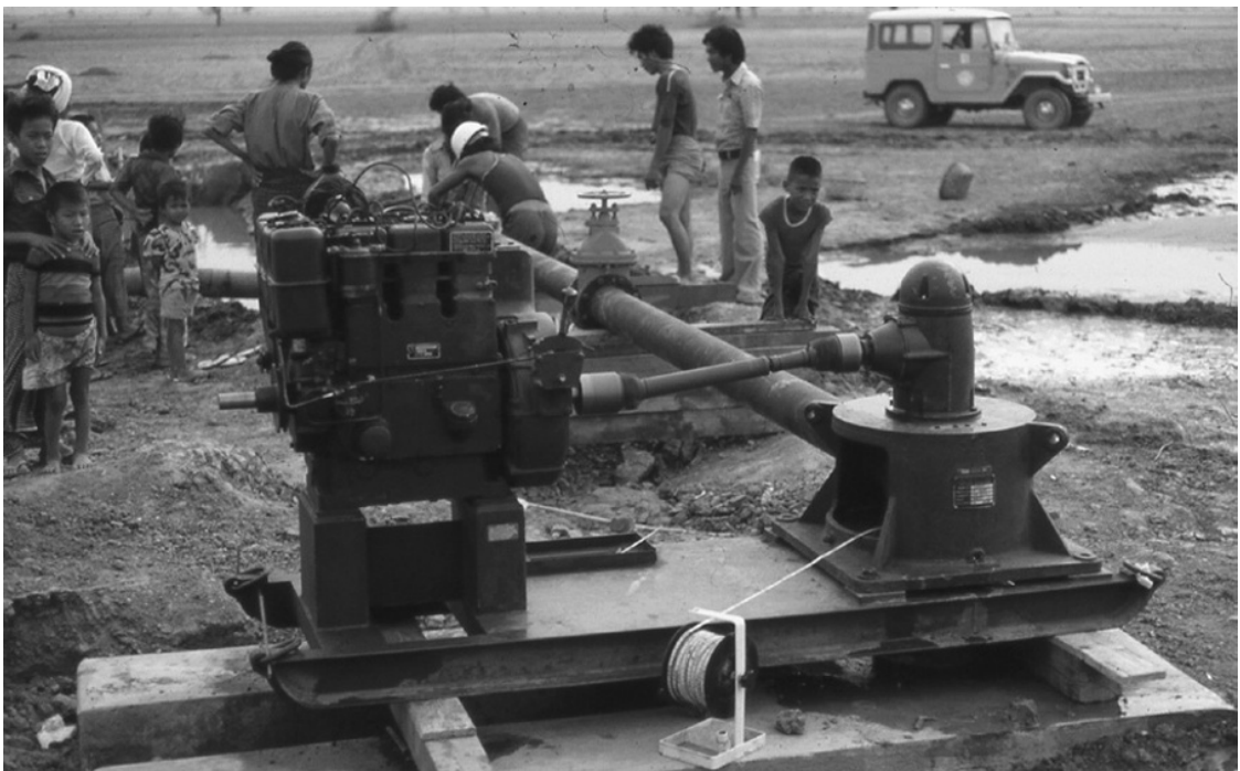
Figure 3.21 A vertical turbine pump installed in an irrigation well in Myanmar. The diesel prime mover is connected to the pump by a right-angle gear drive. This pump installation is temporary, for the purpose of a pumping test. Photo by Bruce Misstear
