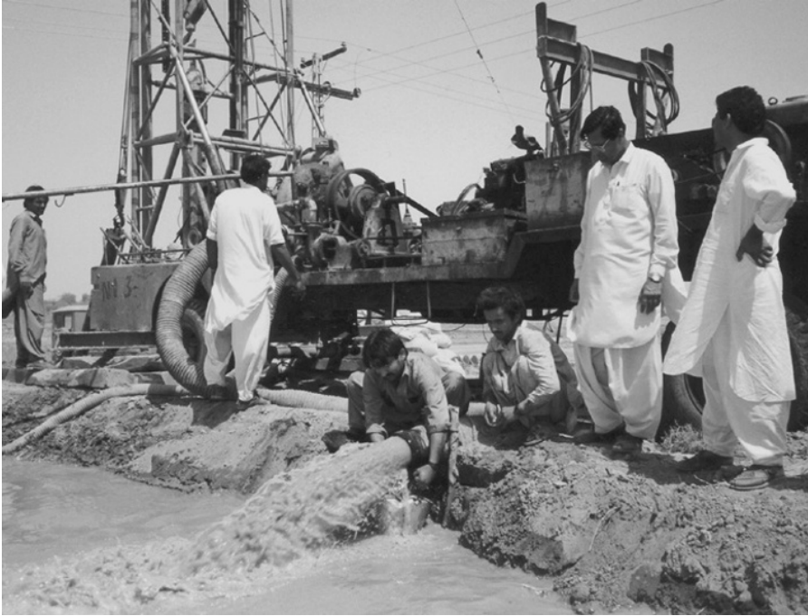
Figure 6.7 Collecting formation samples from reverse circulation drilling in Sind province, Pakistan. Photo by Bruce Misstear
