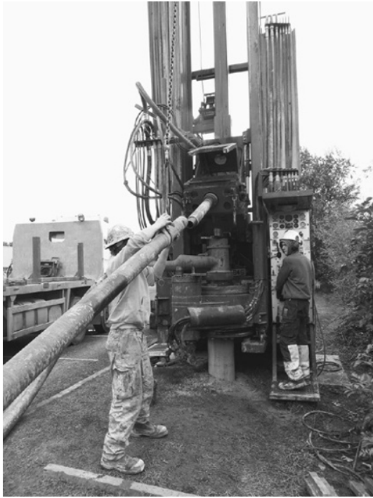
Figure 5.17 Dual rotary rig, Ireland. A drill rod is being added to the top drive whilst jaws from the lower drive clasp the outer casing. Photo by Bruce Misstear
