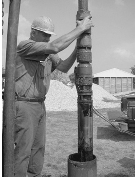
Figure 9.10 Biofouled submersible pump removed from a carbonate aquifer well, Ohio, United States. Iron oxide deposits are visible on the pump bowls, while a black iron sulphide slime can be seen on the motor. Reproduced by permission of Stuart Smith, Smith-Comeskey Ground Water Science LLC
