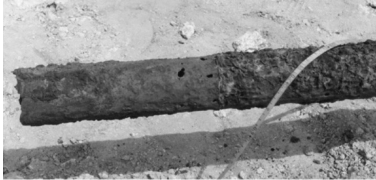
Figure 9.4 Corroded pump rising main removed from a well in an alluvial aquifer, Oman. The rising main exhibits both pitted corrosion and iron oxide incrustation. Photo by Bruce Misstear
