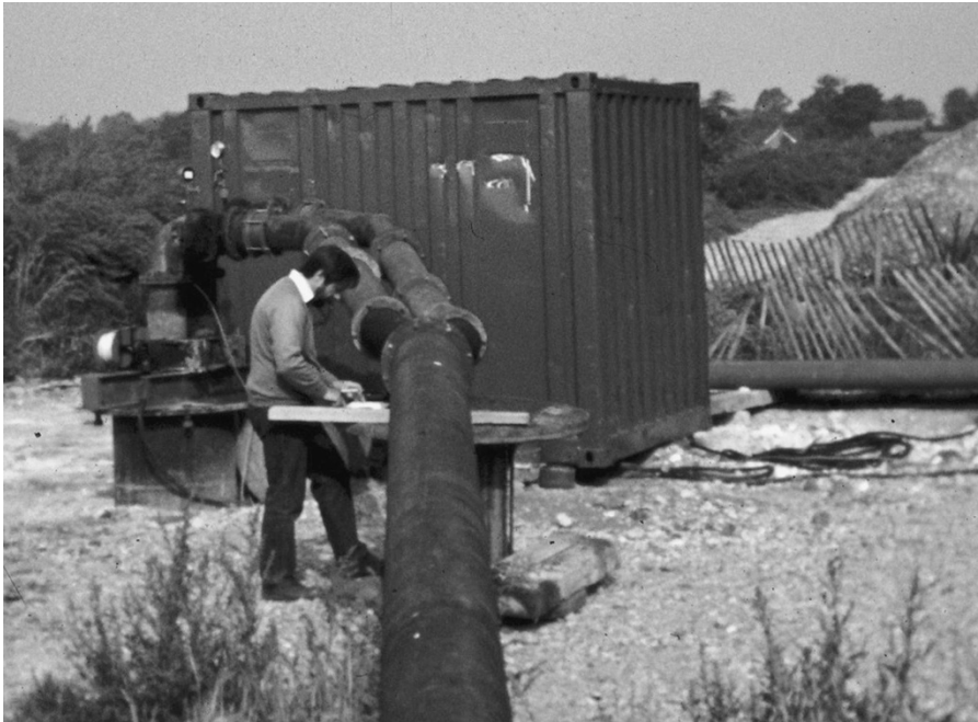
Figure 7.3 Two large submersible pumps (and two rising mains) are installed for test pumping of this abstraction well in the Chalk aquifer at Gatehampton, southern England. The pumped water is discharged to the River Thames. Photo by David Banks
