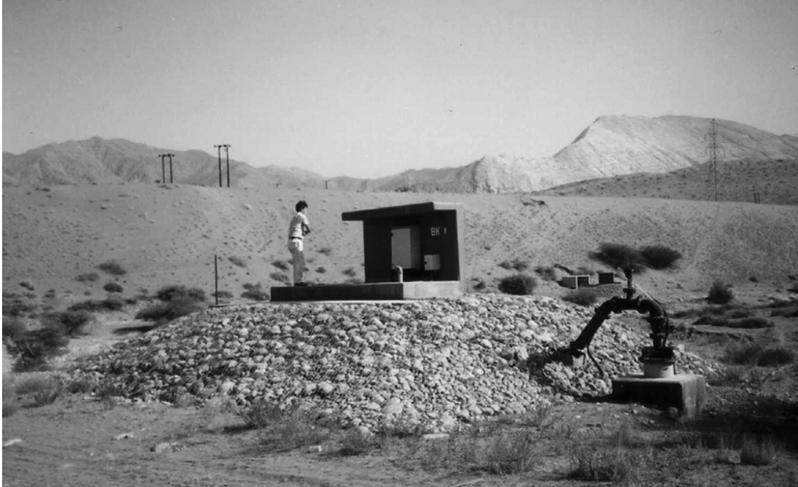
Figure 5.30 A wellhead arrangement at a wadi site in northern Oman which is susceptible to occasional flooding. The valves and other pipework are located in a gabion-protected concrete chamber, whilst the electric control panel is on top of the chamber (where the hydrogeologist is standing) to keep it as high as practicable above anticipated flood levels. The well, which has a watertight cover, is outside the chamber, so as to be accessible for maintenance. Photo by Bruce Misstear
