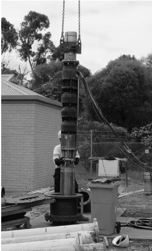
Figure 3.22 An electric submersible pump being installed in a well in Western Australia. Photo by Bruce Misstear
