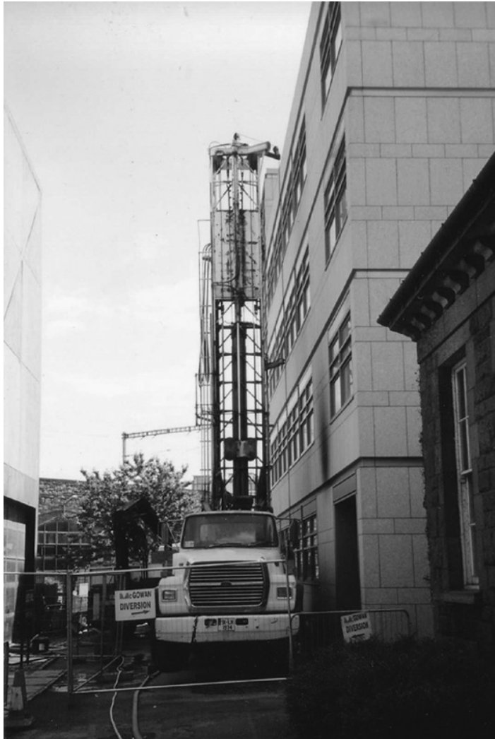
Figure 1.5 Drilling rig being set up for constructing a well in a gravel aquifer used as a source of geothermal energy, Dublin, Ireland. Photo by Bruce Misstear
