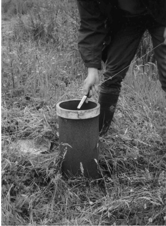
Figure 2.21 Small water level monitoring unit (incorporating pressure transducer, power source and data logger) being installed in an observation borehole in County Monaghan, Ireland. Photo by Bruce Misstear
