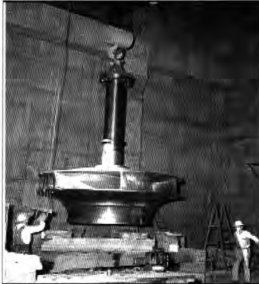
Figure 12.24. Large impeller and shaft assembly (U.S. Bureau of Reclamation).
