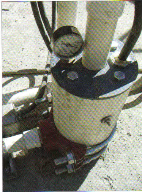
Figure 15.19. A vacuum-tight well head (Moretrench).
