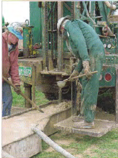
Figure 3.12. Drilling professionals using a small sieve to catch samples of cuttings from a mud rotary drill rig.
