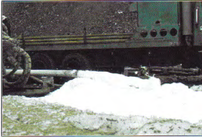
Figure 8.26. A properly run foam exits the blooey line in a uniform steady flow, and has a consistency similar to shaving cream (© 2005 Baroid, a Halliburton PSL).
