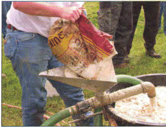
Figure 8.17. The drilling fluid additives are being mixed through a venturi mixer, which is the most effective way to mix drilling-fluid additives and insure proper hydration (© 2005 Baroid, a Halliburton PSL).
