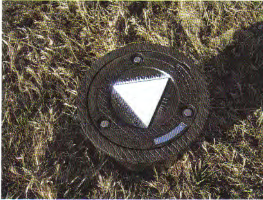
Figure 14.8. Well vault (Site Services, Inc.)
