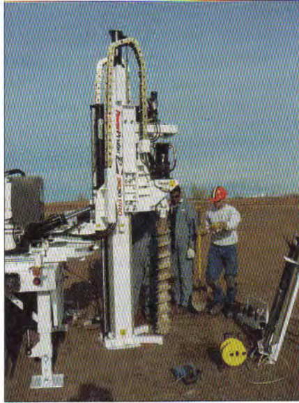
Figure 3.7. Continuous flight auger used to drill nominal 6-in (152-mm) borehole and complete 2-in (51-mm) well (AMS, Inc.).
