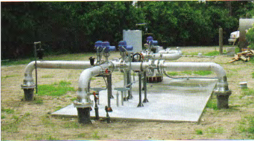
Figure 15.4. Kiawah Island Utility, Kiawah Island, SC (U.S.A.), with PVC casing and SS316 wellhead.
