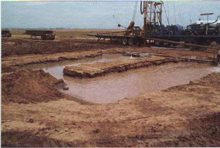
Figure 8.15. The mud pit often is comprised of two reservoirs, to be more effective in settling cuttings (Clear Creek Associates).
