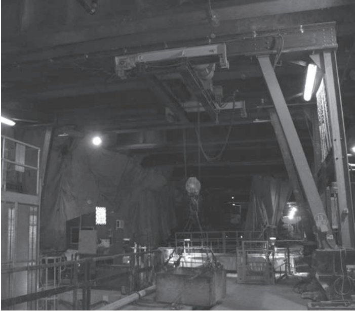
Figure 11.8 Gantry Crane above an Internal Shaft
