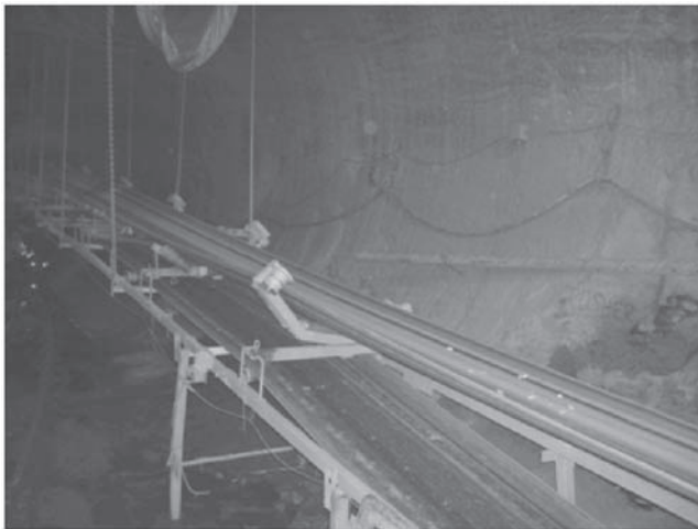
Figure 9.11 Conveyor for Underground Muck Transport
