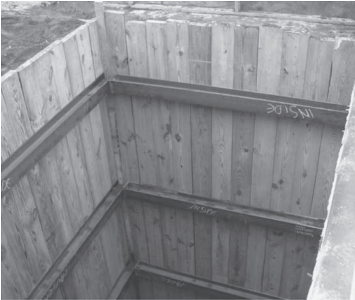
Figure 11.9 Vertical Wood Sheeting Sunk 20 ft to Access Top of Hospital Tunnel at North Shore University Hospital (Courtesy of Macro Enterprises, Ltd.)
