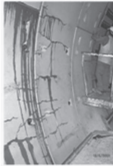
Figure 17.3 Leakage through Cracks in Segments
