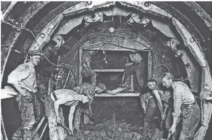
Figure 4.9 Workers Using the Greathead Shield to Construct a segment of the London Underground, London, England (Courtesy of The London Transport Museum)
