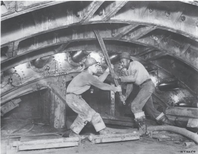
Figure 17.2 Tightening Segment Bolts in the Midtown Tunnel (Photographer Michael Bobco for Somach Photo Service, Feb. 26, 1939. Courtesy of MTA Bridges and Tunnels Special Archive)
