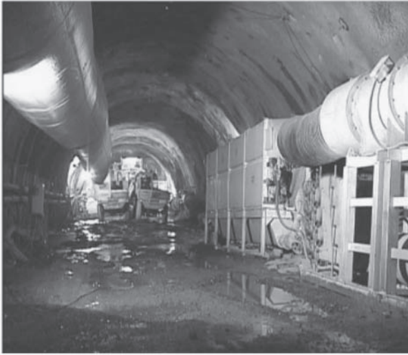
Figure 16.2 Tunnel Air Filter
