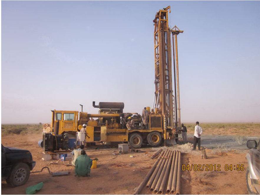
Fig. 18 Drilling in Somaliland. Alluvial and terrace deposits often cover the main karstic aquifer systems
