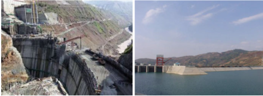
Fig. 7 The Trunk Dam construction (left) and the reservoir (right) on the Karst areas
