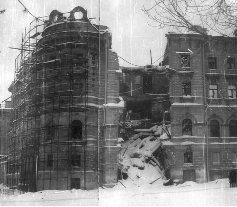
Fig. 4.4 Collapse of a building in the historical part of Kazan (1977)
