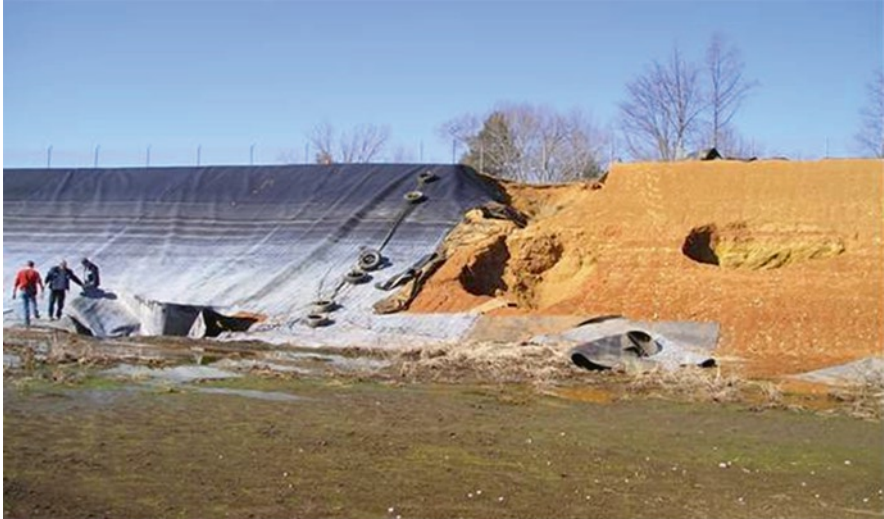
Fig. 2.5 Sinkholes that occurred in a detention pond in Tennessee
