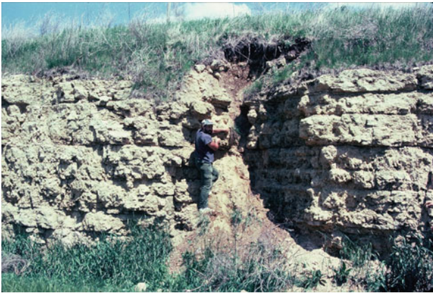
Fig. 6.11 Incipient sinkhole in road cut in the Platteville Formation, Iowa County. Photo provided by Michael J. Day
