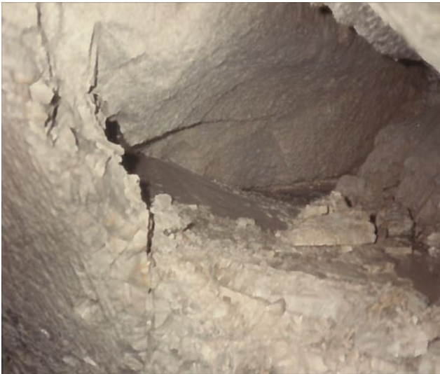
Fig. 6.8 Open void in the wall of 5.2 m diameter MMSD tunnel. Photo HU35-7, © 2020 MMSD records
