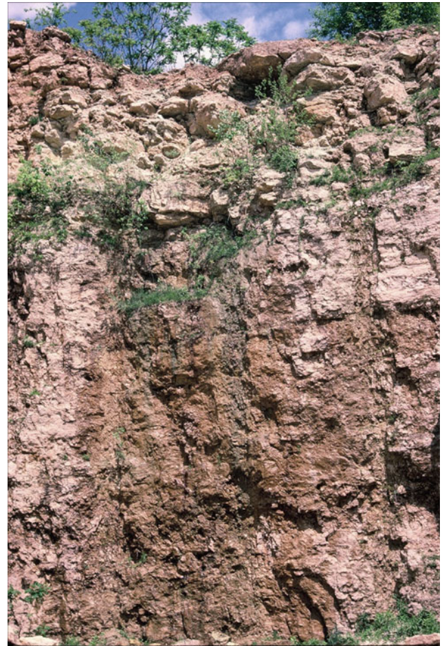
Fig. 6.12 Prairie du Chien quarry with incipient sinkhole, Vernon County. Photo by Michael J. Day
