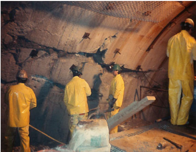
Fig. 6.9 Clean fractures in wall of 5.2 m diameter MMSD tunnel. Photo HU29-21, © 2020 MMSD records
