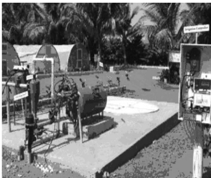
FIGURE 7 Fertilization and chemigation equipments.
