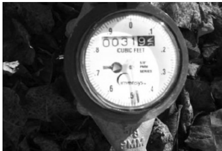
Flow meter to measure the volume of water applied.
