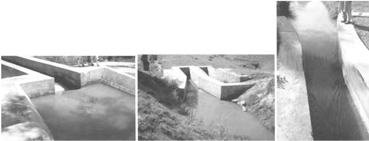
figure 7.16 Inlet transitions to siphon aqueducts on the Shamozaï Distributary, Upper Swat Canal. Compare the smooth flow in the elliptical transition on the right with the turbulence in the straight walled one, and the sudden head loss in the square-edged one
