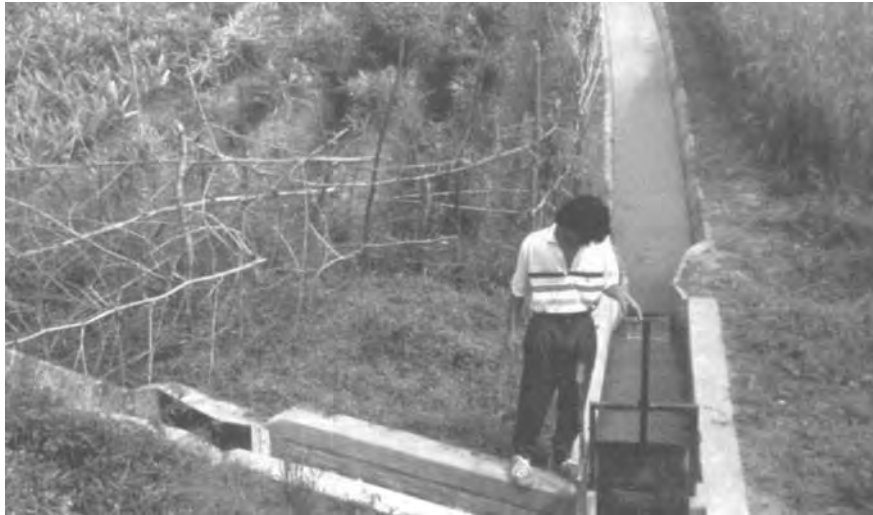
figure 7.3 Simple lift gates used for check and turnout, India. Note the cut-throat flumes, one in precast concrete and the other in steel. The crop is ginger
