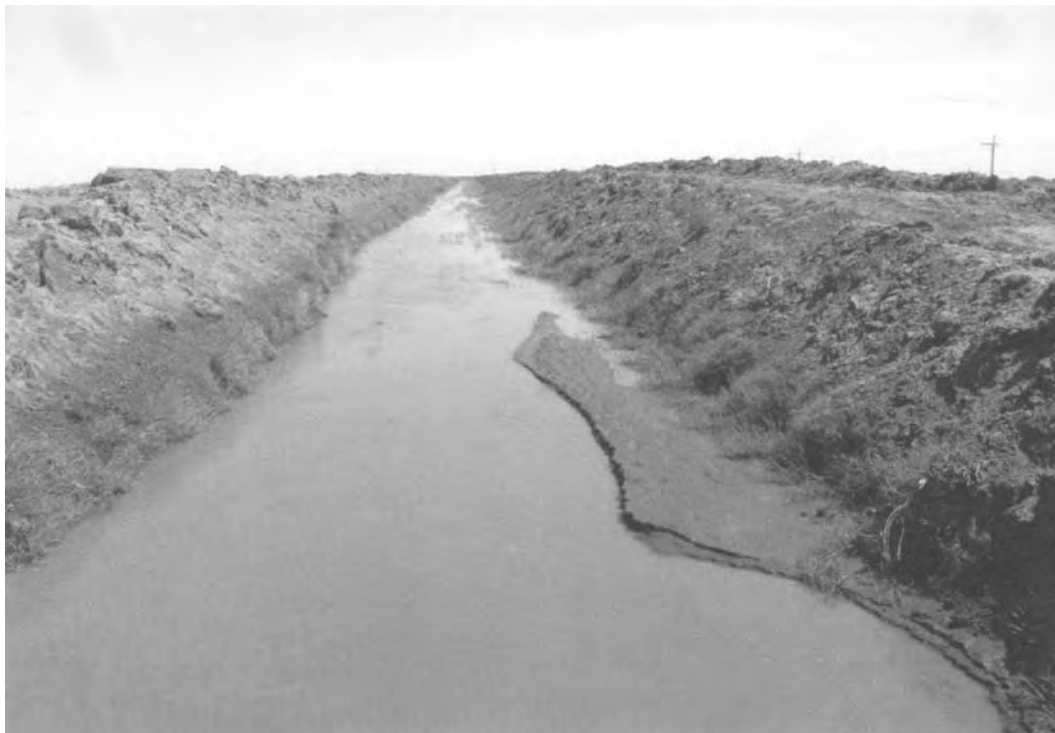
figure 4.6 Silt accumulating in a Gezira minor canal, Sudan. As the silt is dug out, the banks grow higher each year
