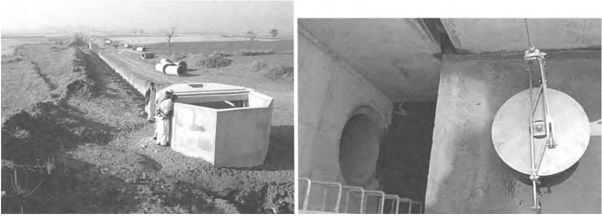
figure 8.9 Harris valve stands in Topi, Pakistan. These are very substantial structures, built to deter vandalism. These 24 inch diameter Harris valves are here arranged in pairs to handle the discharge of 1200 l/s
