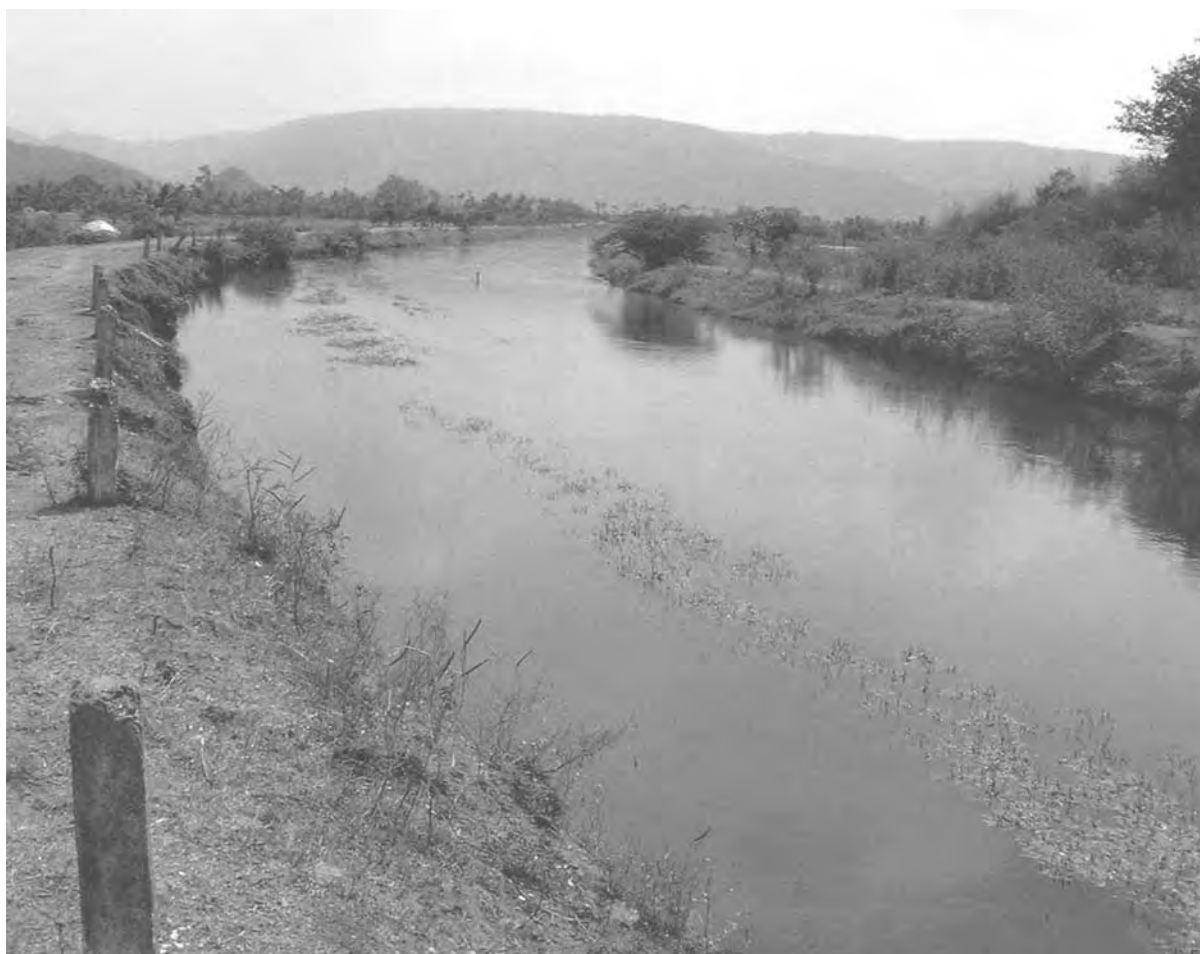
figure 11. 8 Heavy weed growth in clear water from a large reservoir. Yeleru Left Bank Canal, Andhra Pradesh
