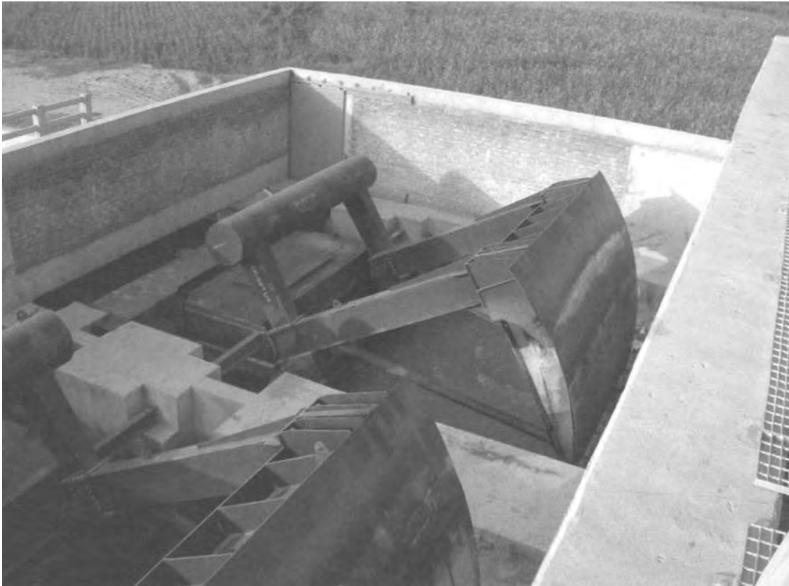
figure 4.3 Downstream control gates on the Pehur High Level Canal, Pakistan
