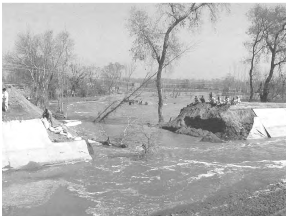
figure 11.1 The most likely time for a canal breach is during first filling after construction or, as in this case, after extensive remodelling with downstream control gates. (Maira Branch Canal, Pakistan. Photo by C. G. Swayne)
