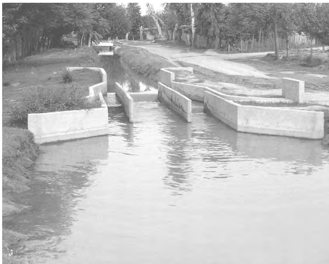
figure 7.7 Double trifurcator. The flow to each outlet is divided twice, to outlets on both sides of the canal
