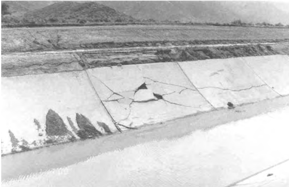
figure 11.6 Lining burst by external hydrostatic pressure from surface-water flooding
