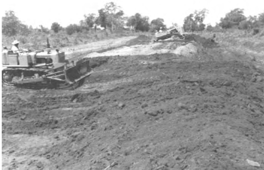
figure 9.14 How not to build a canal. Dozing up the banks without compaction, Sri Lanka
