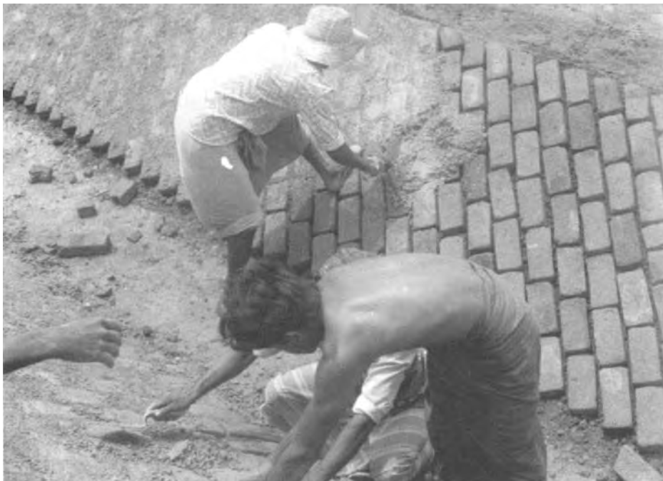
figure 9.4 Brick lining, Sri Lanka. Every joint is a potential source of leakage, but at least it's cheap
