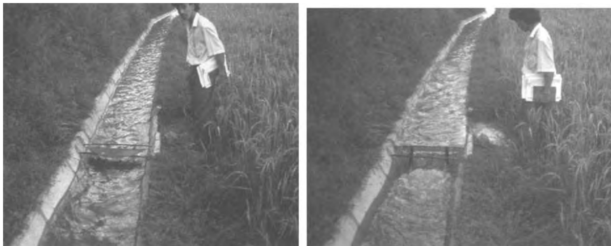
figure 7.11 Parabolic check plate, with field outlet closed at left, open at right
