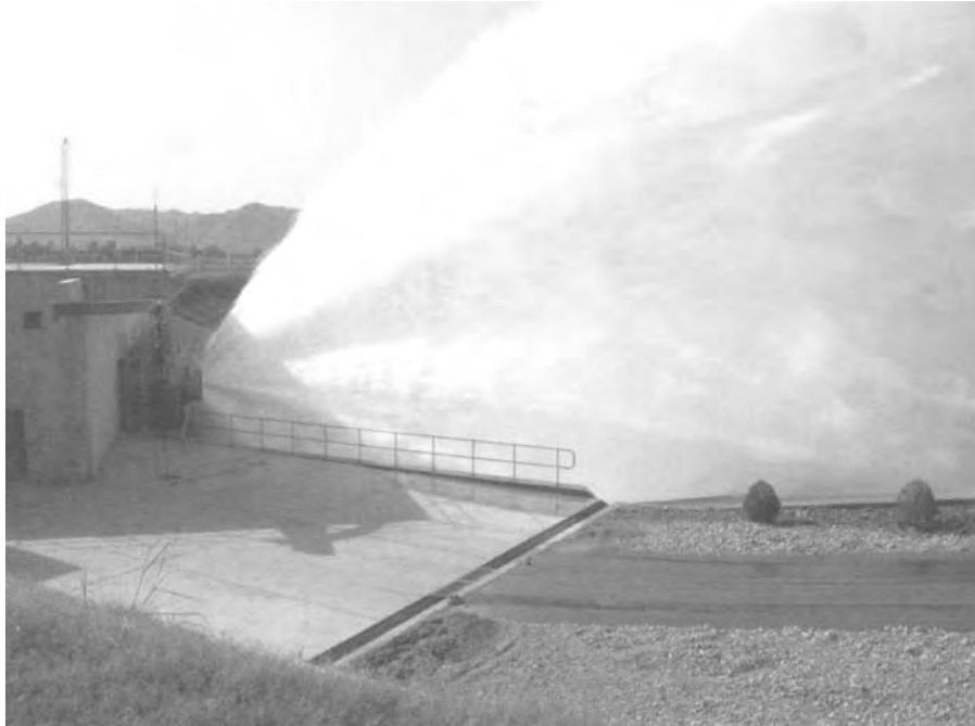
figure 4.9 SCADA-controlled outlet valves supply the Pehur High Level Canal
