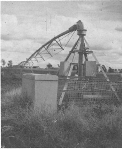
Figure 6.9 Pivot end of a centre-pivot irrigator. Electricity and water are delivered to the pivot point, then along the machine. This older style machine has medium pressure sprinklers mounted on the sprayline.
