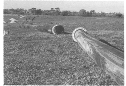
Figure 8.7 Flanges welded to pipes in the field ready for final positioning and bolting together (Courtesy: Vinidex Tubemakers P/L)
