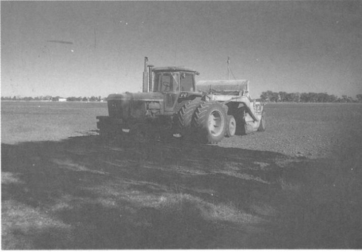
Figure 5.5 Earthmoving under way using a tractor drawn scraper. The operating height of this is adjusted in response to a laser signal. The mast on the machine carries the laser receiver; the laser emitter is mounted on a tower near the centre of the field.
