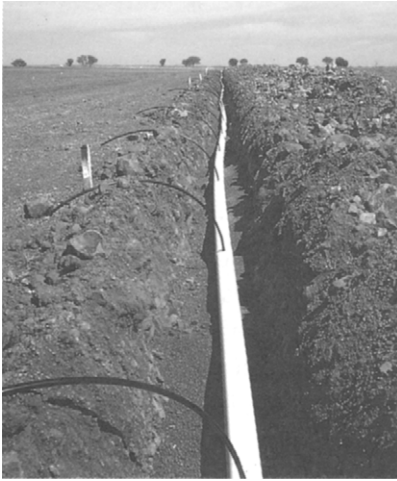
Figure 8.9 Installation of large bore PVC pipe. Trench width, bedding conditions, and backfilling technique should comply with manufacturers requirements. Rocky terrain such as this poses particular difficulties, as the pipe must be protected against rock contact
