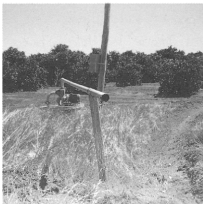
Figure 9.17 On flat terrain or where deep drains prevent the use of channels, drainage water may need to be pumped from a sump.
