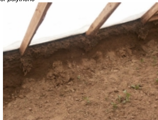
Picture 41 - Earth exfoliation due to joists resting directly on the earth
