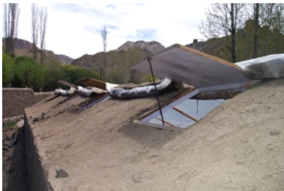
Picture 47 - Top view of roof ventilator
