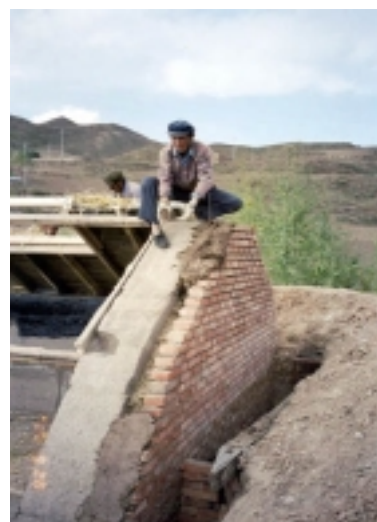
Picture 18 - Construction of the outer wall with baked bricks and the inner wall with stabilised rammed earth in Qinghai
