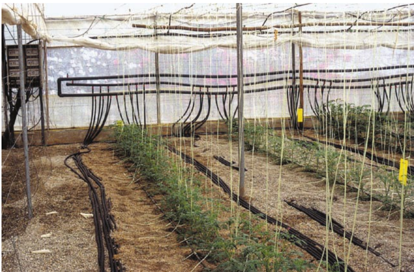
Photo 7.5. Heat distribution pipes of a low-temperature heating system.
