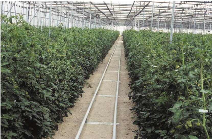
Photo 7.4. Metallic heating pipes that are also used as rails for the movement of trolleys and mechanized elements.
