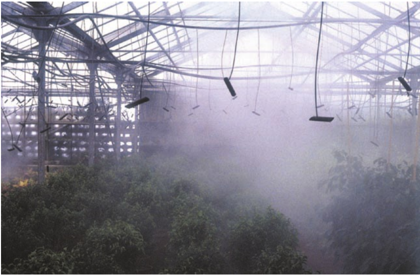
Photo 8.5. Greenhouse water fogging.
