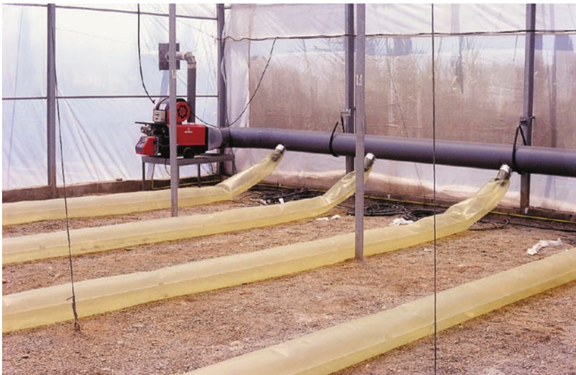
Photo 7.3. Indirect combustion hot air generator and flexible plastic air distribution pipes.
