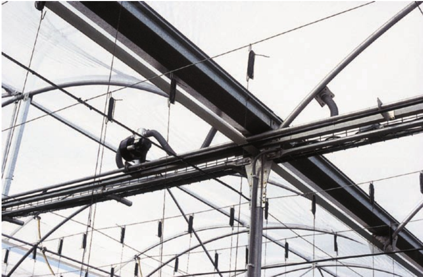
Photo 7.1. Greenhouses made of inflated double plastic film improve the insulation conditions but require special fixing systems.
