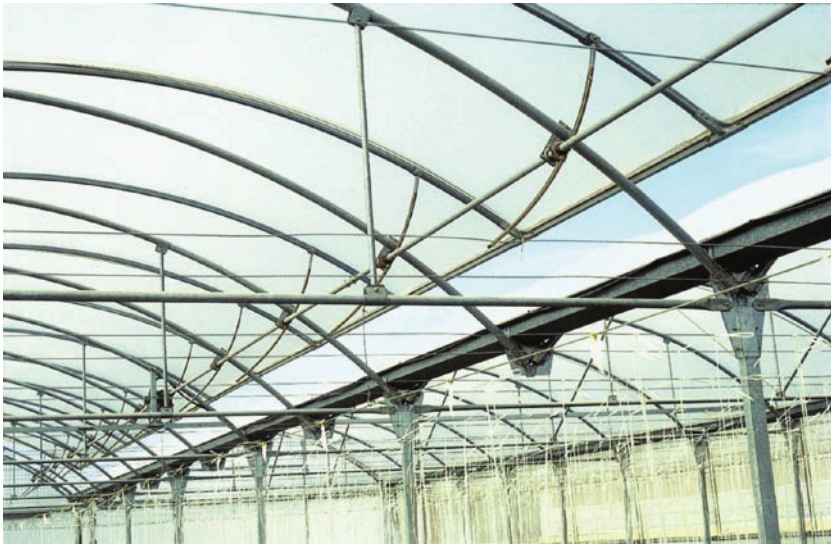
Photo 8.1. The vents must be mechanized to facilitate their automatic opening and closing.
