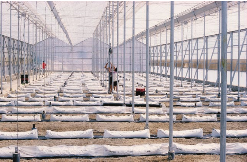
Photo 14.3. Improved high roof slope low-cost parral-type greenhouse, of metallic structure (steel and wire).
