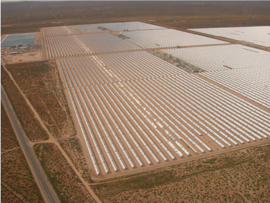
Fig. 1.2 Aerial view showing portions of SEGS III-VII plants located at Kramer Junction, California. Photograph by Alan Radecki Akradecki
