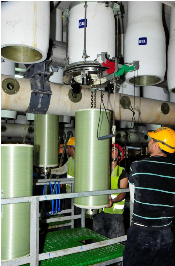
FIGURE 8.5 Sorek SWRO plant loading of 16-inch element.
