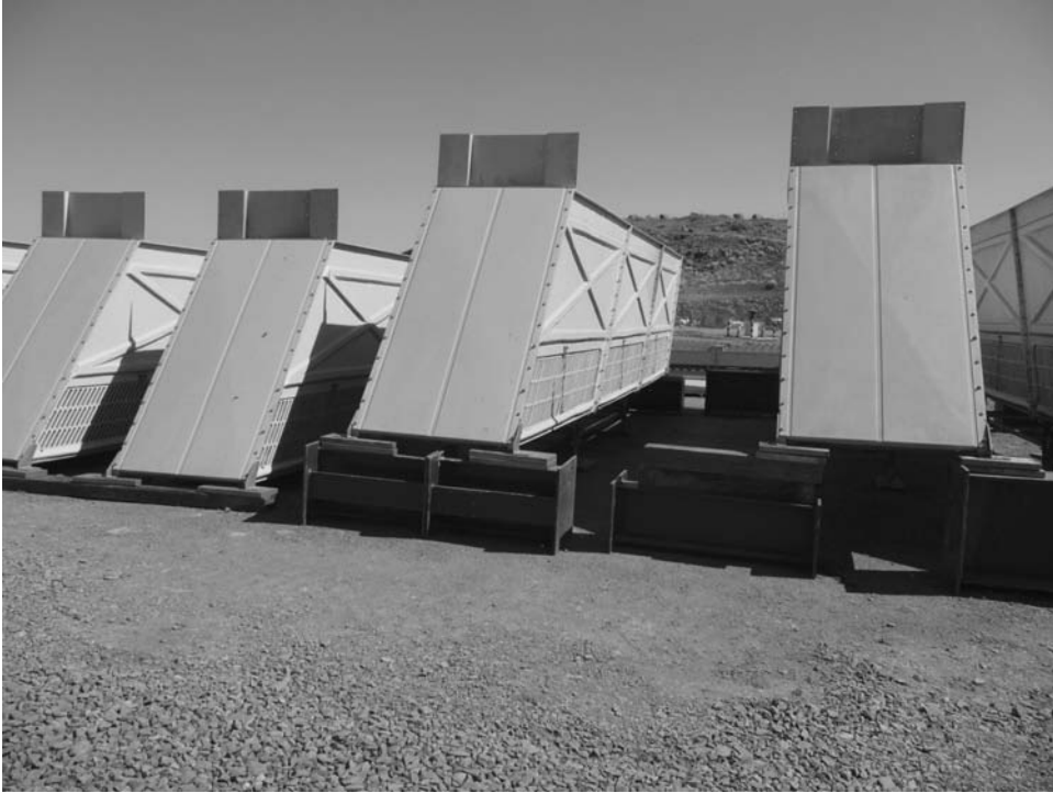
FIGURE 10.3 Lamella modules—Cape Preston desalination plant, Australia.
