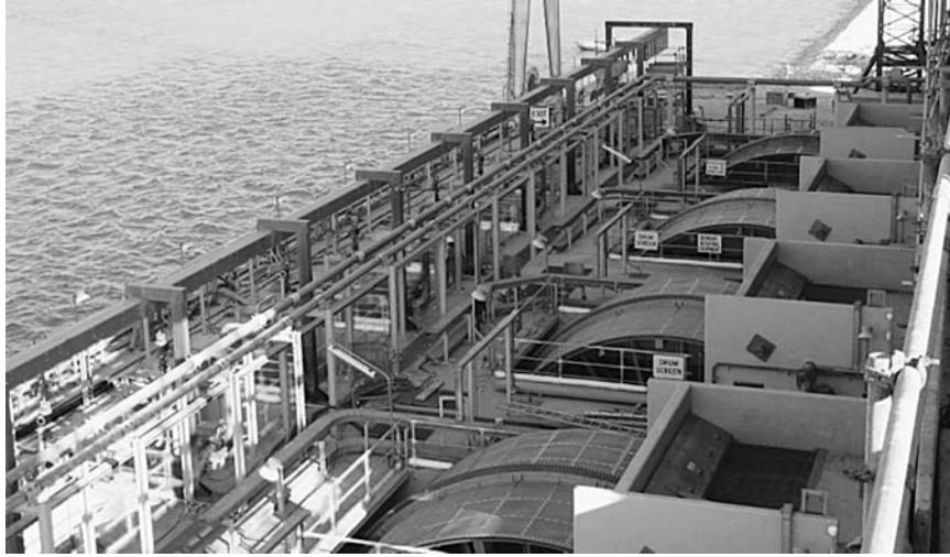
FIGURE 5.2 Fine intake screens.
