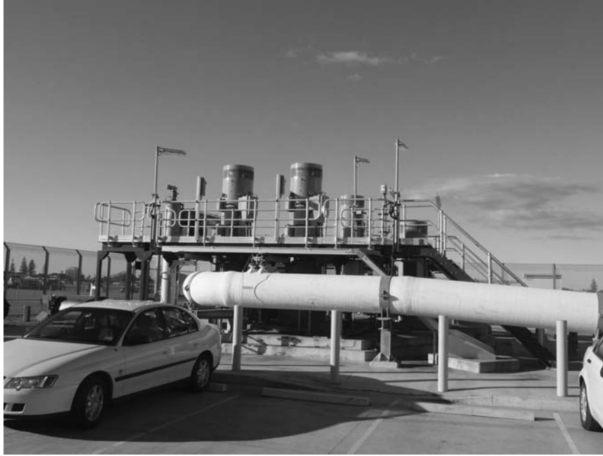
FIGURE 7.1 Wet-well intake pump station of Gold Coast Desalination Plant.
