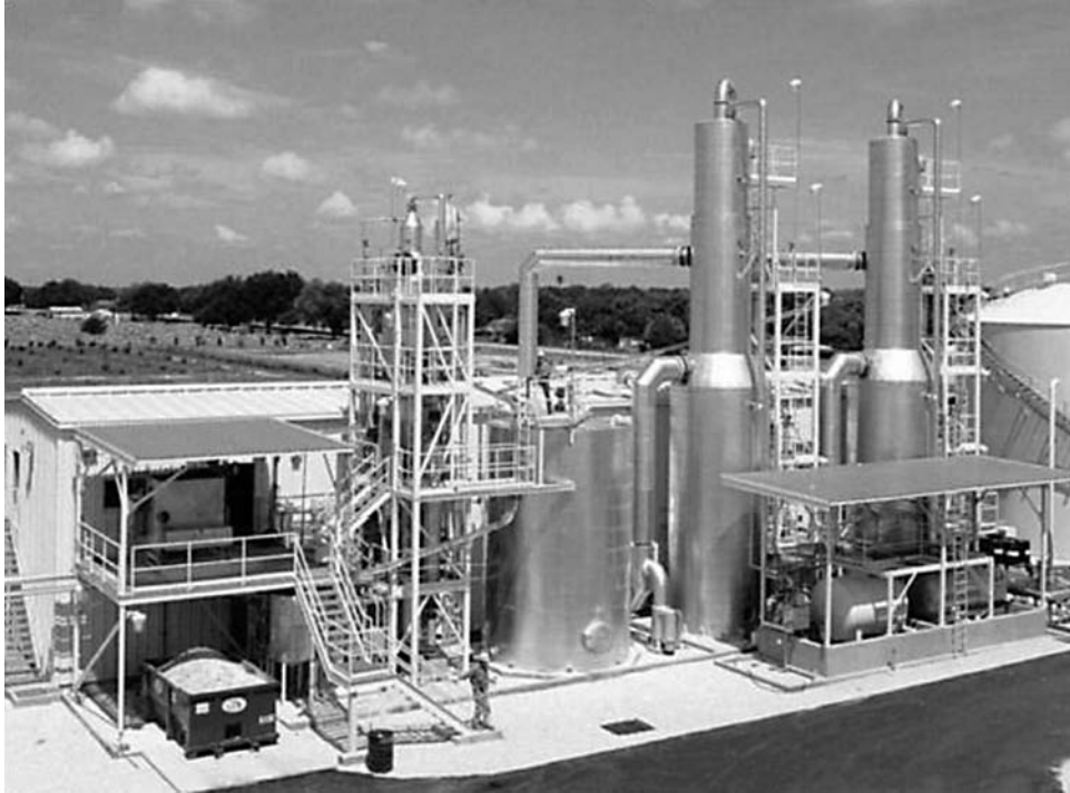
FIGURE 16.51 1000 m 3 /day (0.26 mgd) evaporator-crystallizer.
