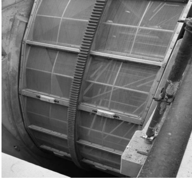
FIGURE 8.5 Drum screen of the Sydney Desalination Plant.
