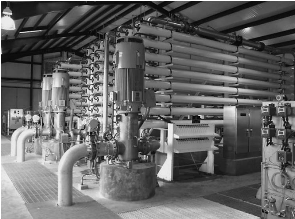
FIGURE 14.6 Vertical turbine high-pressure BWRO pumps.
