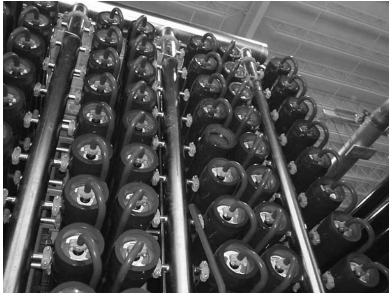
FIGURE 14.14 Permeate manifolds of Tampa Bay plant RO train.
