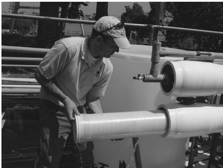
FIGURE 3.13 Unloading an RO membrane element from a pressure vessel.
