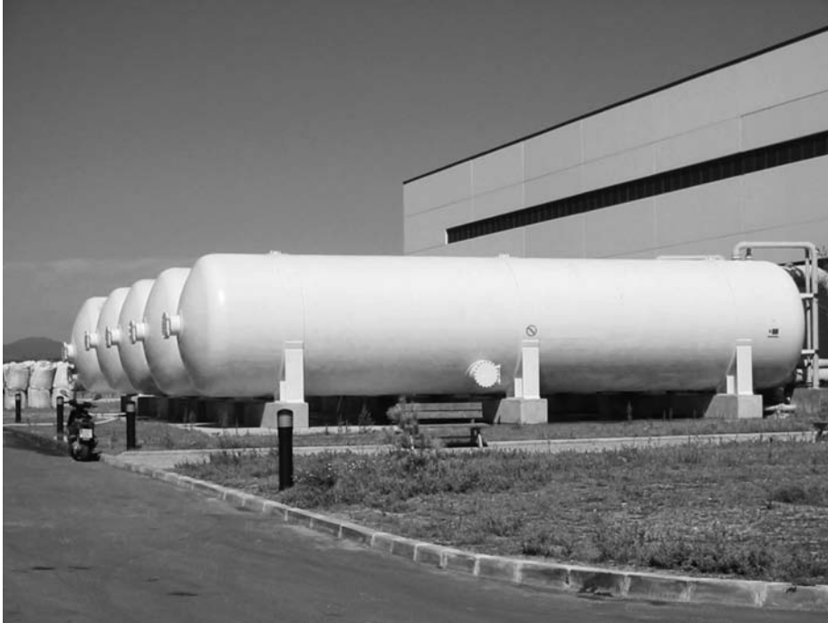
FIGURE 11.5 Horizontal pretreatment pressure filters.
