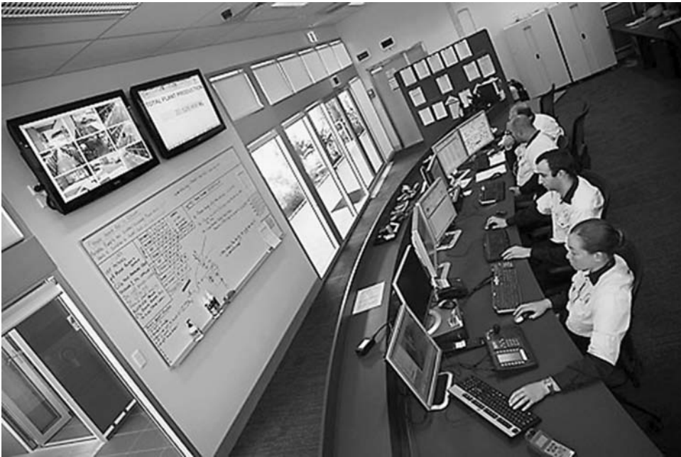
FIGURE 14.26 Central control room of Gold Coast SWRO plant, Australia.
