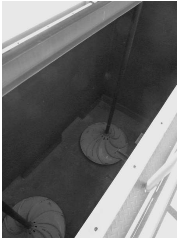
FIGURE 9.2 Flash mixers in coagulation tank.
