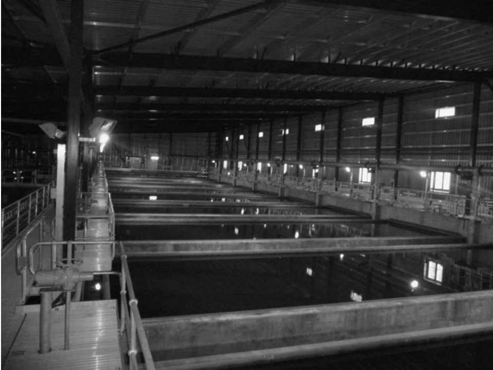
FIGURE 11.2 Single-stage gravity filters at the Gold Coast SWRO desalination plant, Australia.
