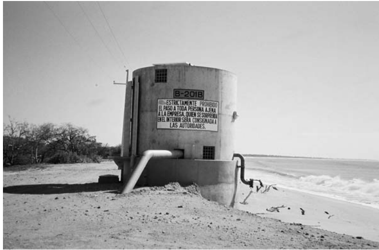
FIGURE 5.7 Radial intake well of a large seawater desalination plant.
