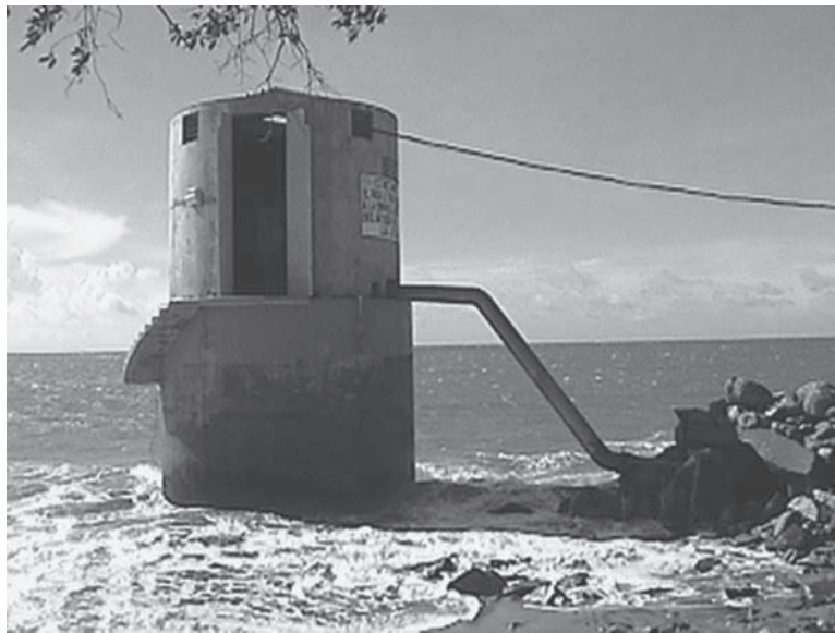
FIGURE 4.2 Seawater intake well exposed to beach erosion.
