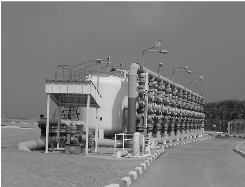
FIGURE 11.4 Vertical pretreatment pressure filters.
