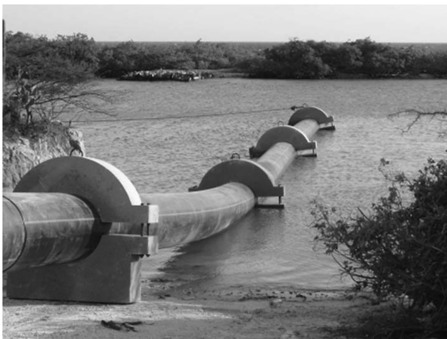
FIGURE 16.4 Outfall discharge pipeline supported on concrete blocks.
