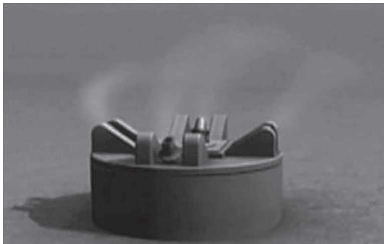
FIGURE 16.6 Sydney water SWRO diffuser structure.
