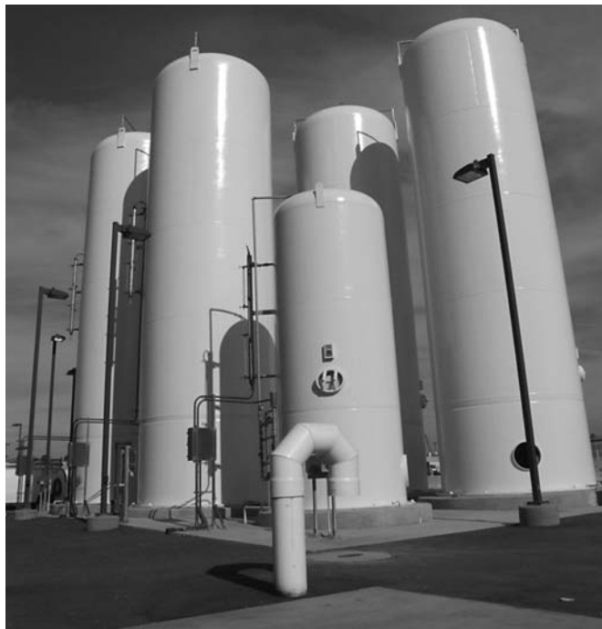
FIGURE 15.4 Carbon dioxide storage tanks.
