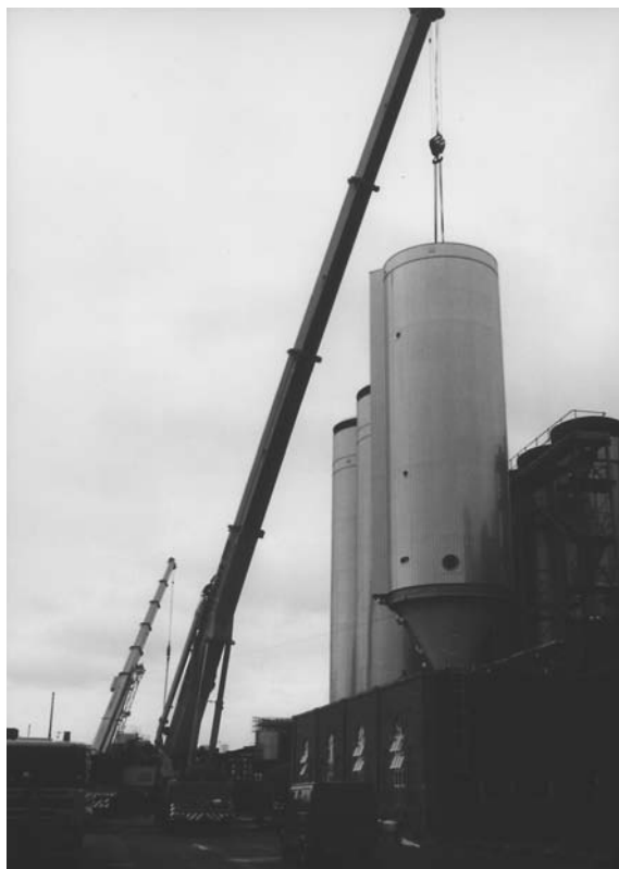
Fig. 5.13 Delivery (a), lifting (b) and installation (c) of new CCVs to Bass Brewers Burton Brewery (kindly supplied by Colin Turton, Bass Brewers).
