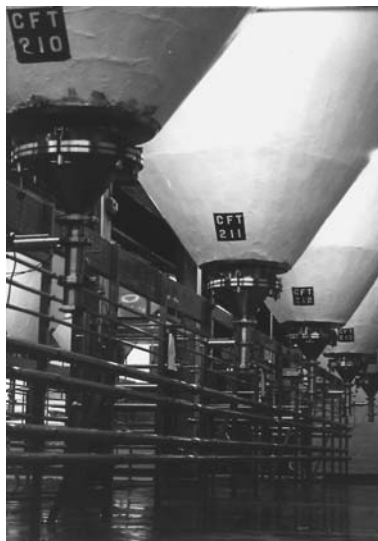
Fig. 5.15 CCV cones and associated mains (kindly supplied by Maxine Bellfield of Vaux Breweries).
