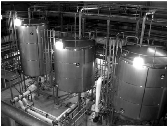
Figure 10.4 Tanks used in a brewery Cleaning-In-Place (CIP) system. Left to right are the prerinse storage tank, the caustic tank and the CIP return tank.
