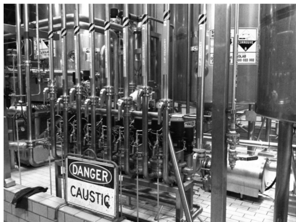
Figure 10.3 Valve manifold with hygienic mix-proof valves used in a Cleaning-In-Place system.
