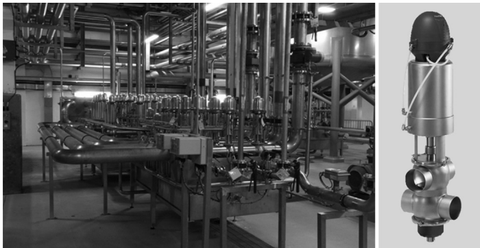
Figure 10.2 Mix-proof valves and valve array commonly used next to a chain of fermenters to hygienically control the transfer of beer and the Cleaning-In-Place cleaning fluid.
